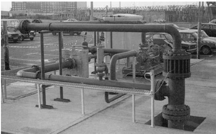
4.33 Southampton geothermal well head, brine pump and filter (reproduced by courtesy of Southampton Geothermal Heating Company).
