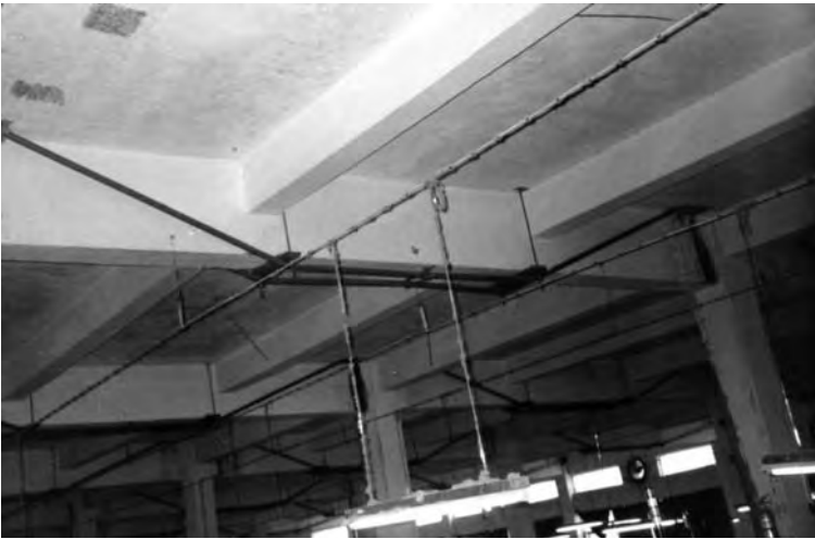
Figure 9.15 A floor structure experiencing excessive vibration then stiffened using profiled post-tensioned cables (courtesy of Professor Jida Zhao, China Academy of Building Research, China).
