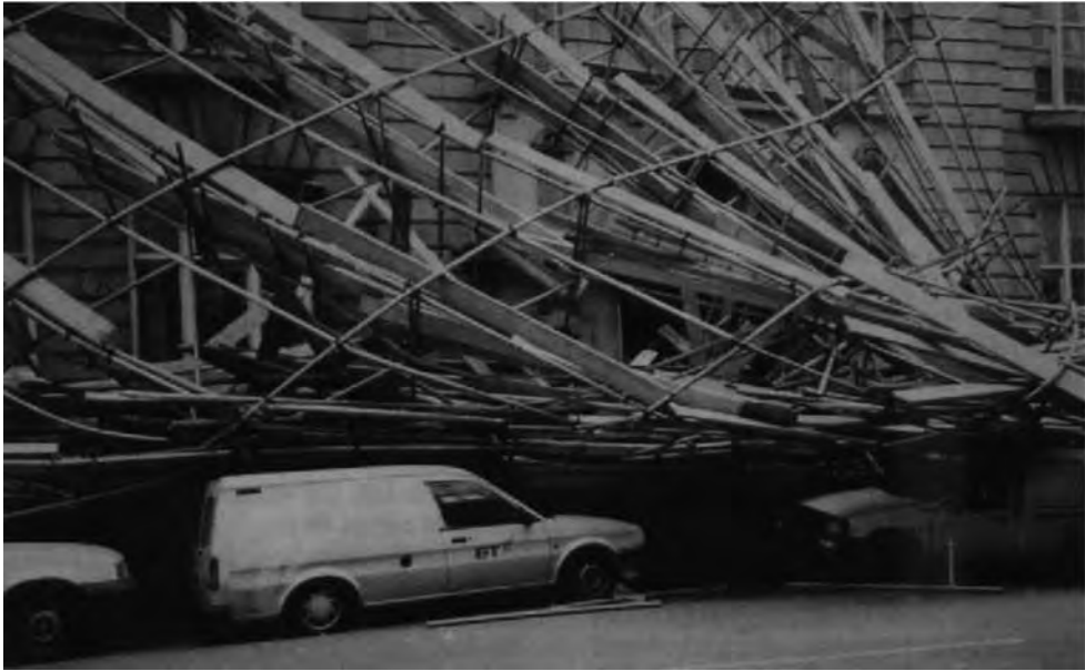
Figure 8.9 Collapse of a scaffolding structure (courtesy of Mr J. Anderson).
