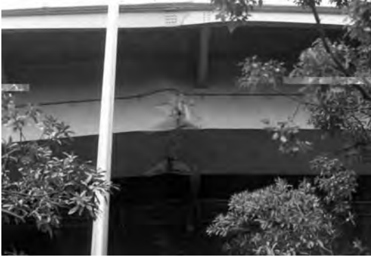
Figure 10.10 Buckling of a box girder (courtesy of Dr A. Mann, Jacobs).
