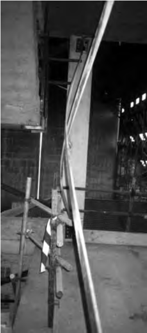
(b) Buckling of two bracing members in a building
