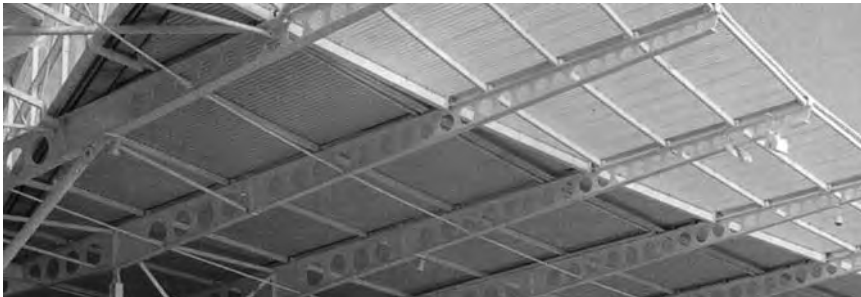
Figure 10.11 Additional supports provided to prevent lateral torsional buckling (courtesy of Westok Ltd).
