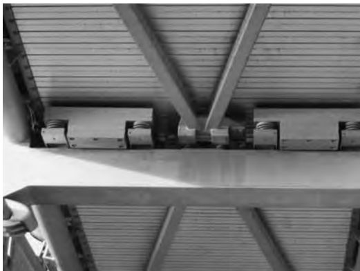
Figure 18.11 Two tuned mass dampers under the deck of the London Millennium Footbridge.
