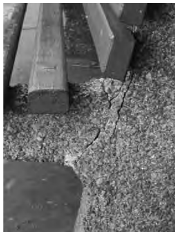
(b) Cracks at the end of the cantilever
