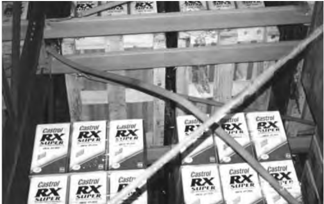
(a) Buckling of a bracing member in a storage rack (courtesy of Dr A. Mann, Jacobs)
