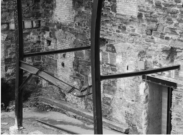
Fig. 6.1 Lateral torsional beam buckling exaggerated by fire.
