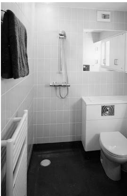
Figure 4.27 A modern shower installation with the waste water outlet in the floor
