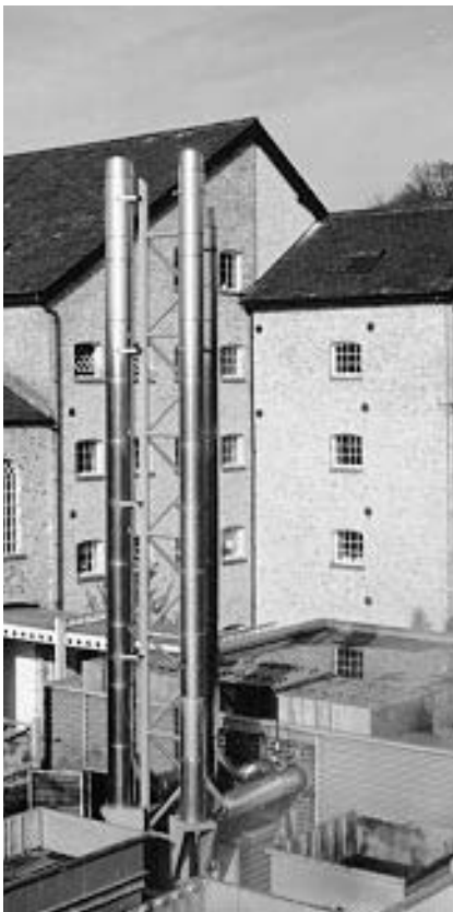
Figure 2.29 Multiple flues from a large installation supported from a common tubular framework
