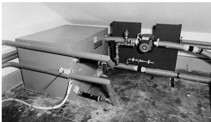
Figure 2.53 Heat pump installation in the Integer House on the BRE site, drawing energy from 50 m underground
