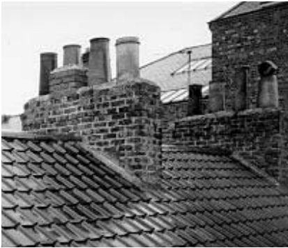
Figure 2.18 Eight different pots on these two chimneys provide evidence of past problems. When a pot of the same height as its neighbours was not available, a rather crude ad hoc solution was employed. The stacks are flaunching with a mortar fillet instead of flashed, and no DPC is evident
