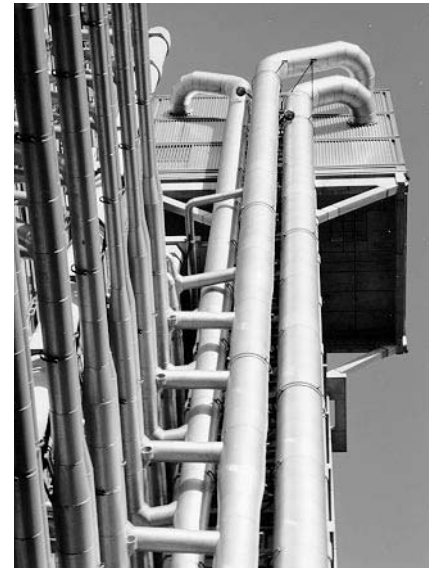
Figure 0.28 Services installations, the Lloyds Building, London
