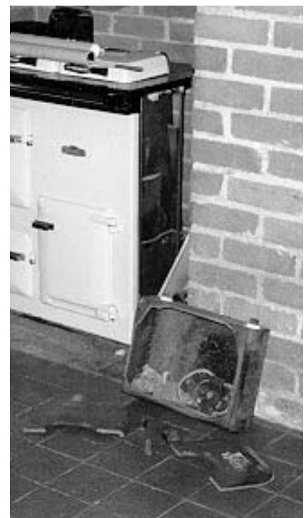
Figure 2.40 This boiler unit, having been catastrophically damaged, has been removed for diagnosis and replacement
