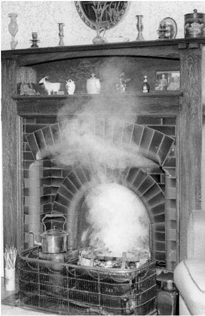
Figure 2.13 A problem which has plagued householders from time to time through the ages. If the fireplace and flue do not conform to the rules first formulated by Count Rumford, and summarised in Chapter 0, down-draught can cause reversal of the smoke flow
