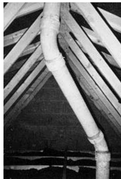
Figure 2.31 An example of an unsupported heavy asbestos cement flue pipe discovered by BRE site investigators in the roof space of a newly built house in the mid-1980s
