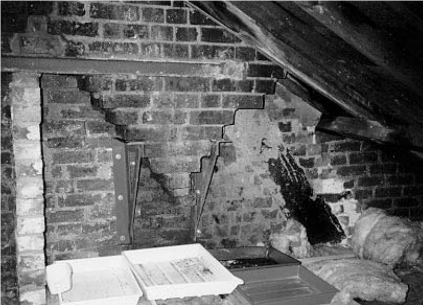
Figure 2.21 The flue and chimney breast below this roof space have been removed, and new steel brackets now provide additional support to the masonry near the foot of the corbel. The raking line of the old flue can be seen left and the brickwork now overhangs some one and a half bricks. The trays catch rainwater drips from the defective flashing above
