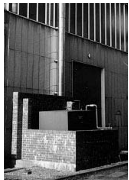
Figure 2.42 An oil storage tank with its surrounding brick wall, both to provide mechanical protection and to contain possible leakage after being holed by corrosion
