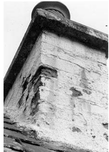
Figure 2.12 Although this stack had been rebuilt some ten years before the photograph was taken, some place (eg underburnt) bricks from the original stack had been reused. Although they may have been whole, they were insufficiently durable for the onerous conditions in the stack. Since they were already contaminated by the products of combustion, the problems recurred, showing up against the cement based paint
