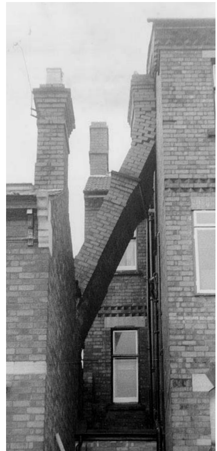
Figure 2.8 A collapsed stack. Incredibly, no bricks seem to have fallen to the ground (Photograph by permission of the Lincolnshire Echo)
