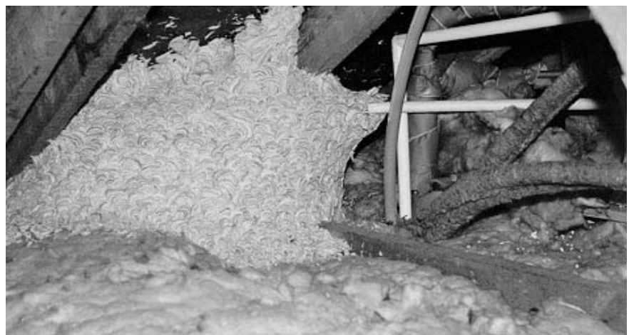
Figure 3.18 A large wasps nest built into the eaves of a 1960s house. Access was made by an overlarge hole for the warning pipe to the central heating header tank
