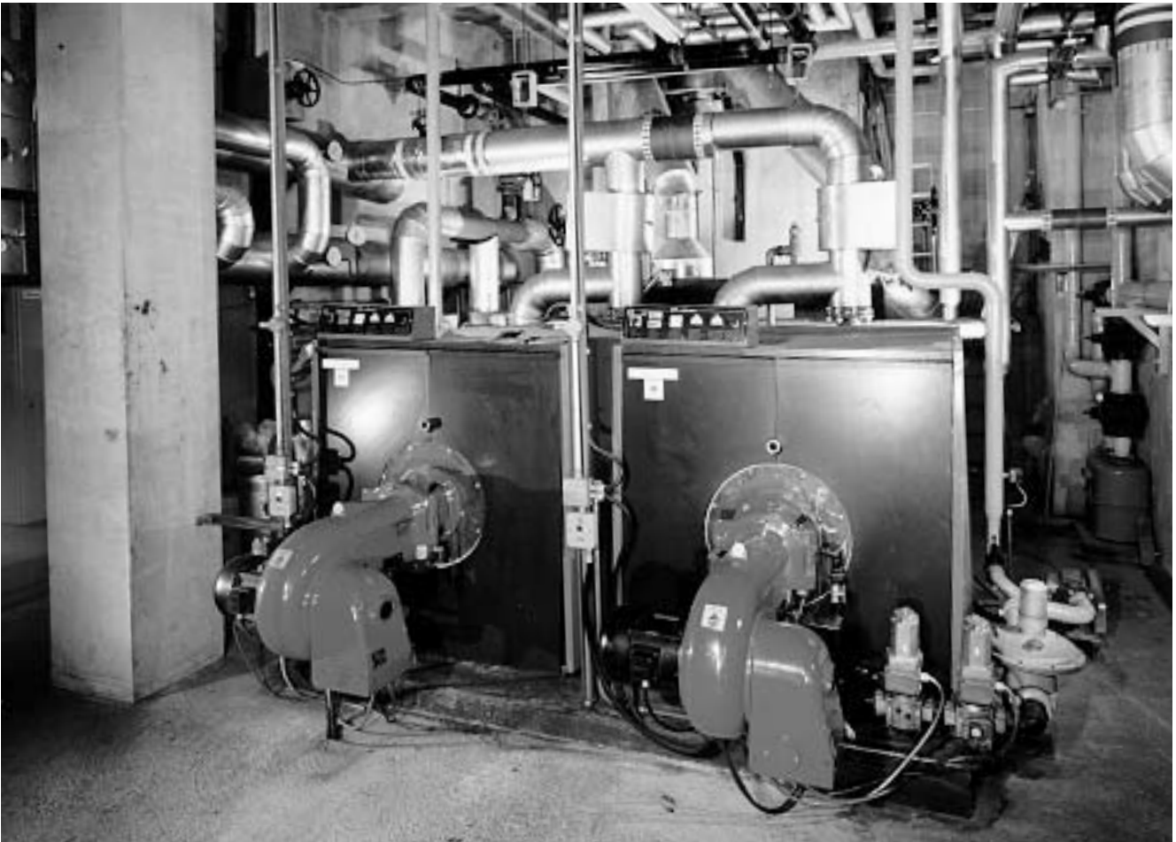
Figure 4.1 Part of the services installation for a large swimming pool
