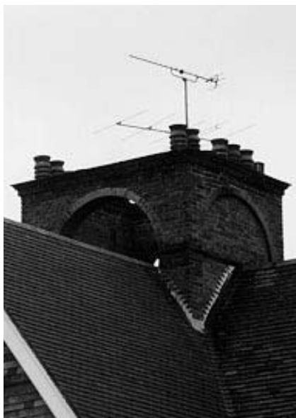
Figure 2.6 Multiple flues can take up a large proportion of the available space in a building. There are only around a dozen flues in this combined stack. The arches were introduced to provide mutual support
