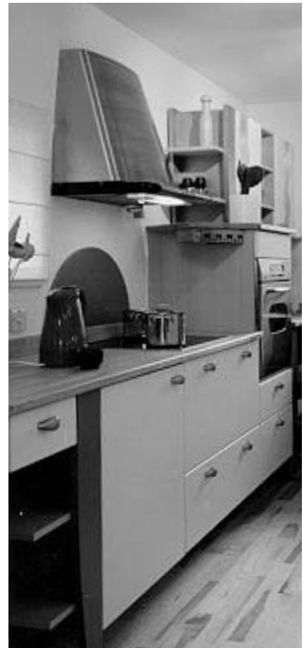
Figure 3.9 A cooker hood incorporated into a kitchen installation
