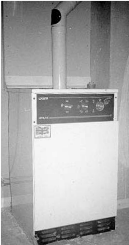
Figure 2.25 This large 1970s open flued boiler takes combustion air from the room in which it is situated, and therefore needs a permanently open vent to the external air. It is too heavy for wall mounting
