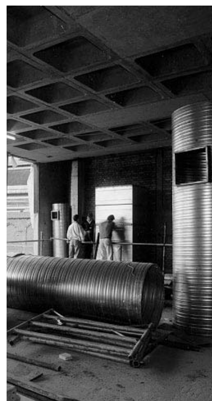
Figure 2.1 Space heating and cooling systems can take up a considerable amount of space. Here ducting, about 1 m in diameter, is being installed in a large building with complex servicing systems
