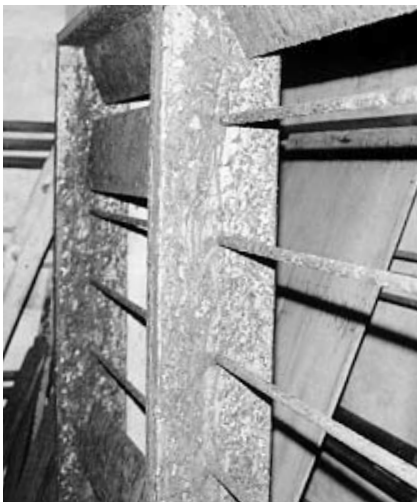
Figure 3.34 Baffles corroding on an austenitic stainless steel air handling grille
