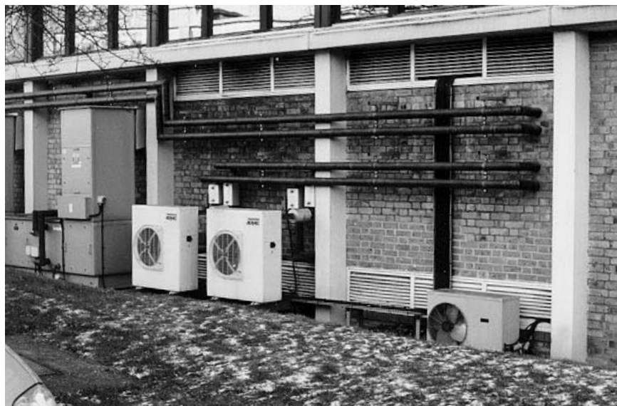
Figure 2.52 Air handling equipment retrofitted to laboratory accommodation. Although this equipment is easy to maintain, it cannot of course be placed in locations accessible by the public
