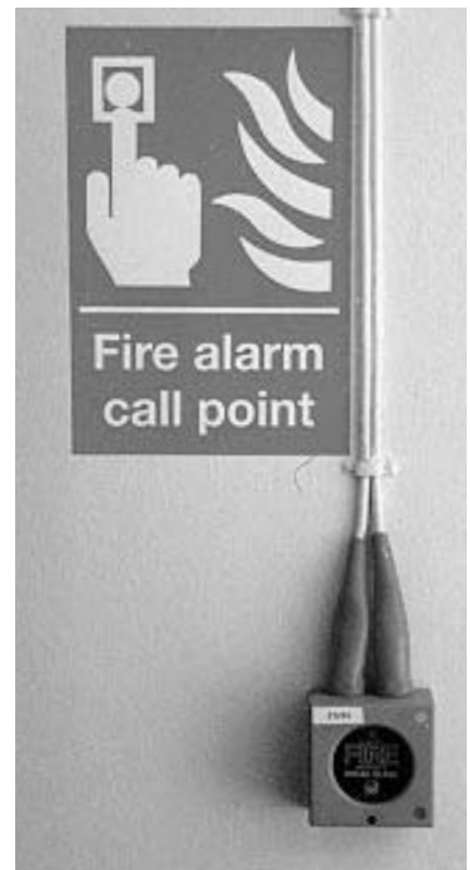
Figure 5.25 A manual switch to operate fire alarm systems
