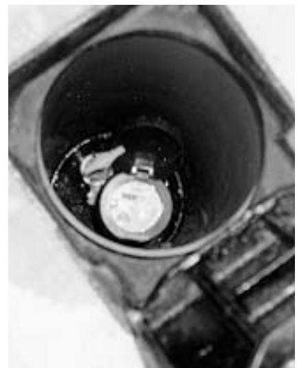
Figure 4.4 A typical water meter installation
