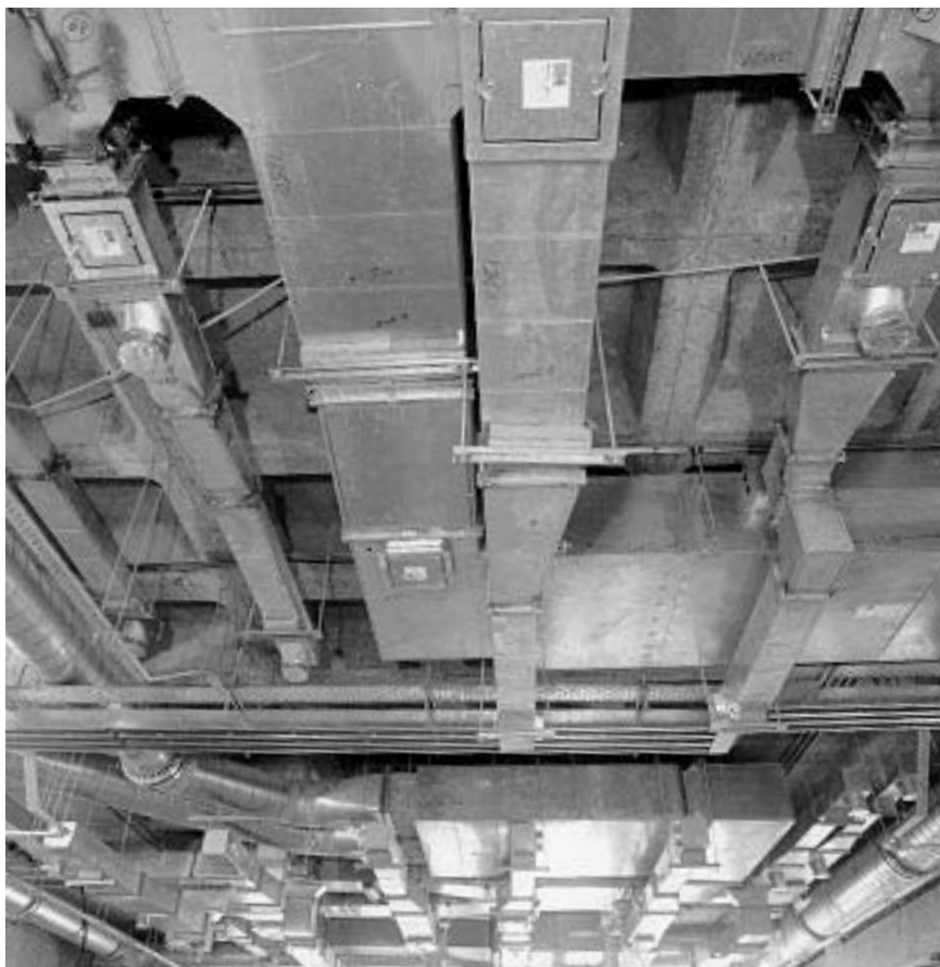
Figure 2.48 Air handling ducting installed in a very highly serviced building. The suspended ceiling has yet to be fixed
