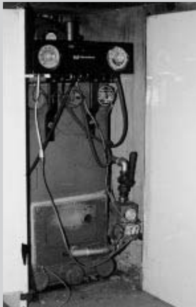
Figure 2.41 A cast iron, gas fired, fan flued 29 year old boiler still in use and still acceptably efficient as far as the owner was concerned
