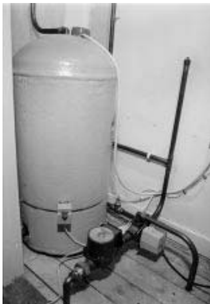
Figure 2.32 A small installation (in 1978) comprising a cylinder thermostat, a pump and a three-way motorised valve. The valve is controlled by both the cylinder thermostat and the room thermostat, and directs flow to whichever system is calling for heat. If both systems call, a shared position is selected, if neither call, the pump and boiler are switched off
