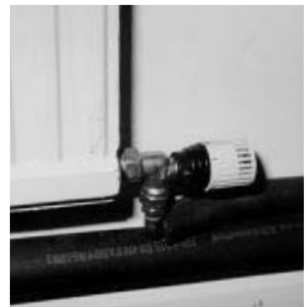
Figure 2.36 A thermostatic radiator valve (TRV) used to control the heat output from a single radiator by controlling the flow of hot water. The photograph dates from the mid-1980s
