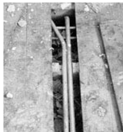
Figure 2.44 In this new installation in a refurbishment project, the uninsulated hot and cold water pipes are touching. Not only will the hot pipe be cooled but the cold pipe will be heated, leading to inefficiencies
