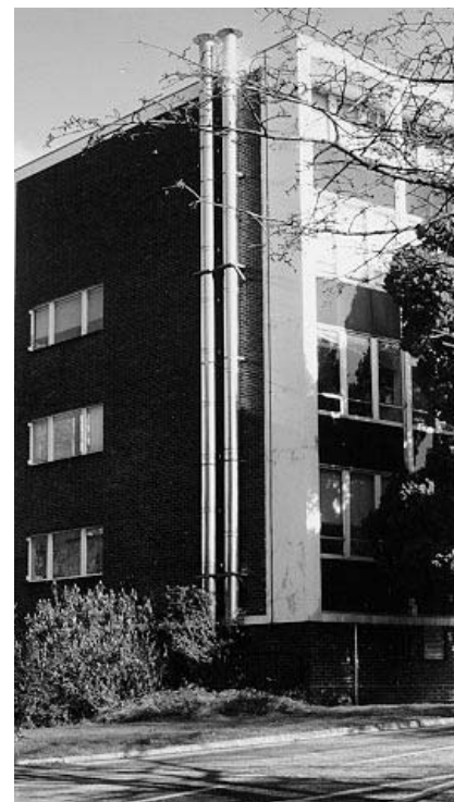
Figure 2.39 In this building on the BRE site, the existing radiator system was reused when new gas boilers replaced the mains distribution system. The stainless steel flues terminate in such a position that emissions are carried clear of opening windows
