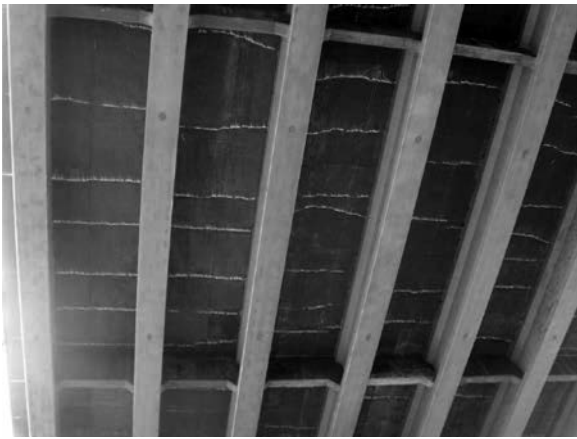
Fig. 3.4.3—Transverse cracking (from below).
