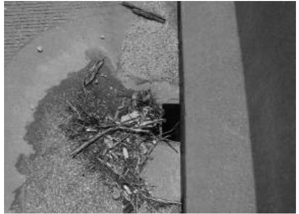
Fig. 3.6.3—Poor design and lack of maintenance permit debris to accumulate and block deck drains.
