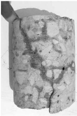
Fig. 6.1.8(b)—Horizontal and vertical cracking aligned with reinforcing bar in concrete sample extracted from a bridge deck.
