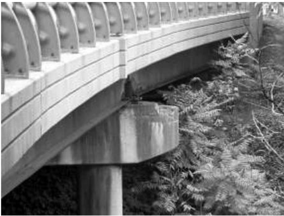
Fig. 3.6.1(b)—Water leakage through failed joint causes corrosion and deterioration of pier cap.
