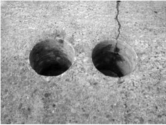
Fig. 6.1.8(a)—Vertical cracking in deck concrete aligned with reinforcing bar (right).
