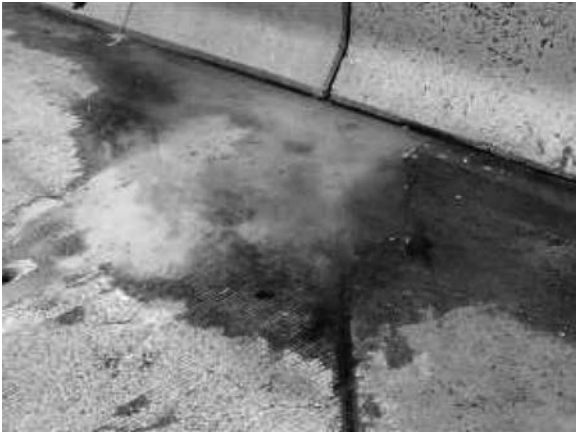
Fig. 3.6.1(a)—Poor deck drainage causes water to collect at joint.
