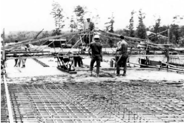
Fig. 6.2.5.1.1(b)—Close-up of longitudinal travel, longitudinal finish screed. Equipment is moving toward camera.
