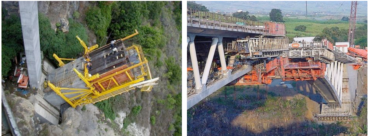
Fig. 7-31. Two cases of cantilever formwork with variable slope. Left: Arco de Los Tilos (Spain) Courtesy of Ferrovial-Agromán. Right: Bridge over the “bras de la Plaine”(Reunion Island). Courtesy of Bouygues Travaux Publics.
