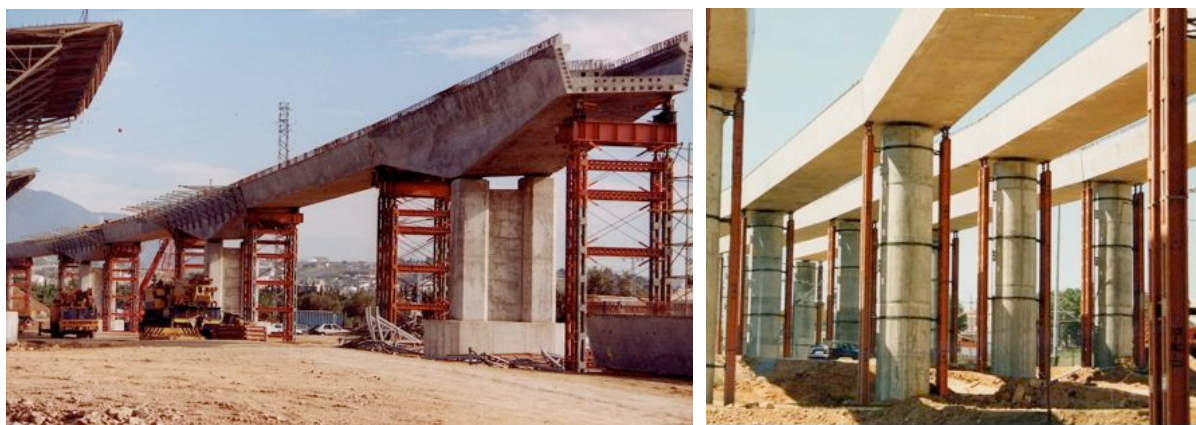
Fig. 7-48. Examples of towers used to bear pre-cast concrete elements. Left: Courtesy of RMD. Right: Courtesy of Alvisa.
