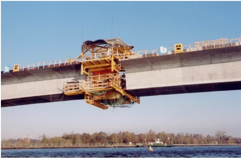
Fig. 7-35. Formwork to do the link between both cantilevers. Courtesy of Setra/CTOA, Gerard Forquet.
