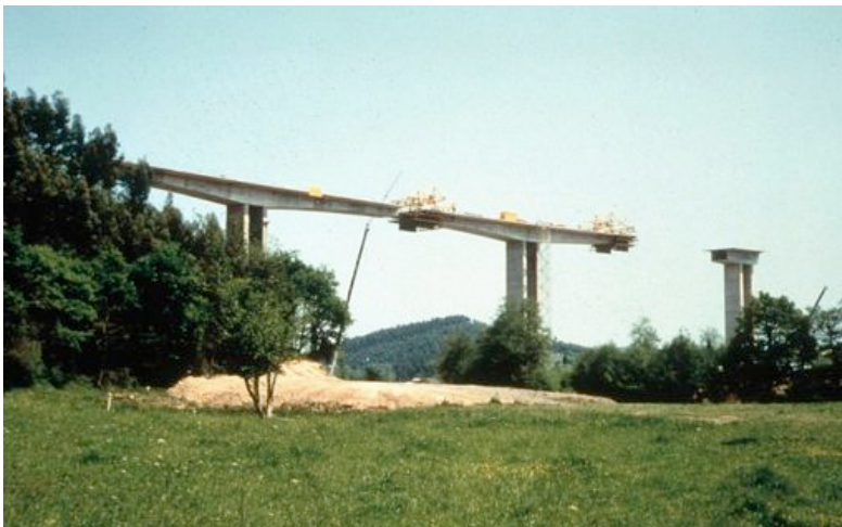
Fig. 7-38. The space between cantilevers must be large enough for the removal of the internal formwork. Courtesy of Ferrovia-Agroman.
