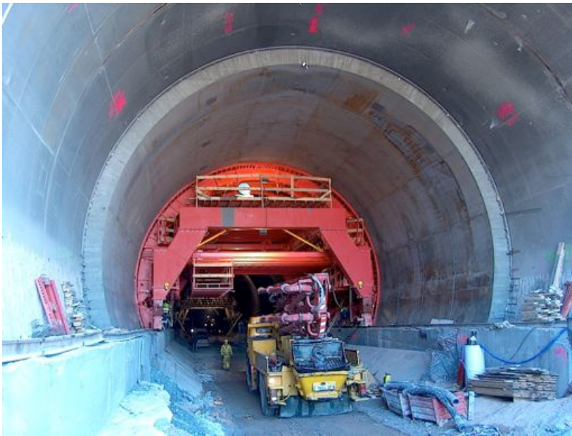
Fig. 7-16. Formwork for a bored tunnel with self-compacting concrete. Courtesy of Ferrovial Agroman.
