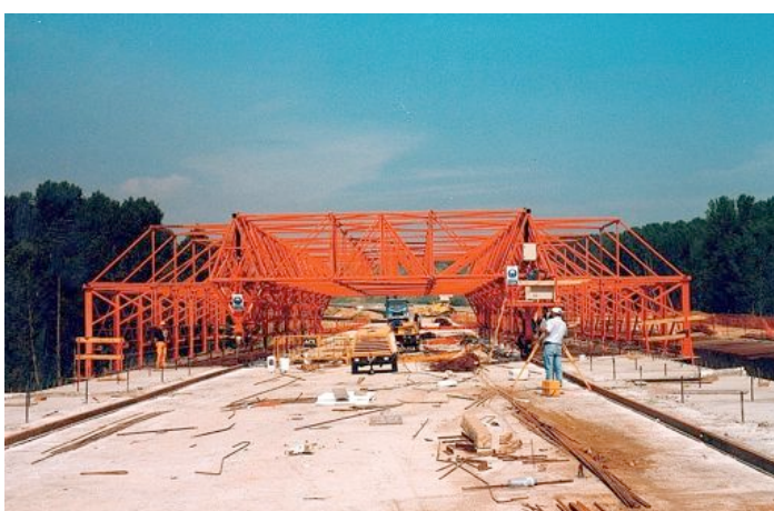
Fig. 7-10. Sometime it is necessary to allow enough space to pass materials. Courtesy of PERI.
