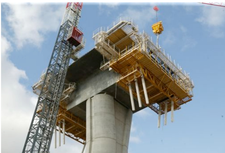
Fig. 7-37. Accesses in safety conditions must be provided. Courtesy of Setra/CTOA, Gerard Forquet.
