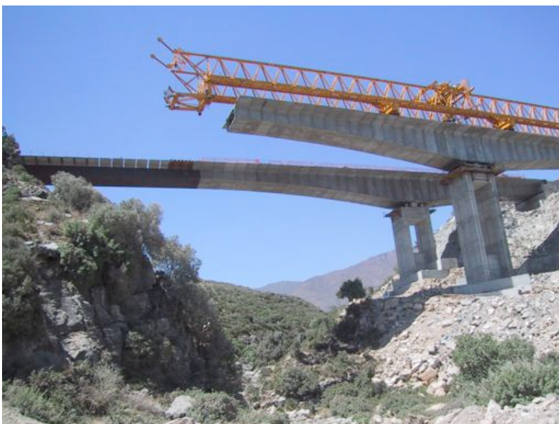
Fig. 7-47. Launching a hybrid deck with precast segments and a composite beam. Courtesy of Ferrovia-Agroman.
