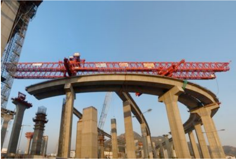
Fig. 7-46. Launching precast segments with a very small radius in plane. Courtesy of Bouygues Travaux Publics.
