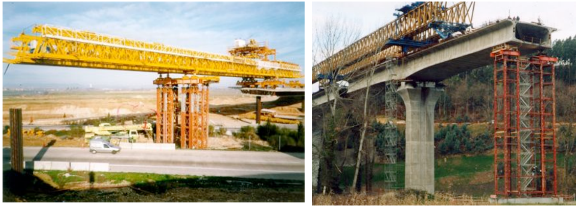
Fig. 7-49. Towers used for the temporary bearing of constructive solutions using travellers. Left courtesy of Ferrovial-Agroman. Right courtesy of RMD.
