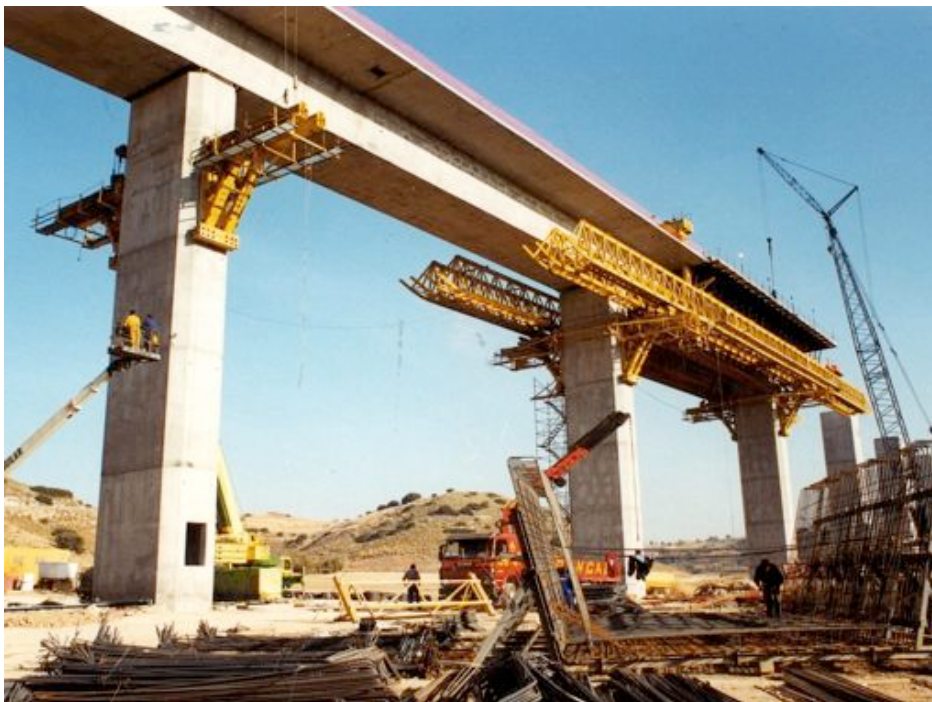
Fig. 7-28. Prefixed cages of reinforcement are essential to obtain a good performance. Courtesy of Ferrovial-Agroman.
