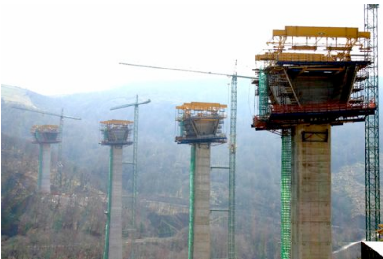
Fig. 7-39. The wind load action on tall bridges can be quite important. Courtesy of Ferrovia-Agroman.
