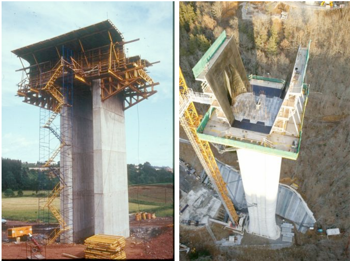
Fig. 7-32. Two examples of special formwork for the first segment. Left: courtesy Ferrovial-Agroman; Right: Courtesy of Bouygues Travaux Publics.
