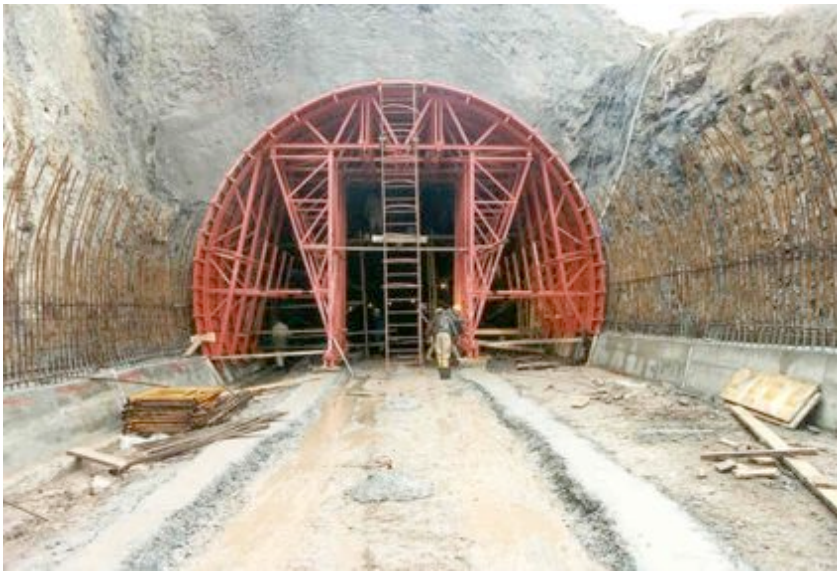
Fig. 7-14. Cross view. Notice the space to allow the passing of trucks. Courtesy of PERI.
