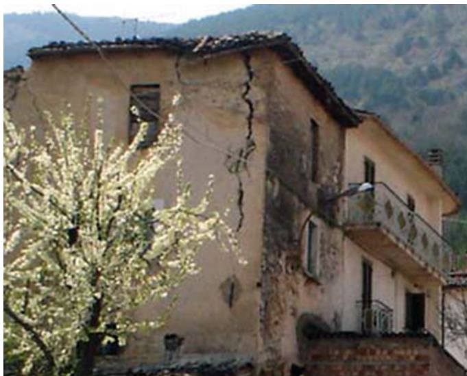
Fig. 11.36 Overturnig detachment of facades
