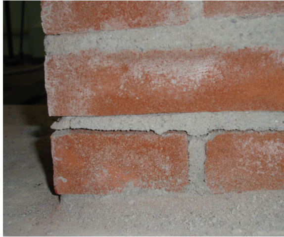
Fig. 1.34 Detachment of brick and mortar joints in a section of a masonry arch
