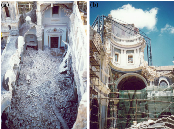
Fig. 2.80 a The interior of the church after collapse; b the collapsed dome
