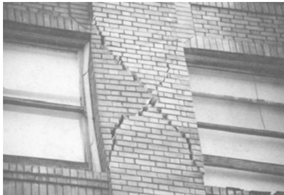
Fig. 11.13 A typical X cracking occurring in a wall pier
