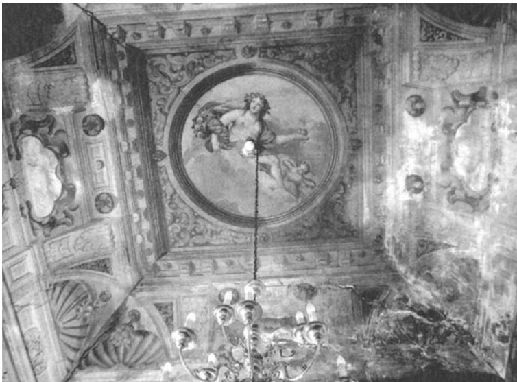
Fig. 6.58 Typical cracking pattern at the corners of a cloister vault; Palazzo Martinengo delle Palle in Brescia (Tomasoni 2008)
