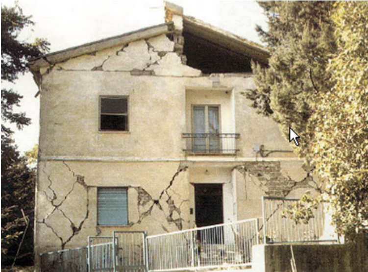
Fig. 11.46 Damagement of a multi-storey wall under in-plane seismic actions
