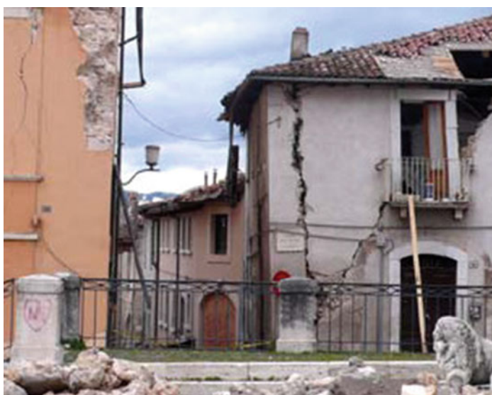
Fig. 11.37 Overturnig detachment of facades
