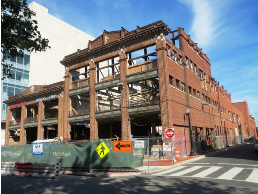
Figure 5.4 Wonder Bread Building (White Cross Bakery), Washington, DC, USA. Photographs provided courtesy of Dr Smith.
