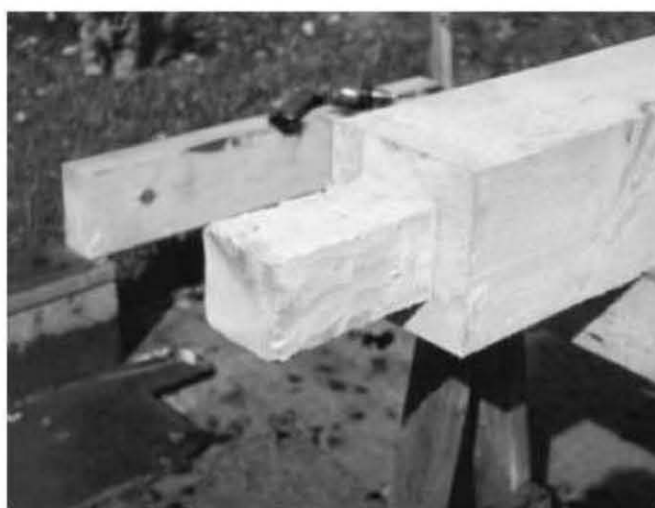
Fig. 4.31: The four eight-by-eight corner posts have two inches of wood removed all the way around the top of the post, down to a shoulder eight inches from the top. Again, this is accomplished by combining saw cuts with chisel work. All of the post tops for the garage are shaped in this way before they are stood up and plumbed, but sidewall posts need shoulders on just the inner and outer sides, not all four.
