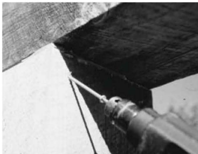
Fig. 5.32: A couple of screws hold the girder in place. Right-angle connectors are good in this situation, too.
