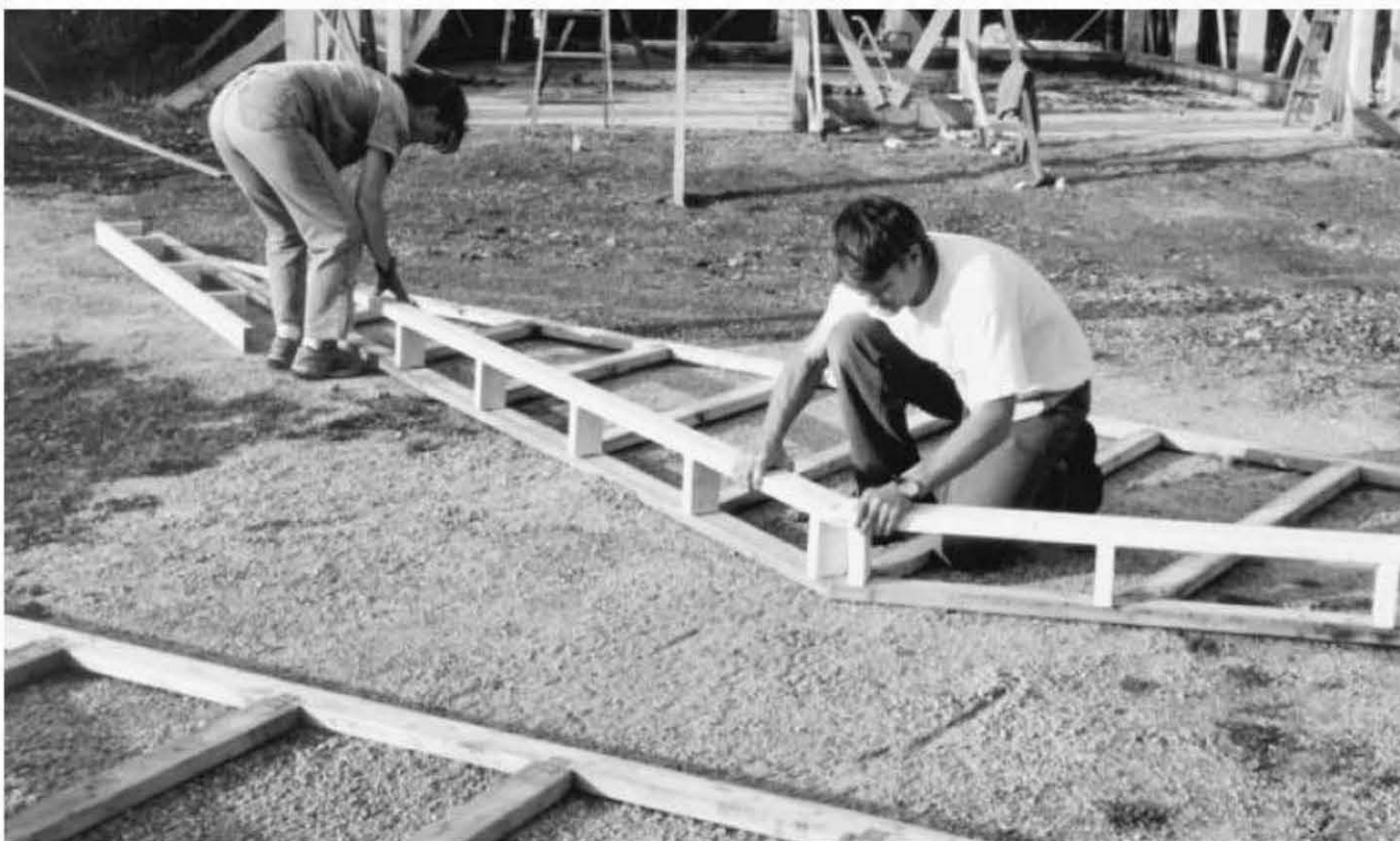
Fig. 4.50: Chris and his wife, Kat, make and install the “ladder” to the two gable trusses, to provide an overhang. Note that the gable trusses have lots of vertical members, instead of the angled tension and compression chords. With the ladder and number of vertical members, these trusses are probably about twice as heavy as the others. They can be installed after the other trusses are well-braced to each other.
