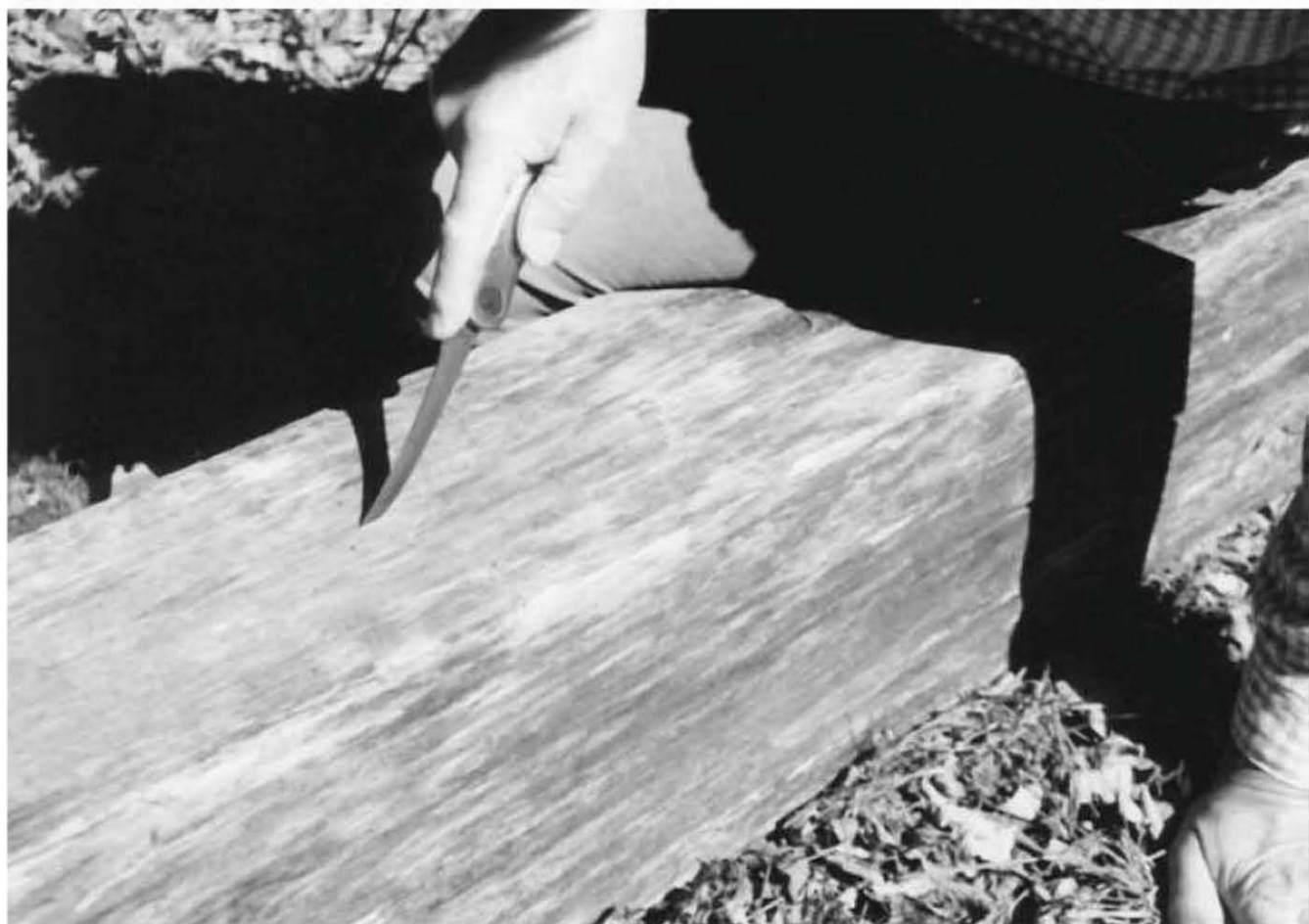
Fig. 3.1: The author uses a knife to probe an old timber for soft or deteriorated wood. This one was a reject.
