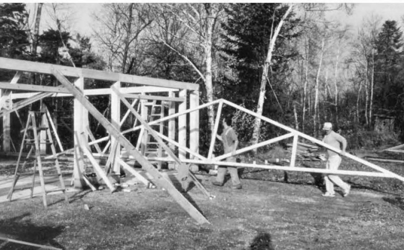
Fig. 4.45: These engineered trusses are strong even for our North Country snow loads, but are made from two-by-fours, so they are not very heavy.
