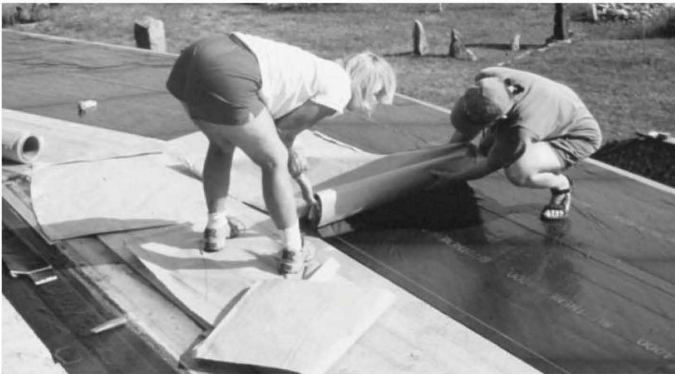
Fig. 5.37: Diane Lukaris and Jaki Roy roll out the Bituthene™ 4000 waterproofing membrane onto the wooden substrate, which has already been primed with a compatible acrylic primer provided with the product. The backing paper is removed as the 36-inch-wide membrane is rolled out, exposing a very sticky bitumastic membrane that adheres extremely well to the primed wooden deck. The ladies are careful to maintain the required three-inch overlap between adjacent courses.
