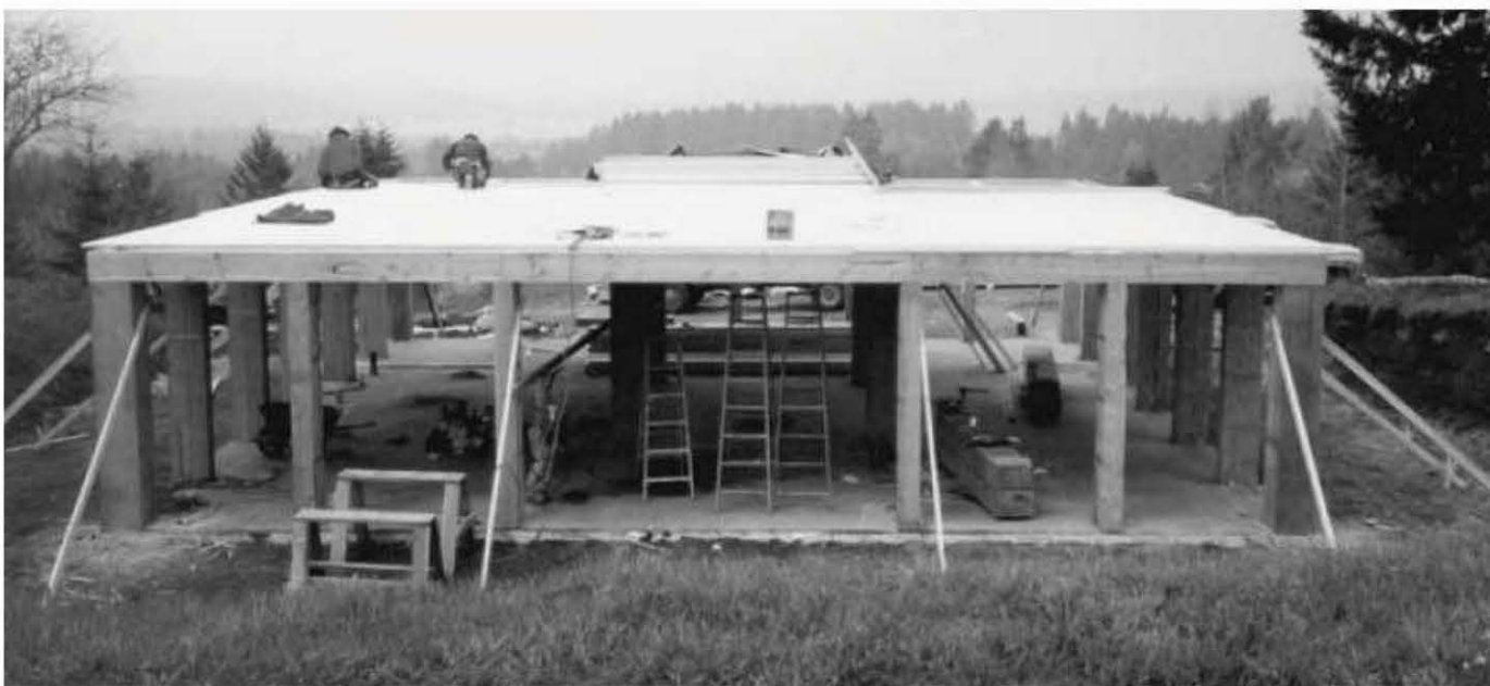
Fig. 4.58. Joe's Rocket Research Landing Pad is ready for a rocket to land. The plank roof will receive the roof trusses. Joe Zinni photo.
