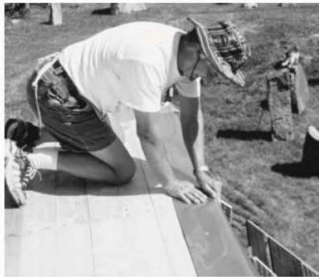
Fig. 5.36: The author makes a drip edge by bending two inches of a seven-inch-wide piece of flashing over the edge of the south overhang.
