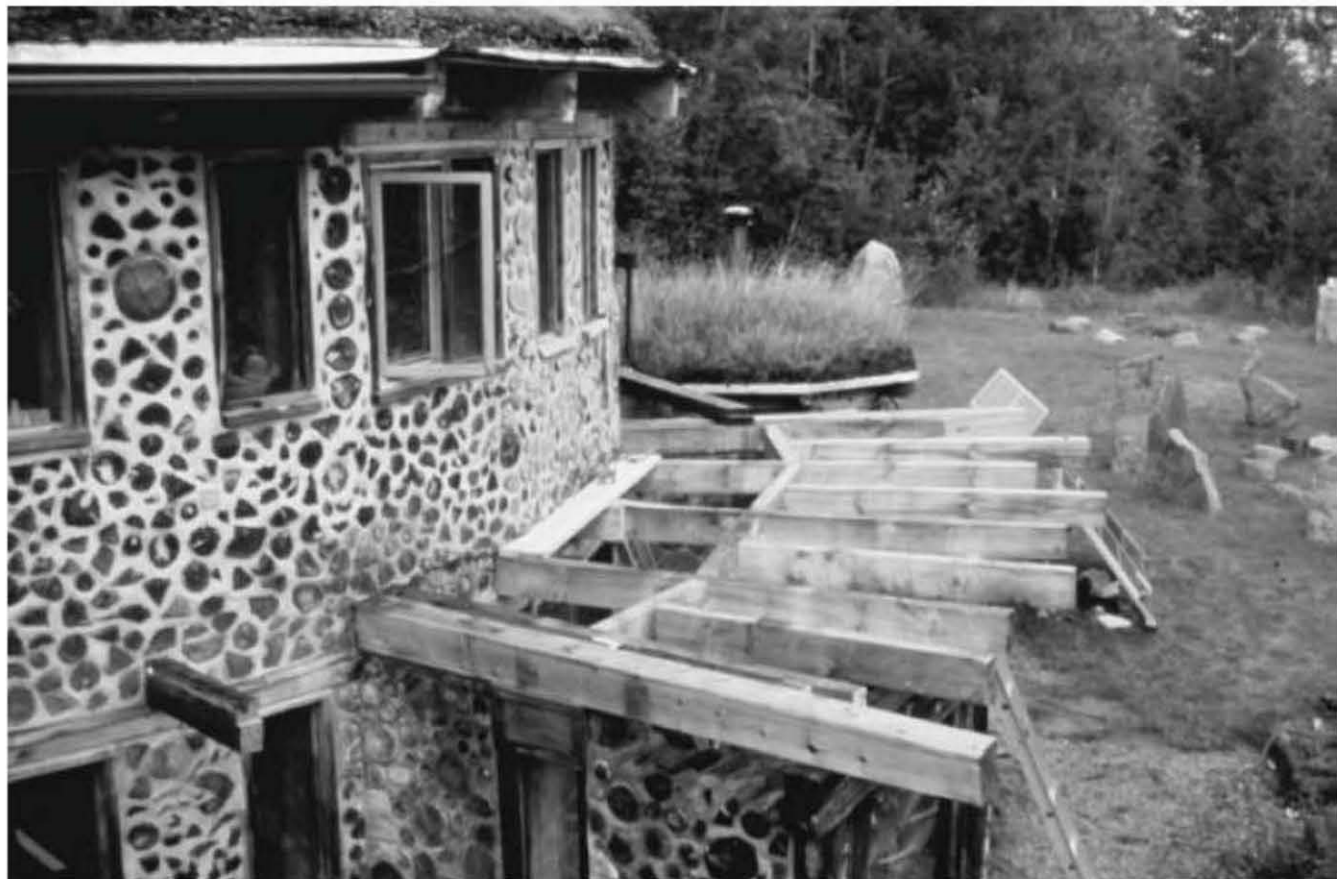
Fig. 5.19: The floor frame for the new room is completed, and the first two flooring planks are installed.
