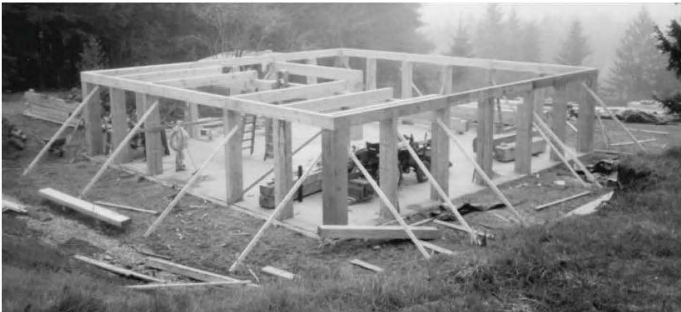
Fig. 4.57: The basic post and beam frame is almost completed. Joe Zinni photo.
