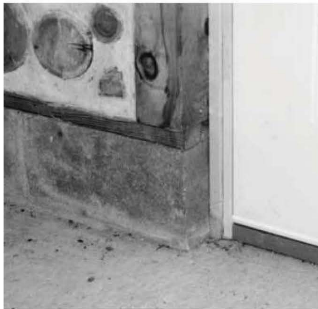
Fig. 4.3: Here, the posts — and the cordwood walls — are built up on a pressure-treated wooden plate one course of blocks higher than the floating slab.
