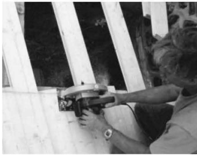
Fig. 5.21: The chalk-line has been snapped, and I cut the ends of all of the boards in this section at once. If done in the middle of a four-by-eight joist, this will leave a two-inch-wide bearing surface for the next facet. At the edge of the building, a straight overhang can be created in this way.
