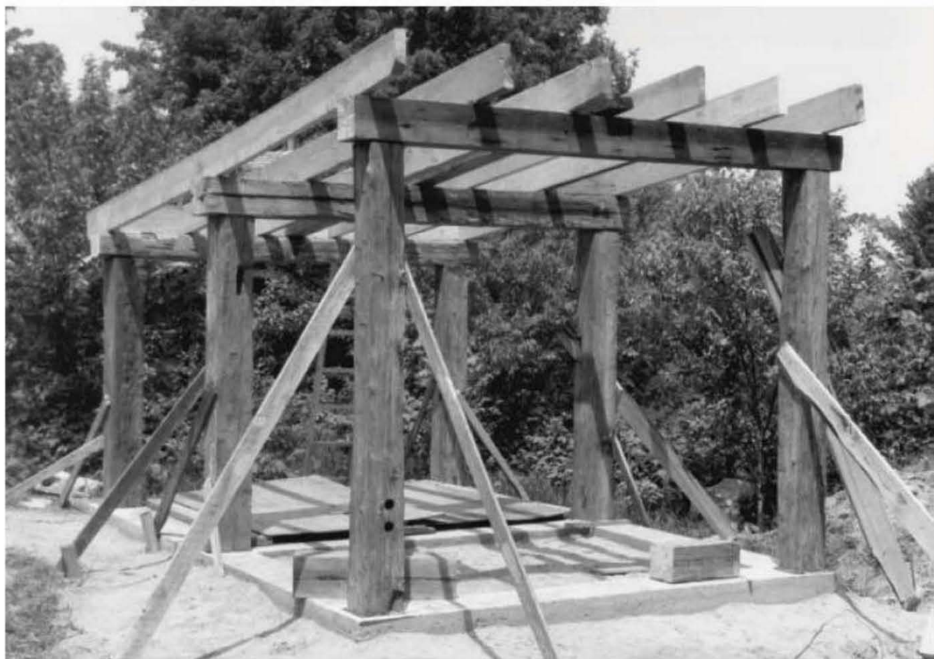
Fig. 2.21: The six posts are plumbed, then braced to stakes with scrap lumber.
