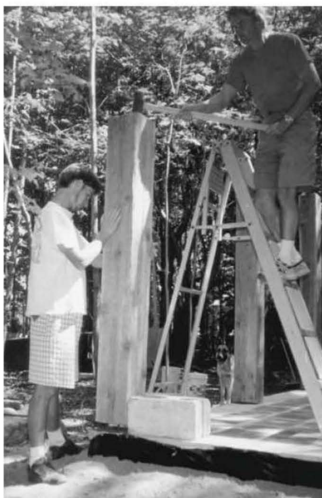
Fig. 4.5: Guided by adjacent blocks, Rohan holds the post in position over the pin. When Rohan nodded his head, I hit it with a sledgehammer. (The post, that is.)
