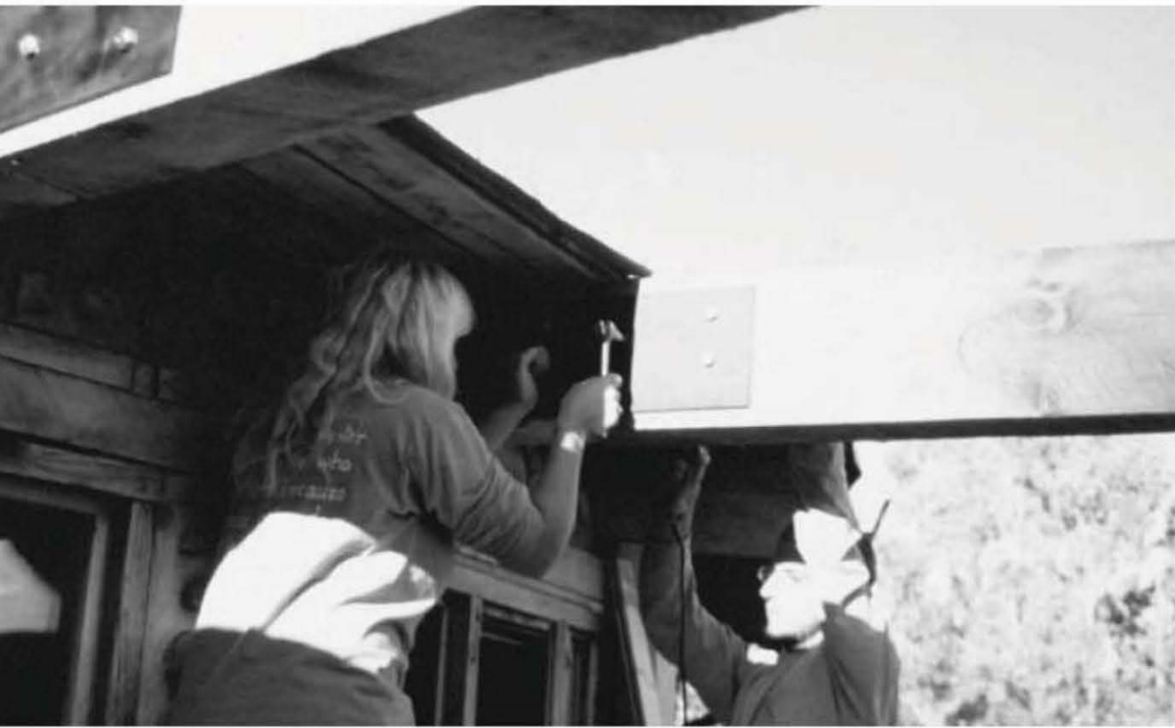
Fig. 5.34: Anna tightens lag screws up against the metal plate, which acts as its own washer. Rohan drills three-eighths-inch holes for the plate on the other side, appropriate for one-half-inch lag screws. He hangs the plate in position on two small screws, which hold it in place while he drills his holes.
