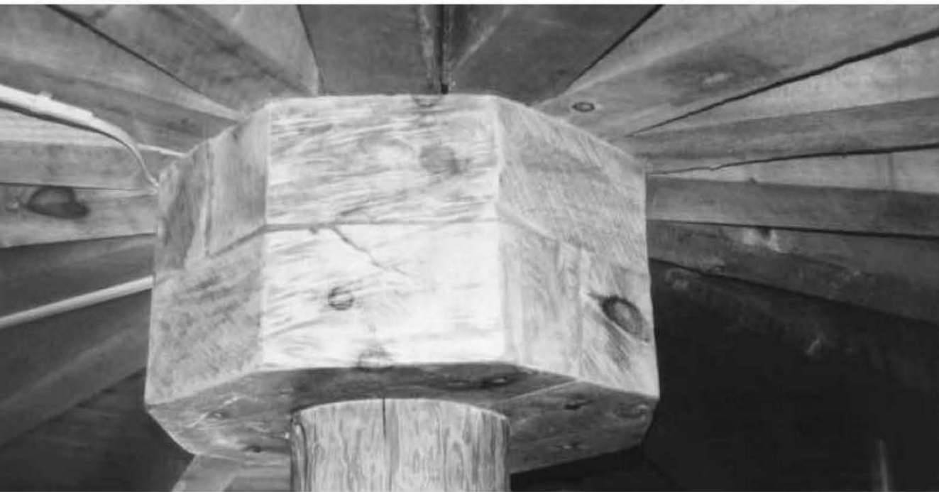
Fig. 4.28: At the Earthwood office, 16 five-by-ten radial rafters join over an octagonal capital. The capital, 12 inches (30.5 centimeters) high by 24 inches (61.0 centimeters) in diameter, is made from four pieces of six-by-twelve timber, with consecutive courses criss-crossed at 90 degrees to each other. The pieces are fastened together with 10-inch (25.4-centimeter) log cabin spikes, eight in all.
