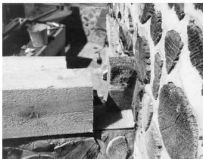
Fig. 5.7: I notched the east side eight-by-eight girt to fit it up against the stub of the original four-by-eight rafter. I chiseled and scraped deteriorated wood, back to sound material, and doused the area with a water-sealing product. Note the use of Sill Seal™ between the girt and the top mortar joint of the cordwood wall.
