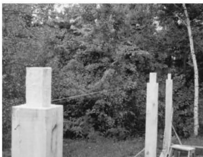
Fig. 4.32: Here, the three major eight-by-eight posts along the sidewall are in place. The middle post is set to the stretched nylon mason’s line. Corner posts are shaped as in the previous picture, Fig. 4.31, and the middle eight-by-eight has had just its sides trimmed back two inches to receive the two-by-eights, butted together on the shoulder.
