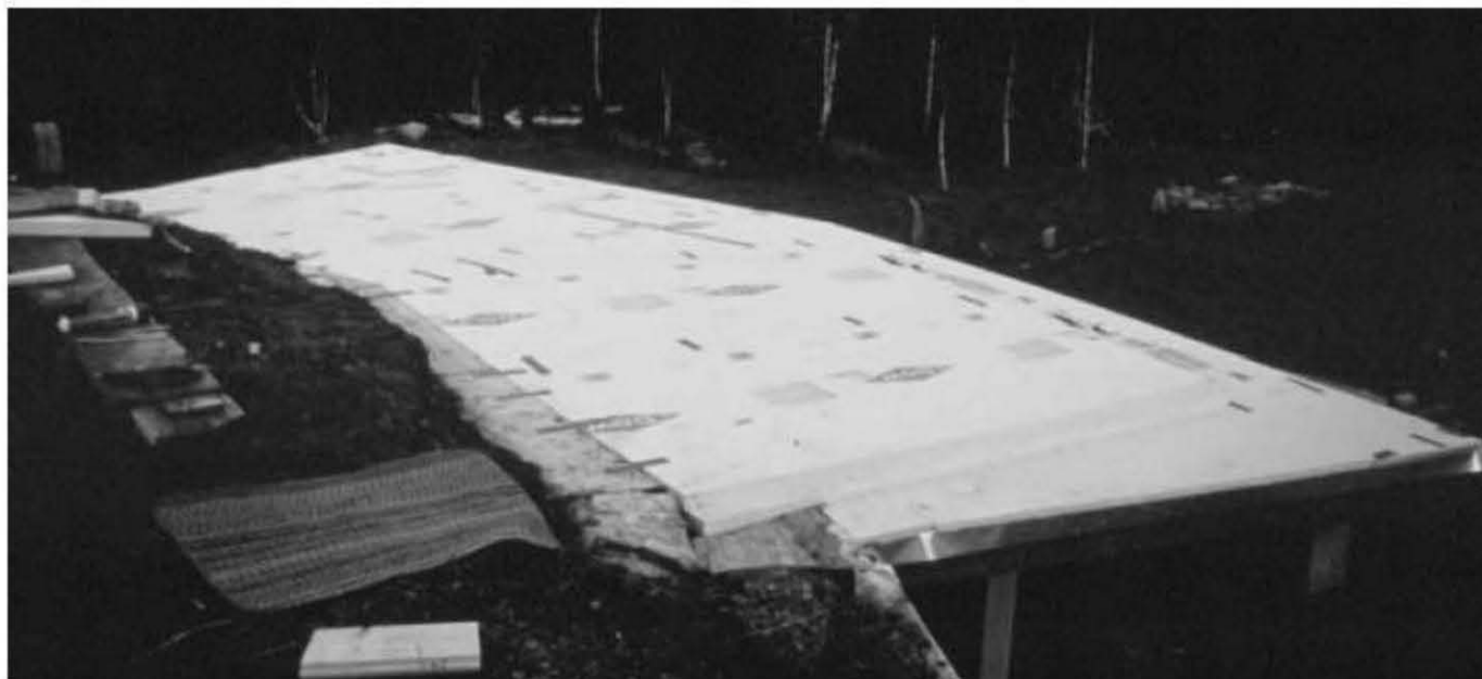
Fig. 5.38: We installed 4 inches of Dow Styrofoam™, an extruded polystyrene, over the membrane.
