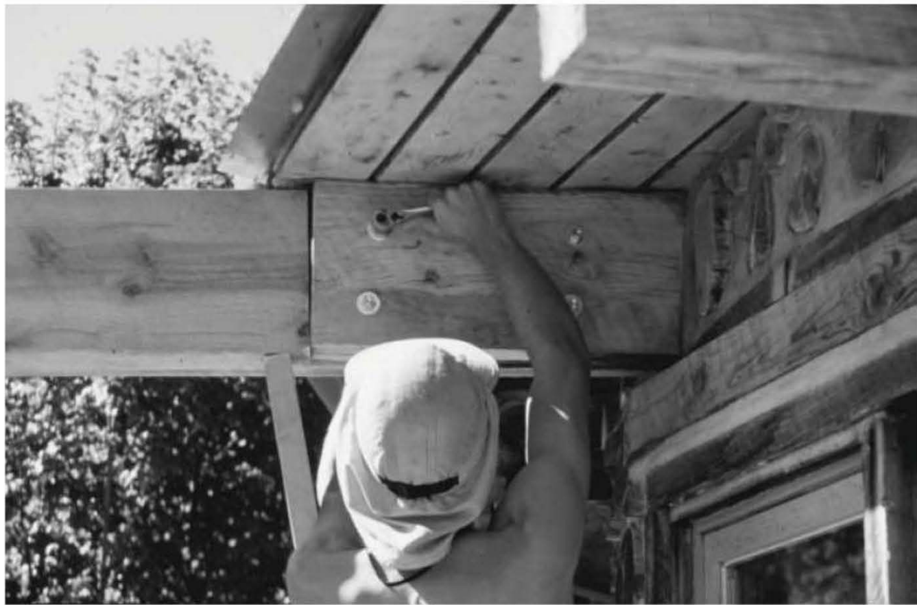
Fig. 5.33: Rohan Roy tightens the nuts onto the lag bolts. Four one-half-inch lag bolts are plenty strong enough to make this joint.
