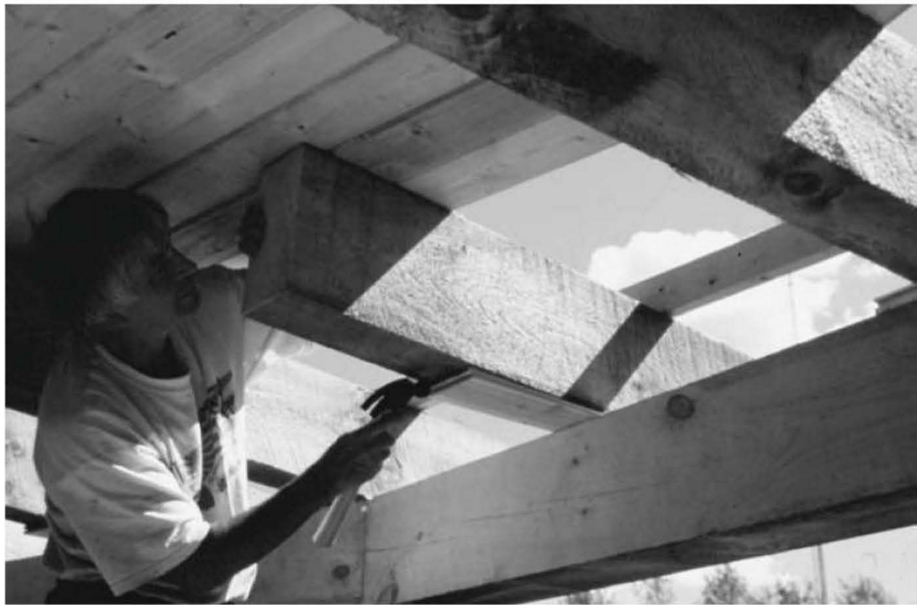
Fig. 5.35: The author checks the rafter position against pencil lines, while tapping in a couple of cedar shingles to snug it in place. Note the wooden straightedge outside the building, to assure that planking will hit all three rafters in a single flat plane. Anna Milburn-Lauer photo.
