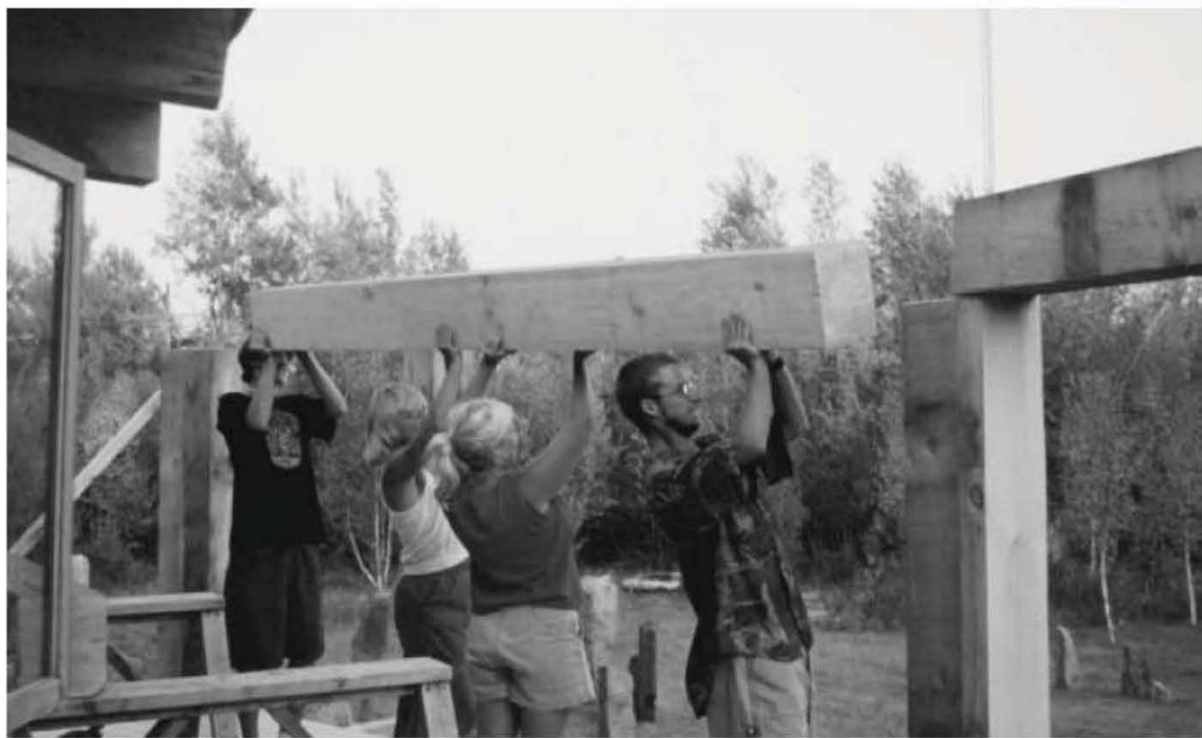
Fig. 5.31: Sons Rohan (right) and Darin (left) lift the ends up onto the tops of the double-wide posts, while Jaki and Anna lighten their load with assistance from below.
