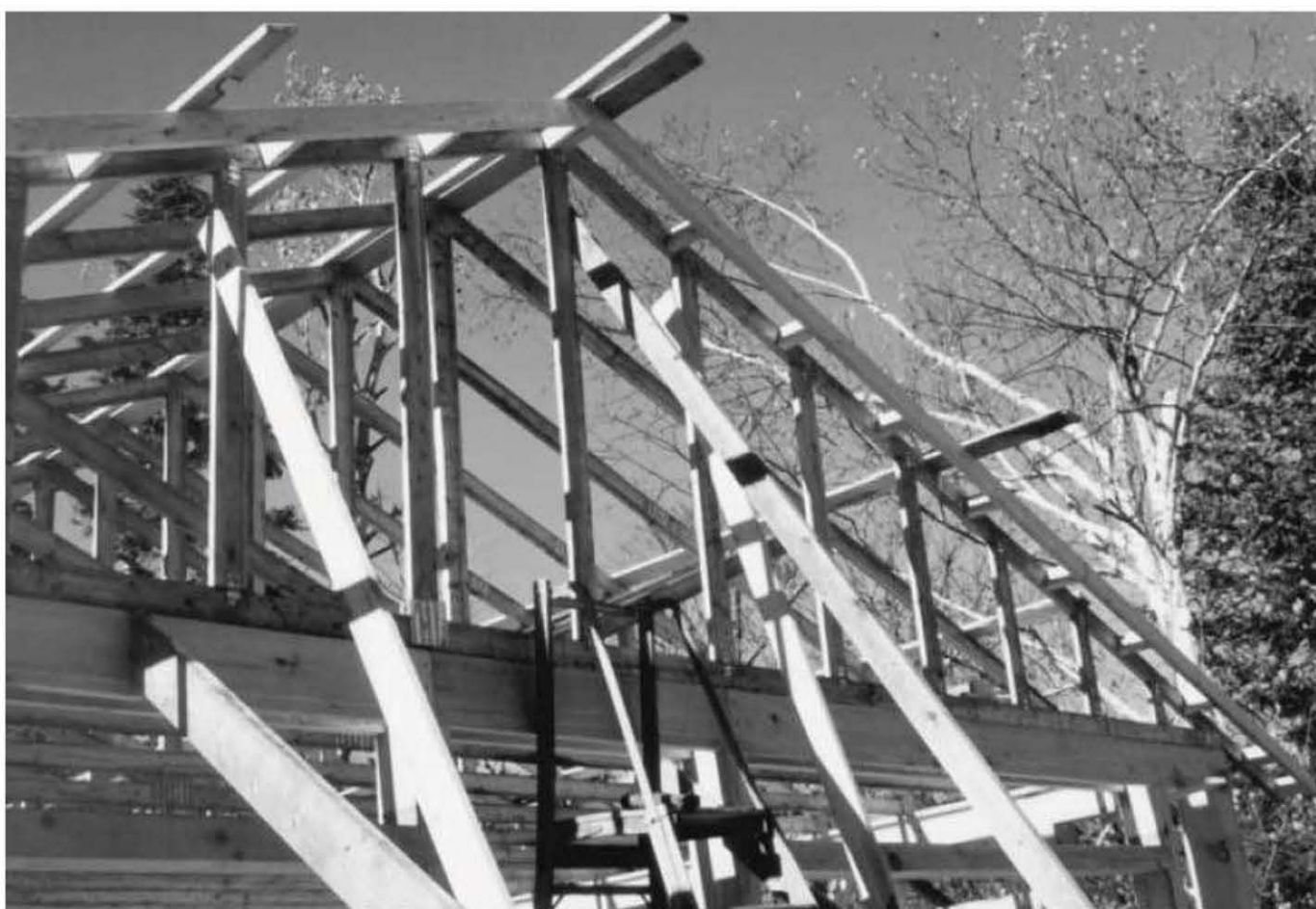
Fig. 4.51: The last truss, a gable truss, is braced in place. Once the trusses are in place, roofing options are to install horizontal boards called “purlins” and metal roofing, or the entire roof can be planked or decked with plywood for installation of shingles.
