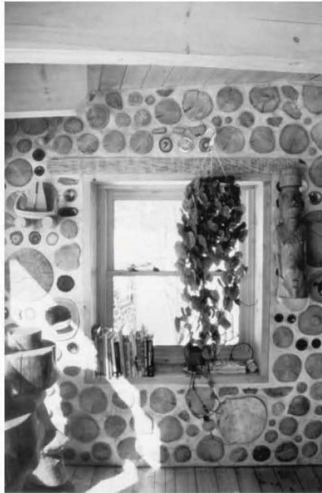
Fig. 5.42, near right: The west wall of the new sunroom. The double-wide four-by-eight lintel over the window carries the load down to the cordwood wall without placing pressure on the window itself.
