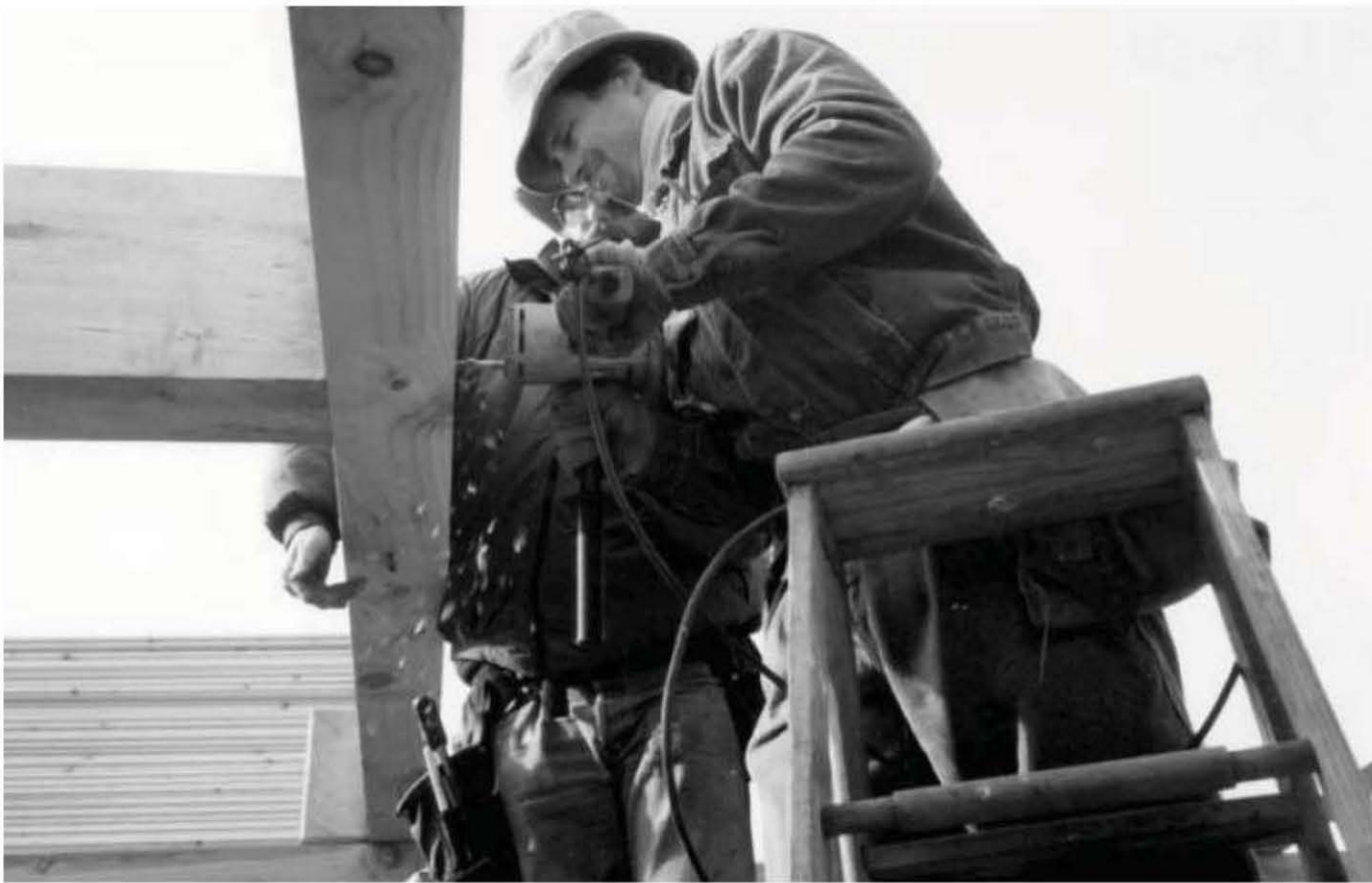
Fig. 4.56: Joe Zinni fastens one six-by-twelve timber to another with two large lag screws. Joe Zinni photo.
