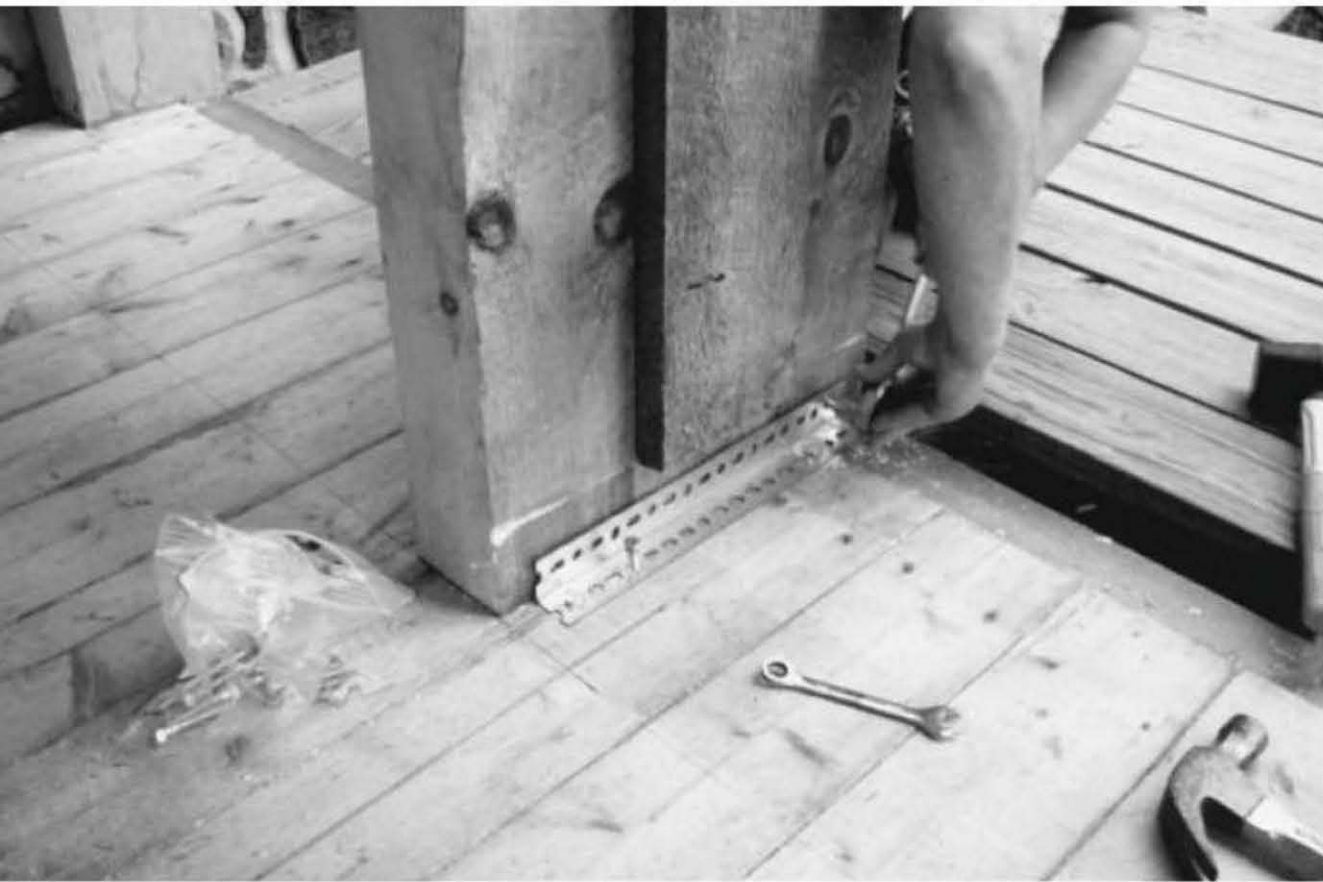
Fig. 5.40: The one-by-six key piece locks the doorframe to the cordwood wall. The angle iron ties the doorpost to the floor.
