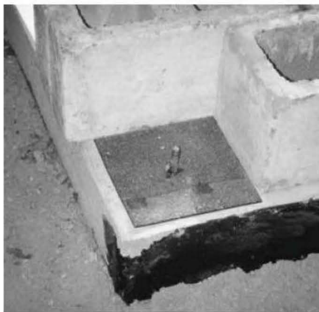
Fig. 4.4: The damp-proof square covers the footprint where the eight-by-eight posts will stand.
