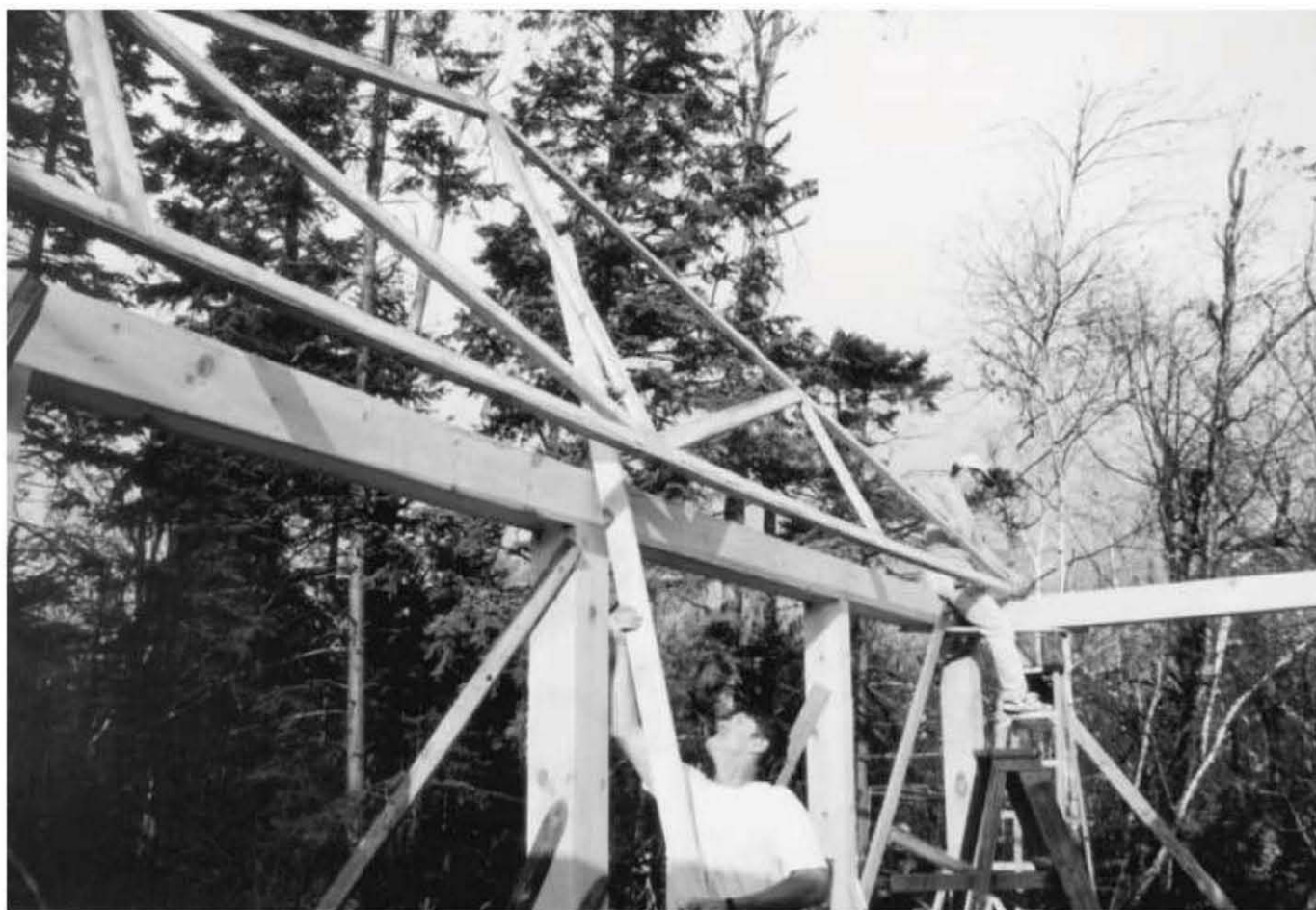
Fig. 4.47: Chris started with the second truss from the end, well braced to the ground. The first and last trusses, called the gable trusses, have overhangs built into them, which makes them more difficult to deal with. After all the other trusses are braced firmly in place, the two gable trusses are installed. The 24-inch centers are already marked on the sidewall girts, and each truss is given exactly the same overhang at each end. Once the overhang has been determined at both ends of the first truss, the others can be marked exactly the same. Before the crew arrived, Chris made sure that his sidewalls were straight and well-braced from the sides.
