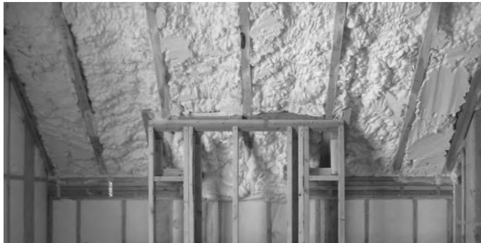
Figure 6-1 Spray-in Icynene foam insulation acts as an air barrier as well as insulation. Photo courtesy of Magleby Companies.
