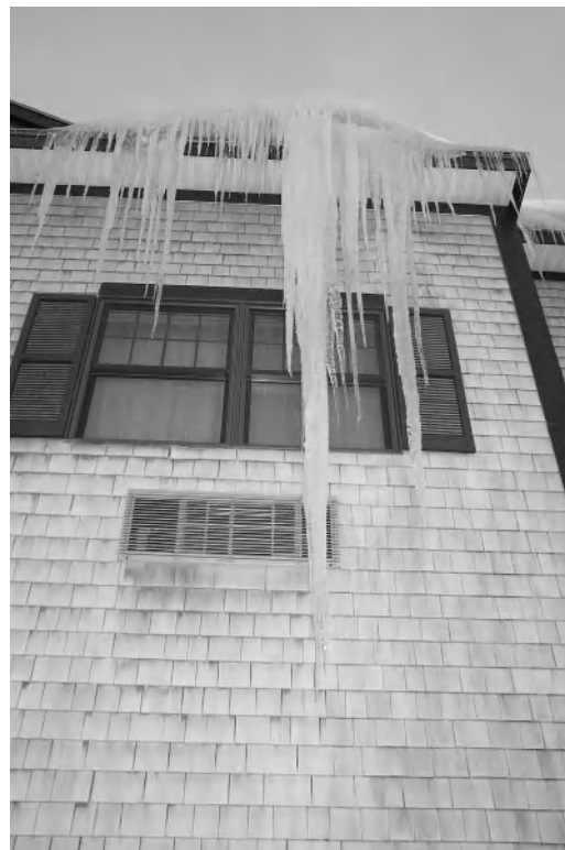
Figure 2-3 Icicles like these on a Maine hotel can form when heat escapes through the roof, melting snow and ice. Water runs off and refreezes at the eave, creating an ice dam that blocks further water runoff. Conditions like this can often be avoided with proper insulation and attic ventilation. Photo courtesy of National Oceanic and Atmospheric Administration/Department of Commerce.
