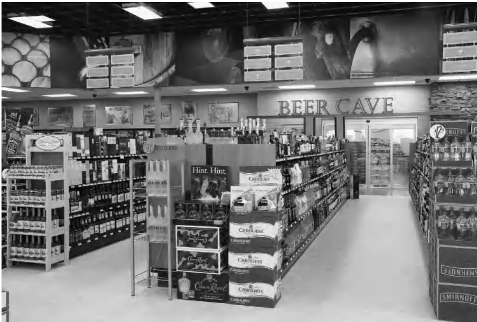
Figure 9-9 The Beer Cave is a walk-in cooler where shoppers can pick up cases of beer. The cooler is integrated with the geothermal heat pump system. Photo by Brian Droege. Courtesy of CNH Architects.
