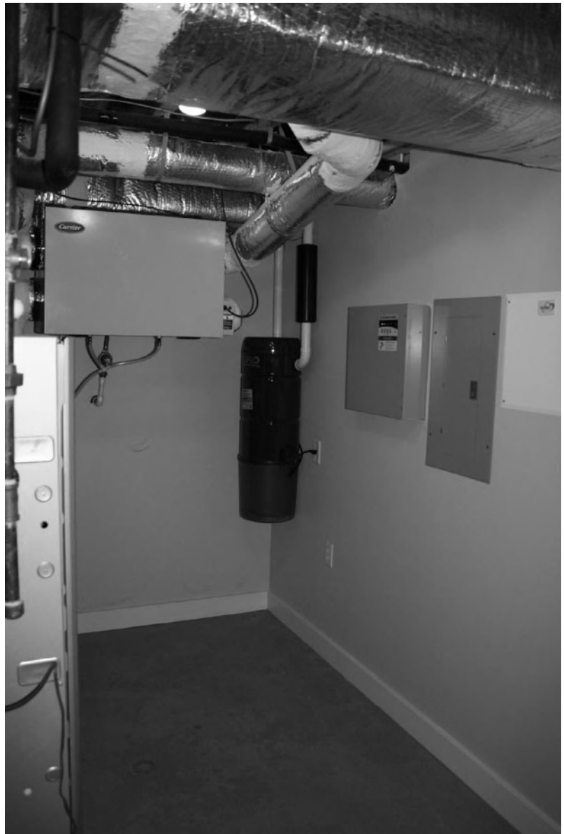
Figure 3-6 The mechanical room features insulated and sealed ductwork, a 13.0 SEER air conditioner, a natural gas hot water heater, and a 94.1 AFUE furnace. Photo by Isaac Zuercher.
