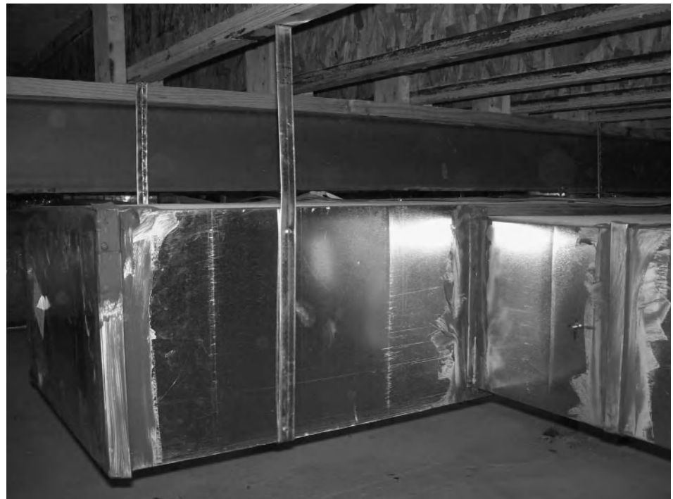
Figure 5-2 Sealing ducts with mastic increases energy efficiency and improves comfort and indoor air quality. Photo courtesy of the McKee Group.
