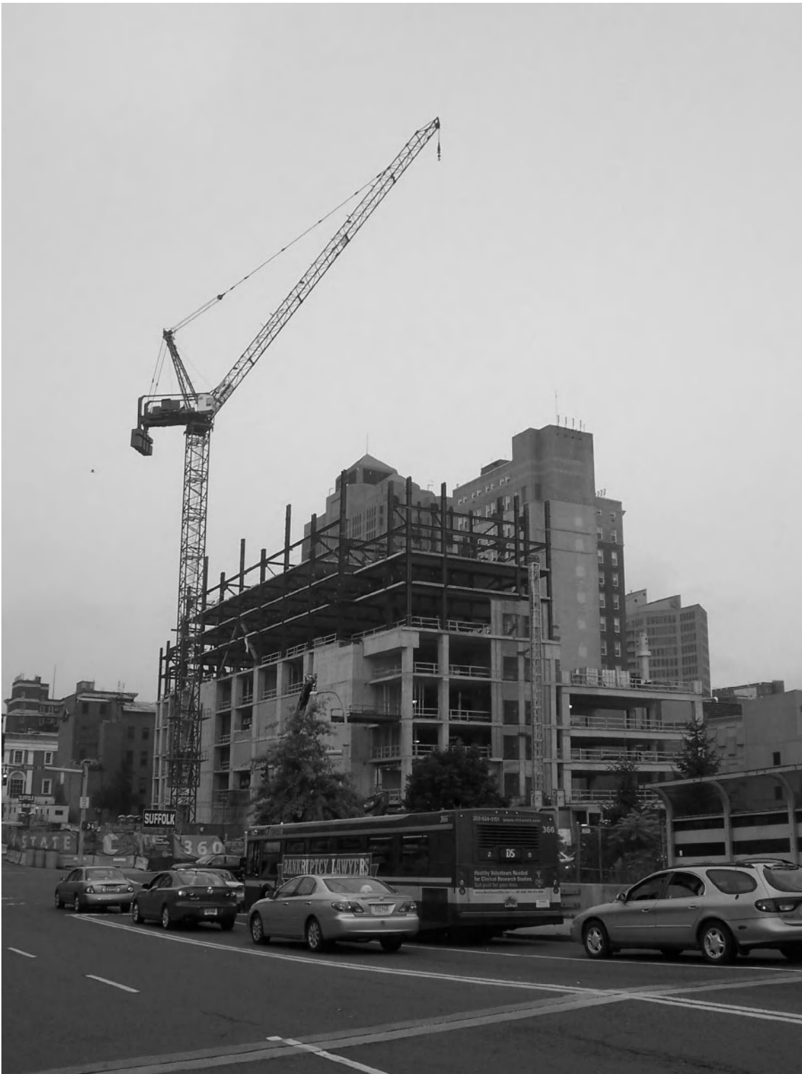
Figure 10-3 This mixed-use development under construction on a former parking lot in downtown New Haven, Connecticut, addresses many Sustainable Sites credits. Developed and designed by Becker + Becker of Fairfield, Connecticut, this 700,000-square-foot project is in the LEED for Neighborhood Development pilot program.
