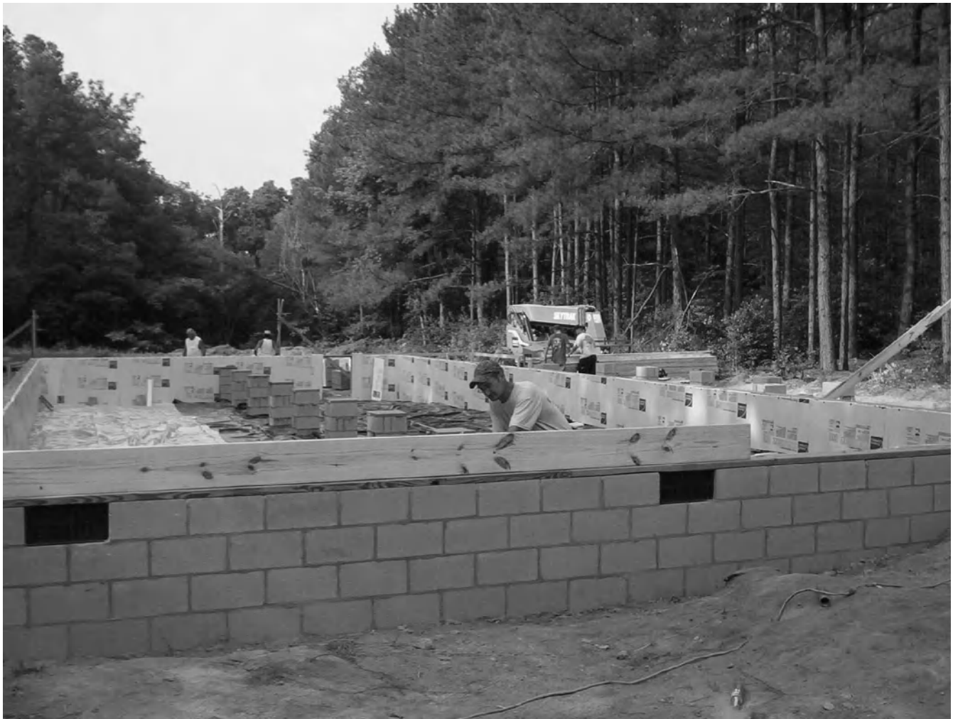
Figure 5-5 The insulated crawl space improves energy efficiency. Photo courtesy of Carolina Log Center.
