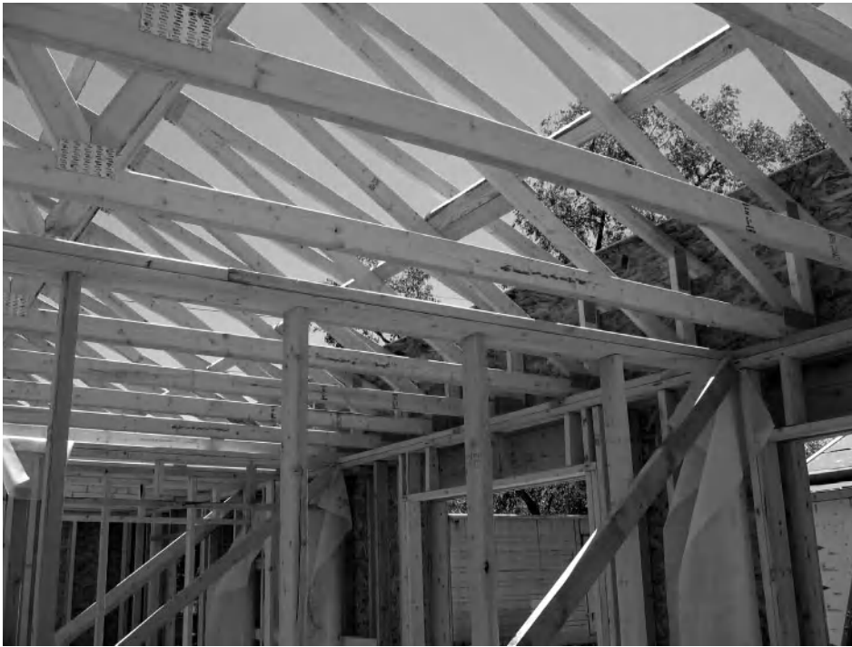
Figure 5-3 Raised-heel truss attic construction allows adequate room at the eaves for full-depth insulation to extend to the exterior wall. In this case, R-60 insulation will be installed. Photo by Paul Norton, courtesy of DOE/NREL.
