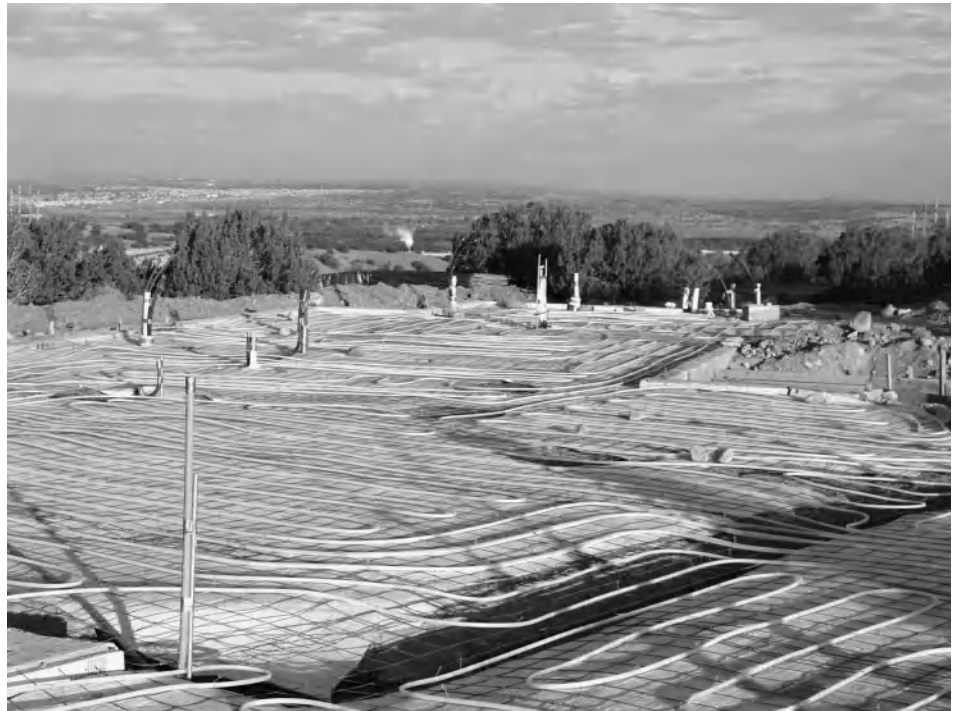
Figure 5-11 The reflective thermal blanket under the radiant floor heating system improves energy performance. Photo courtesy of Kayeman Custom Homes.
