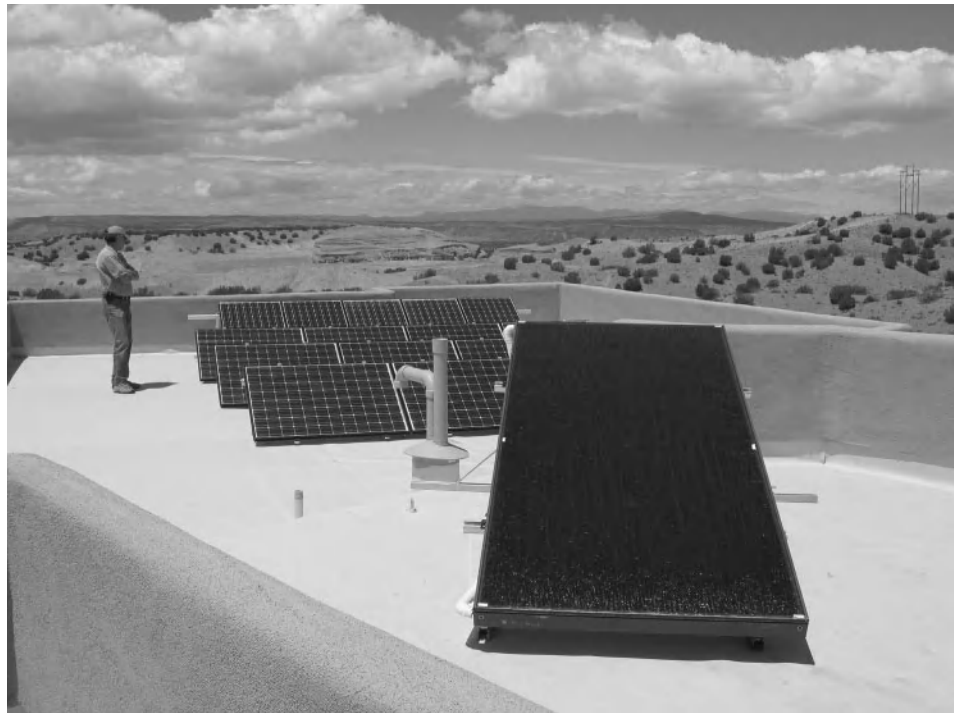
Figure 5-9 Renewable energy sources in this home include a solar thermal domestic hot water system and 3kW solar photovoltaic system. Photo courtesy of Kayeman Custom Homes.
