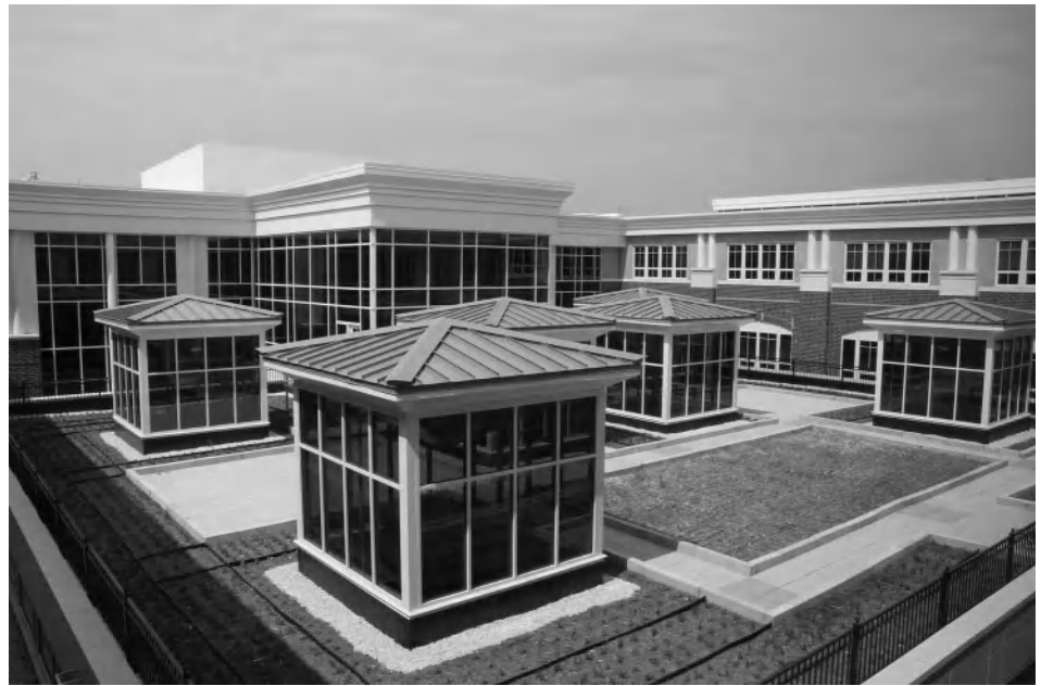
Figure 8-8 About 10,000 square feet of the roof is extensively planted. Image © 2007, Judy Davis/HDPhoto. Courtesy of Hoachlander Davis Photography, LLC.
