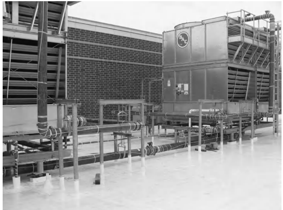
Figure 8-9 Each cell of the cooling tower has a variable-speed fan, resulting in energy savings over traditional constant speed fan operation. Image © 2007, Moseley Architects.
