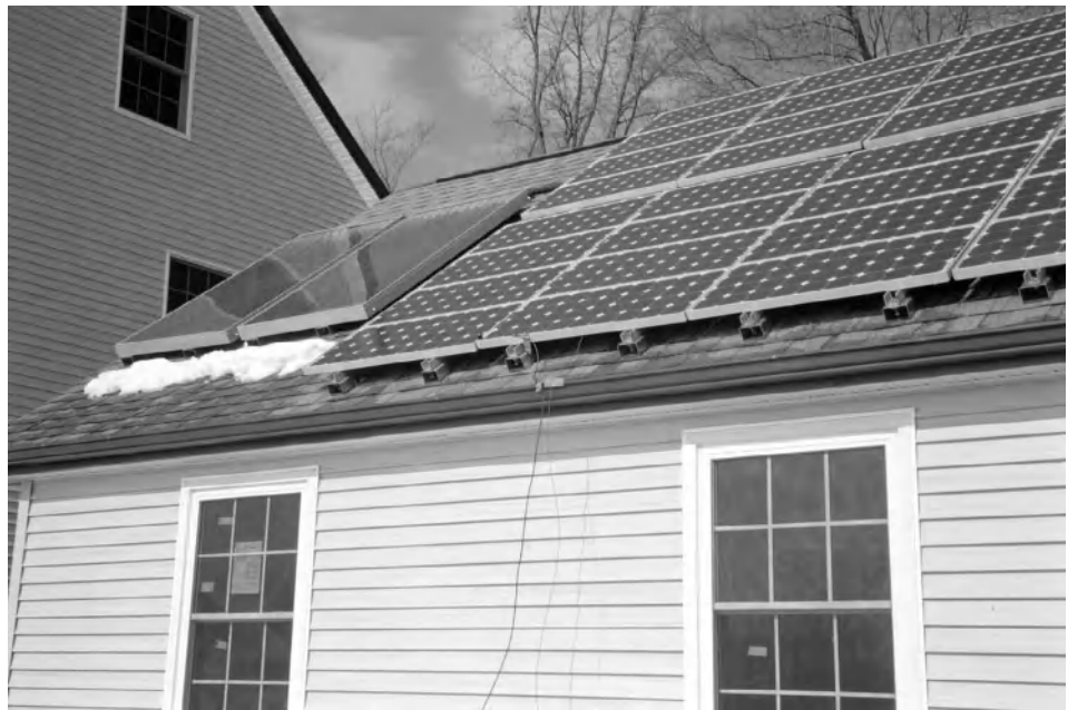
Figure 1-2 Solar panels on this California home will contribute to a savings of 60 percent on utility bills for this net-zero energy home. Photo courtesy of DOE/NREL.
