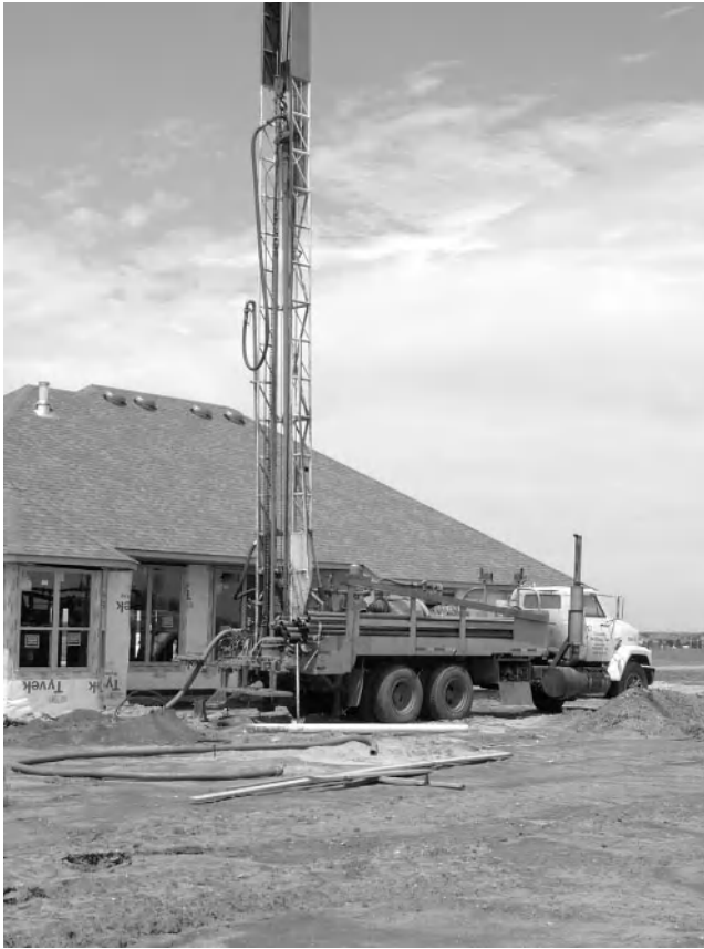
Figure 1-3 Drilling boreholes for a ground source heat pump system, also known as a geothermal heat pump system. This is a highly efficient renewable energy system for space heating and cooling and for water heating. Photo courtesy of Ideal Homes, www.Ideal-Homes.com .
