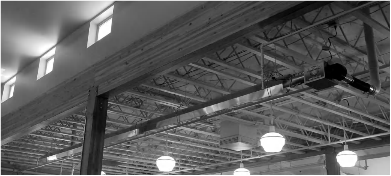
Figure 8-6 Two-stage infrared tube heaters provide primary heat for the building. © 2009, Architecture West, LLC.
