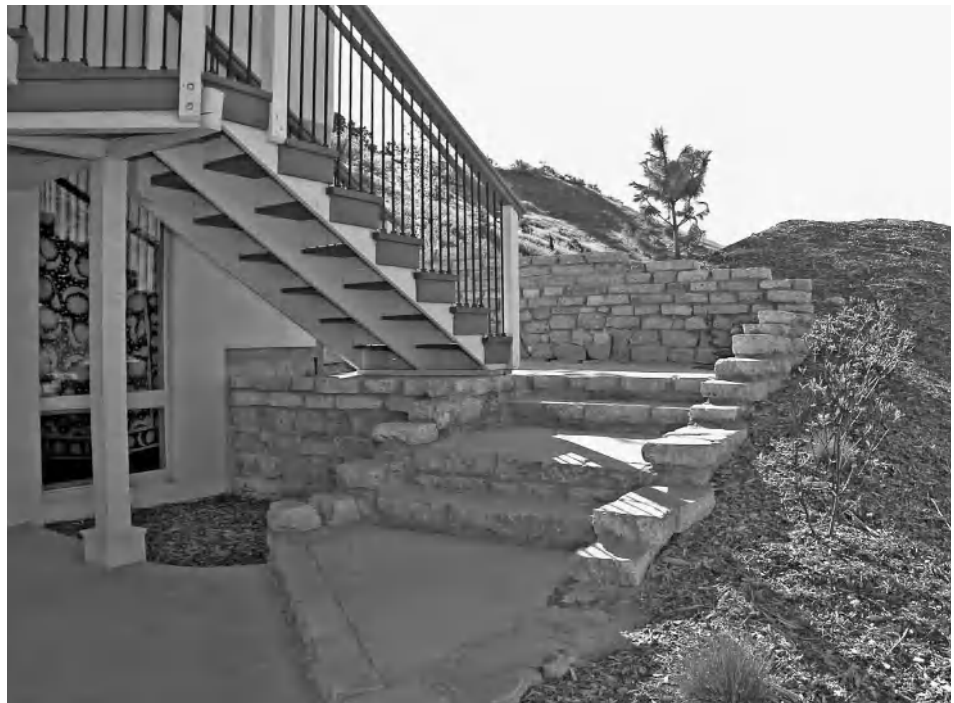
Figure 4-4 Recycled concrete was diverted from landfills and used for retaining walls and as a masonry veneer. Photo by Jennifer Hopkins, courtesy of Mark L. Hixson Design-Build.
