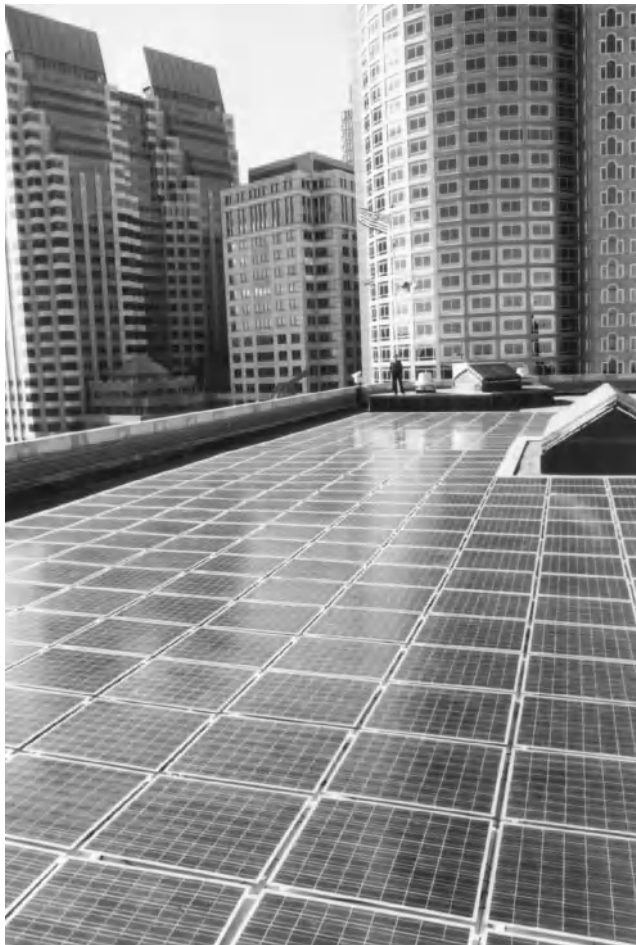
Figure 11-1 There are 372 solar panels in this photovoltaic system on the roof of the Williams Building in Boston. Image courtesy of DOE.
