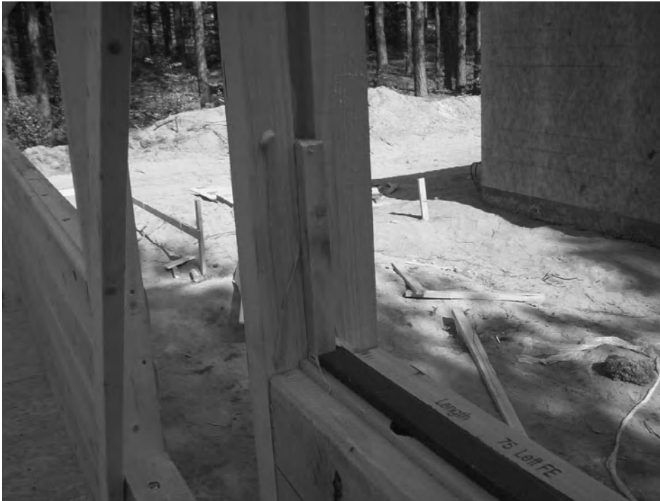
Figure 5-6 The black gasket on top of the log (right) will be compressed with the addition of the next log, creating a seal. Logs meet window and door openings with a tight seal formed by a spline and caulk. Photo courtesy of Carolina Log Center.
