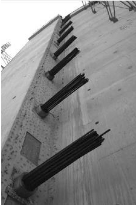
Figure 3.13 Prestressing anchorages at a buttress of a prestressed tank. (Courtesy of VSL International Limited, Hong Kong.)
