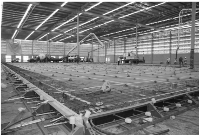
Figure 3.3 Examples of post-tensioned slabs before concrete casting. (Courtesy of VSL Australia, Sydney.)
