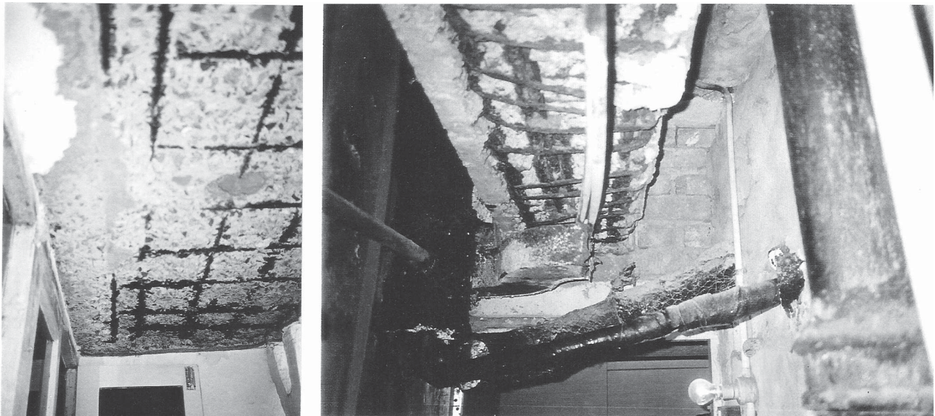
FIG. 4.5 Heavy corrosion of rebars in a 4-star hotel in Chennai due to permeable or less than nominal cover
