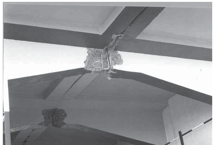
FIG. 7.17 Splitting bond failure in Surajbari bridge during Bhuj earthquake
