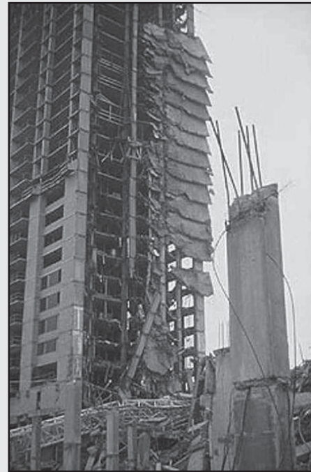
Progressive collapse of Skyline Plaza building in Virginia, USA
