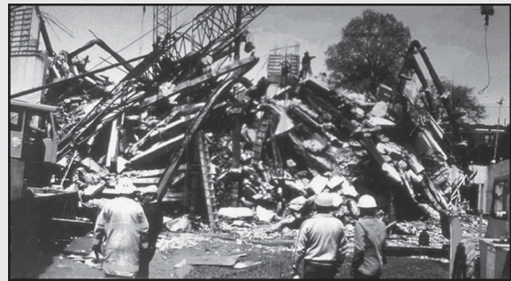
Collapse of L'Ambiance Plaza (Courtesy: The National Institute of Standards and Technology, US Department of Commerce)
