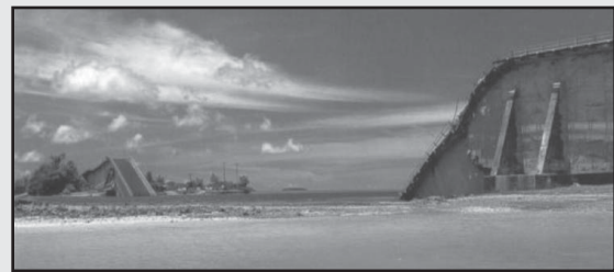
Koror–Babeldaob bridge—Before and after collapse
