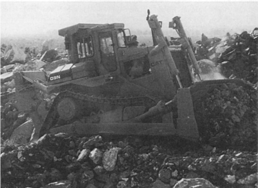
Local conditions are an important element in a contractor's costs, and working in unfamiliar areas can produce some unanticipated conditions. (Courtesy of Caterpillar, Inc.)
