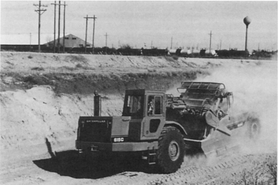
As newer and more productive equipment is developed, competitive pressure can accelerate the need to reinvest in new equipment. (Courtesy of Park Construction Company and Caterpillar, Inc.)
