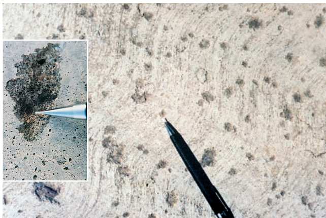
Figure 11-22. Popouts caused by ASR of sand-sized particles.
