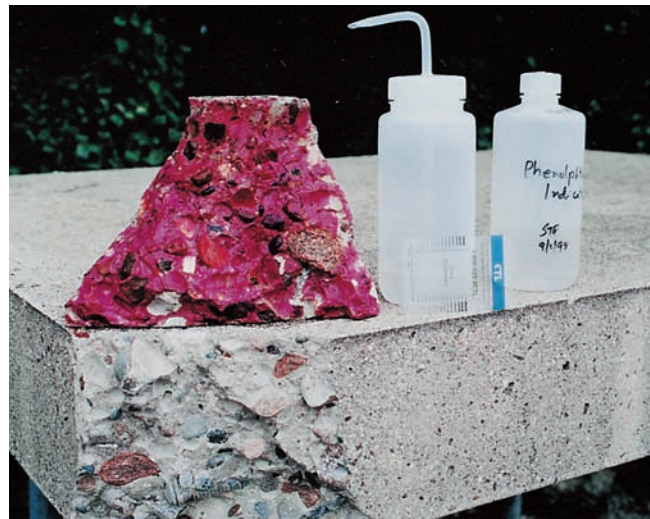
Figure 18-25. The depth of carbonation is determined by spraying phenolphthalein solution on a freshly broken concrete surface. Non-carbonated areas turn red or purple, carbonated areas stay colorless.
