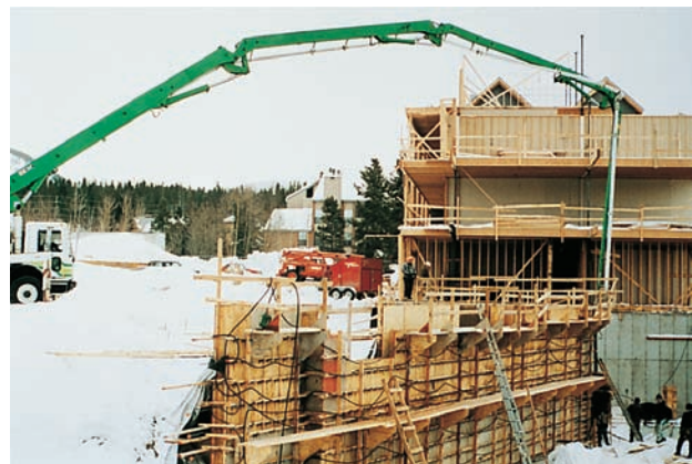
Figure 17-25. Hydronic system showing hoses (top) laying on soil to defrost subgrade and (bottom) warming the forms while fresh concrete is pumped in.
