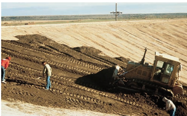
Figure 20-12. A dozer places a plant-mixed soil-cement on a slope for construction of a wastewater lagoon.
