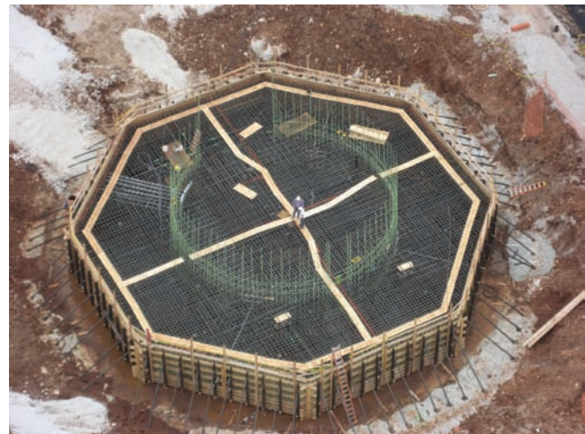
Figure 20-7. Large foundation placements as shown require mass-concrete precautions (Courtesy of Carson-Mitchell Construction Co.).
