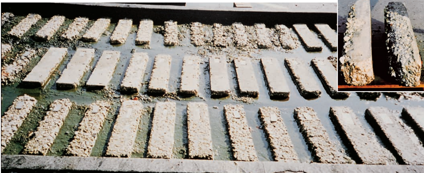
Figure 11-33. Concrete beams after seven years of exposure to sulfate-rich wet soil in a Sacramento, California, test plot. The beams in better condition have low water-cementitious materials ratios, and most have sulfate resistant cement. The inset shows two of the beams tipped on their side to expose decreasing levels of deterioration with depth and moisture level. Deterioration of concrete exposed to sulfates is often a combination of chemical sulfate attack and physical salt crystallization.
