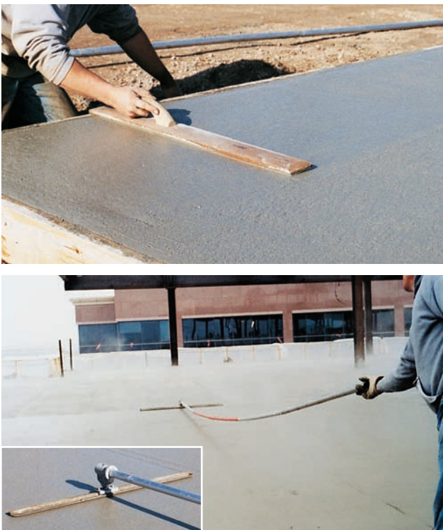
Figure 14-22. (top) Darbying brings the surface to the specified level and is done in tight places where a bullfloat cannot reach. (bottom) Bullfloating must be completed before any bleed water accumulates on the surface.
