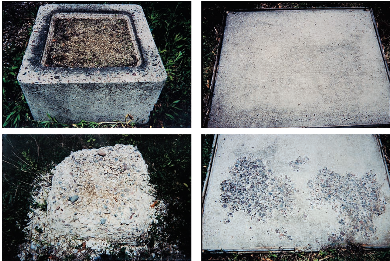
Figure 11-16. Effect of weathering on boxes and slabs on ground at the Long-Time Study outdoor test plot, PCA, Skokie, Illinois (Stark and others 2002). Specimens at top are air-entrained, specimens at bottom exhibiting severe crumbling and scaling are non air-entrained. All concretes were made with 335 kg (564 lb) of Type I portland cement per cubic meter (cubic yard). Periodically, calcium chloride deicer was applied to the slabs. Specimens were 40 years old when photographed (see Klieger 1963 for concrete mixture information).
