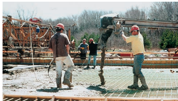
Figure 14-9. The swing arm on a conveyor belt allows fresh concrete to be placed evenly across a deck.
