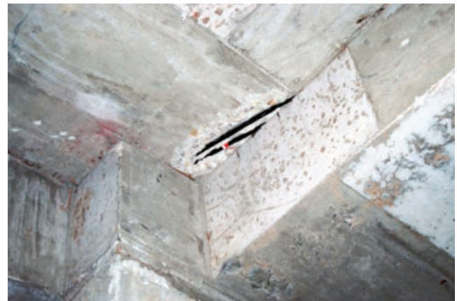
Figure 8-12. 'Blow-out' of post-tensioning tendon during stressing.
