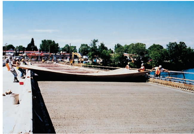
Figure 14-29. An excellent method of wet curing is to completely cover the surface with wet burlap and keep it continuously wet during the curing period.
