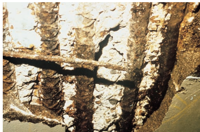
Figure 7-17. The damage to this concrete parking structure resulted from chloride-induced corrosion of steel reinforcement.
