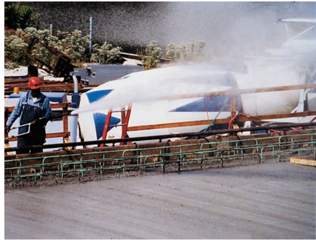
Figure 15-4. Fogging minimizes moisture loss during and after placing and finishing of concrete.
