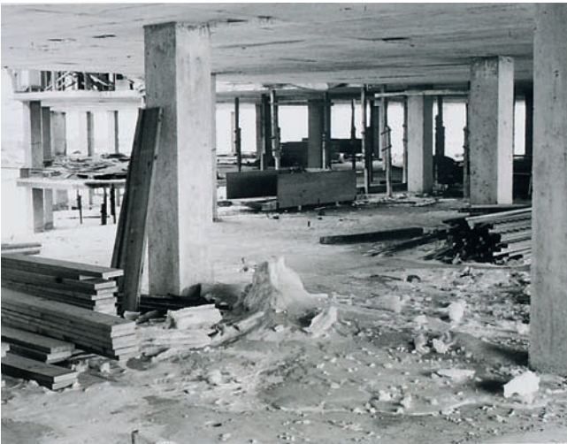
Figure 17-11. Example of a concrete floor that was saturated with rain, snow, or water and then frozen, showing the need for air entrainment.
