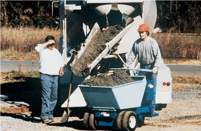
Figure 13-8. Versatile power buggy can move all types of concrete over short distances.
