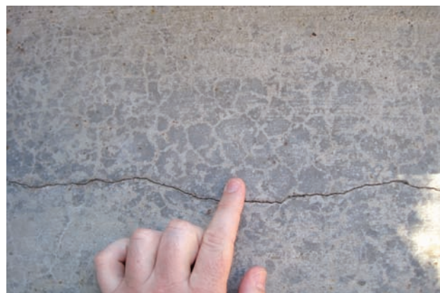
Figure 16-13. Crazing cracks are a network of fine cracks, compared to a flexural or tensile stress crack.
