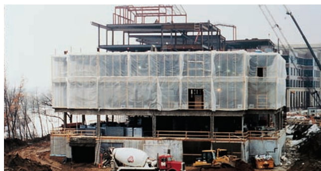
Figure 17-18. (top) Tarpaulin heated enclosure maintains an adequate temperature for proper curing and protection during severe and prolonged winter weather. (bottom) Polyethylene plastic sheets admitting daylight are used to fully enclose a building frame. The temperature inside is maintained at 10°C (50°F) with space heaters.
