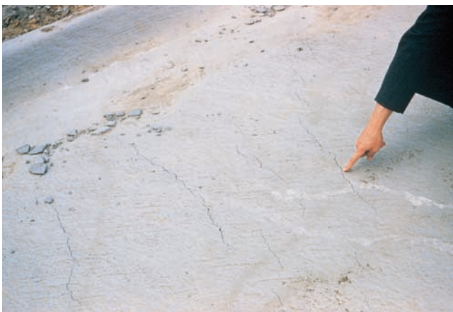
Figure 16-8. Typical plastic shrinkage cracks.
