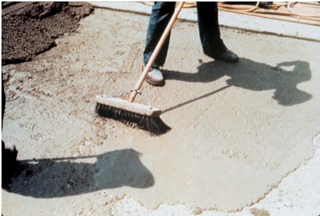
Figure 14-14. Application of a bonding grout just ahead of the overlay concrete. The grout must not dry out before the concrete is placed.
