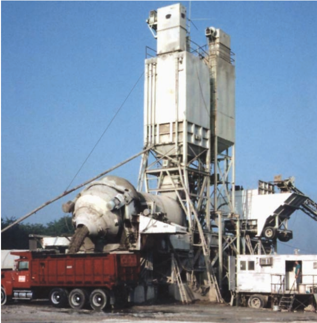
Figure 13-2. Concrete can be mixed at the jobsite in a stationary mixer (Courtesy of Baker Concrete).
