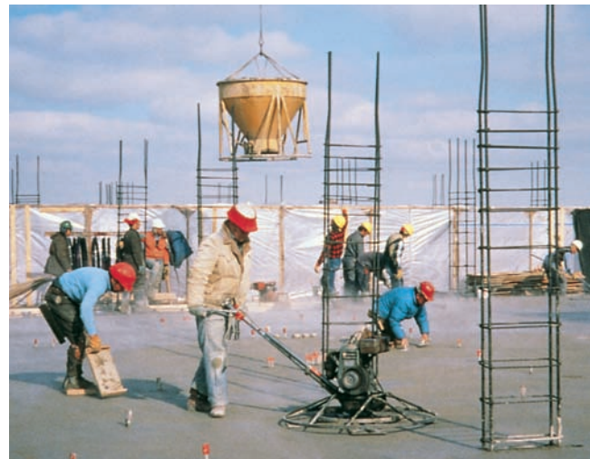
Figure 17-9. Finishing this concrete flatwork can proceed because a windbreak has been provided, there is adequate heat under the slab, and the concrete has low slump.
