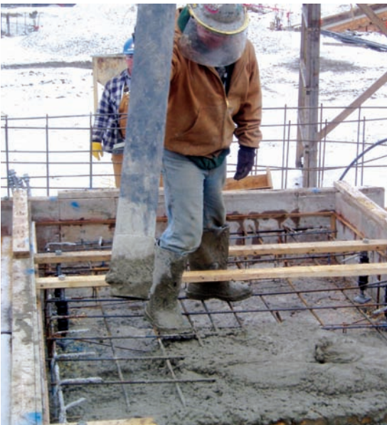
Figure 13-13. (top) A truck-mounted pump and boom can conveniently move concrete vertically or horizontally to the desired location. (bottom) View of concrete discharging from flexible hose connected to rigid pipeline leading from the pump. Rigid pipe is used in pump booms and in pipelines to move concrete over relatively long distances. Up to 8 m (25 ft) of flexible hose may be attached to the end of a rigid line to increase placement mobility (Bottom photo Courtesy of Baker Concrete).
