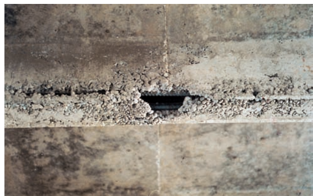
Figure 14-16. Honeycombs and rock pockets are the results of inadequate consolidation.
