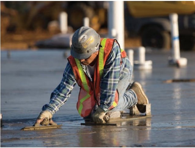
Figure 14-25. Hand floating (left hand) the surface with a hand float held flat on the concrete surface and moved in a sweeping arc with a slight sawing motion. Troweling (right hand) with blade tilted is performed before moving the kneeboards (Courtesy of Baker Concrete).
