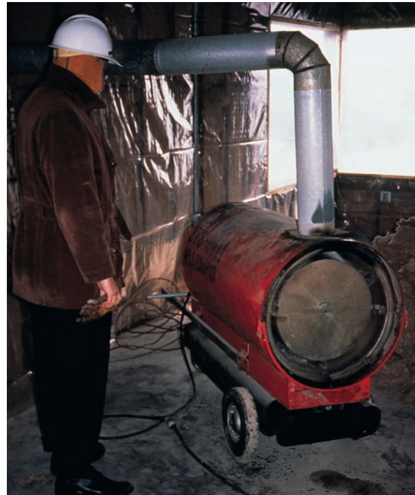
Figure 17-23. An indirect-fired heater. Notice vent pipe that carries combustion gases outside the enclosure.
