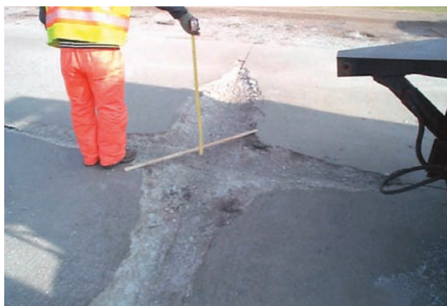
Figure 11-12. V-shaped joints are a common sign of the effects of freeze-thaw damage in concrete pavements. Some joints exhibit an inverted V-shaped deterioration (Courtesy of D. Harrington).
