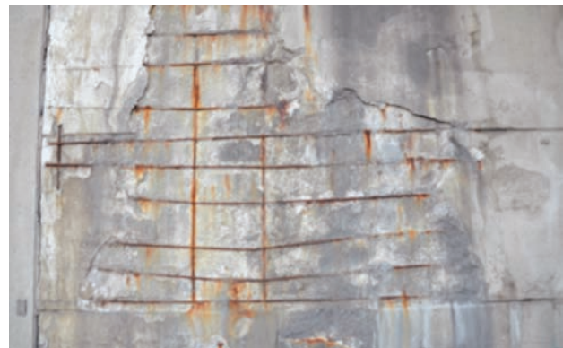
Figure 8-5. Reinforcing steel corrosion and concrete spalling due to reduced cover.
