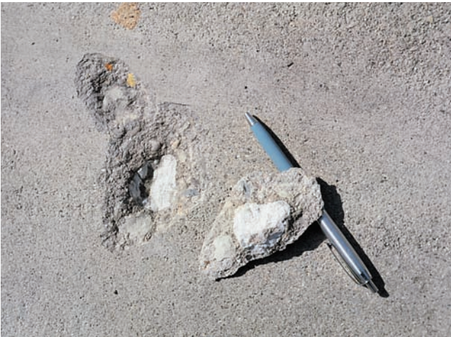
Figure 6-20. A popout is the breaking away of a small fragment of concrete surface due to internal pressure that leaves a shallow, typically conical depression.
