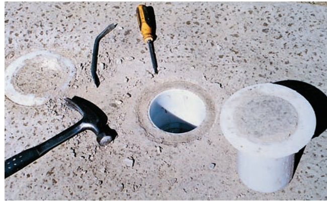
Figure 18-17. Concrete cylinders cast in place in cylindrical molds provide a means for determining the in-place compressive strength of concrete (ASTM C873/C873M).
