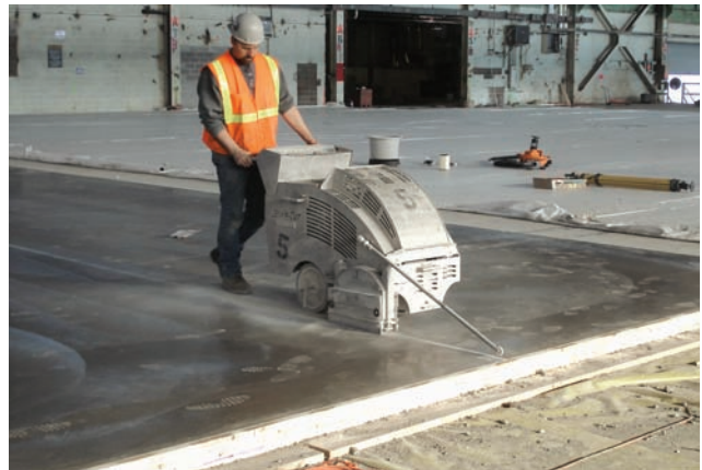
Figure 14-32. Sawing a continuous cut in the top of a slab is one of the most economical methods for making a contraction joint.
