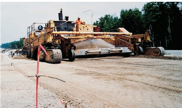
Figure 14-1. A base course foundation for concrete pavement is shaped by an auto-trimmer to design grades, cross section and alignment using automatic sensors that follow string lines.
