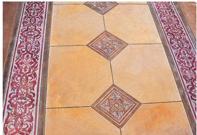
Figure 2-6. Decorative concrete flooring created using a sandblast stencil technique eliminates the need for carpeting or other flooring materials that can impair indoor air quality.
