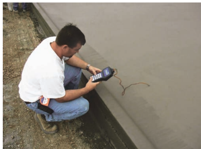
Figure 17-26. Downloading data from a maturity sensor embedded in a pavement.
