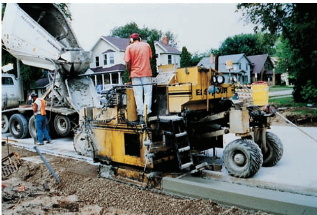
Figure 14-15. Curb machines continuously extrude low-slump concrete into a shape that immediately stands without support of formwork.
