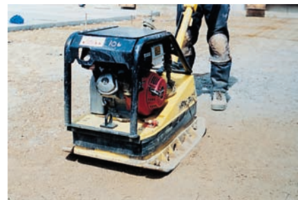
Figure 14-3. (top) Adequate compaction of a base course foundation for concrete pavement can be achieved by using a vibratory roller. (bottom) Vibratory plate compactors are also used to prepare subgrades under slabs.
