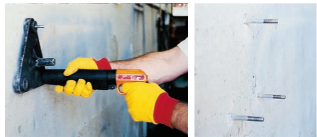
Figure 18-28. The Windsor-probe technique for determining the relative compressive strength of concrete. (left) Powder-actuated gun drives hardened alloy probe into concrete. (right) Exposed length of probe is measured and relative compressive strength of the concrete then determined from a calibration table.
