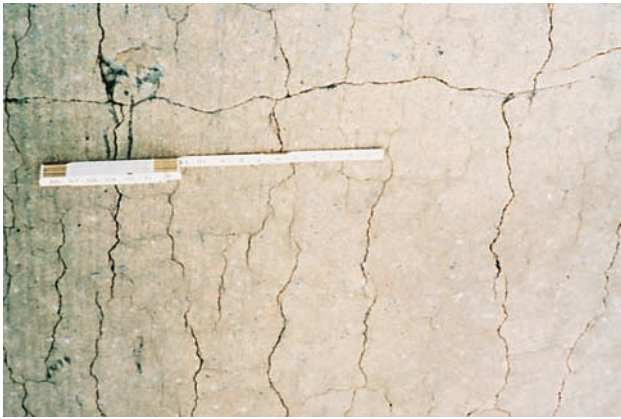
Figure 11-21. Indication of potential alkali-silica reaction is provided by the classic map cracks on the surface of the concrete. ASR should be verified by petrographic examination.
