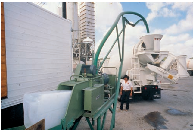
Figure 16-6. Substituting ice for part of the mixing water will substantially lower concrete temperature. A crusher delivers finely crushed ice to a truck mixer reliably and quickly.
