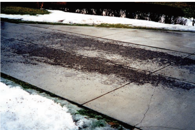
Figure 11-10. Severe scaling of a concrete pavement.
