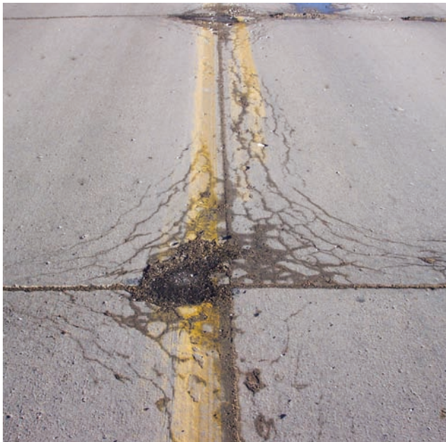
Figure 6-21. D-cracking along a transverse joint caused by failure of carbonate coarse aggregate (Courtesy of J. Grove).
