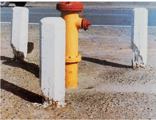
Figure 11-35. Salt crystallization attack is often observed near the soil line. Here concrete posts have been attacked by sulfate salts near the soil line.
