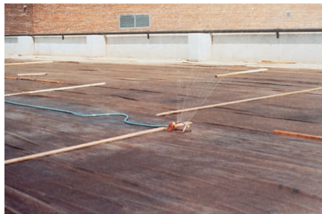
Figure 15-5. Lawn sprinklers saturating burlap with water keep the concrete continuously moist. Intermittent sprinkling is acceptable if no drying of the concrete surface occurs.
