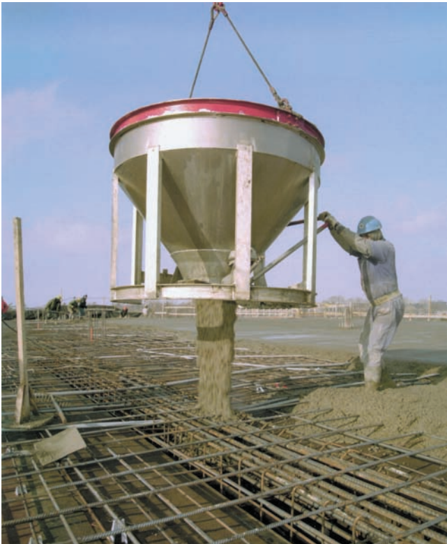
Figure 13-9. Concrete is easily lifted to its final location by bucket and crane.
