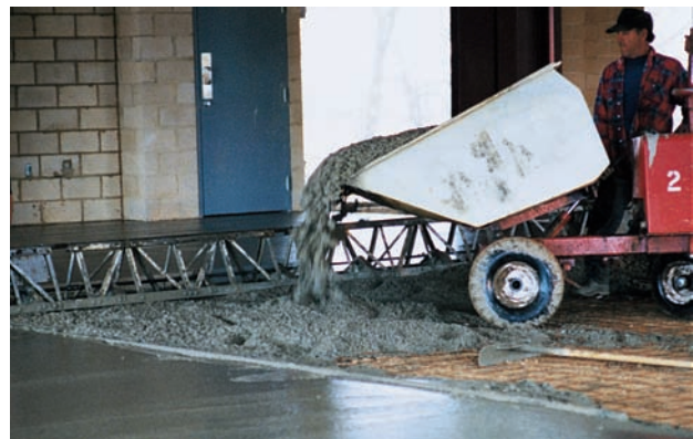
Figure 14-8. Concrete should be placed as near as possible to its final position.
