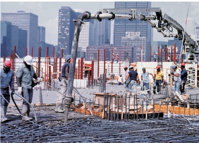
Figure 13-19. A pump boom mounted on a mast and located near the center of a structure can frequently reach all points of placement. It is especially applicable to tall buildings where tower cranes cannot be tied up with placing concrete. Concrete is supplied to the boom through a pipeline from a ground-level pump. Concrete can be pumped hundreds of meters (feet) vertically with these pumping methods.
