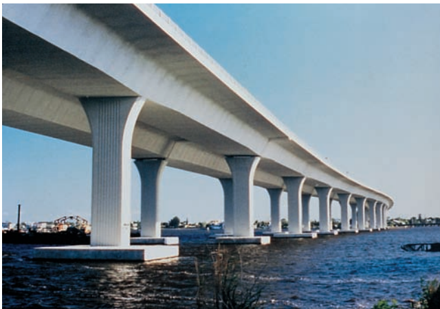
Figure 11-38. Concrete exposed to a marine environment.
