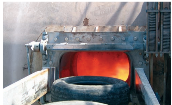
Figure 3-13. Whole rubber tires introduced directly into the kiln by conveyor as an alternative fuel.
