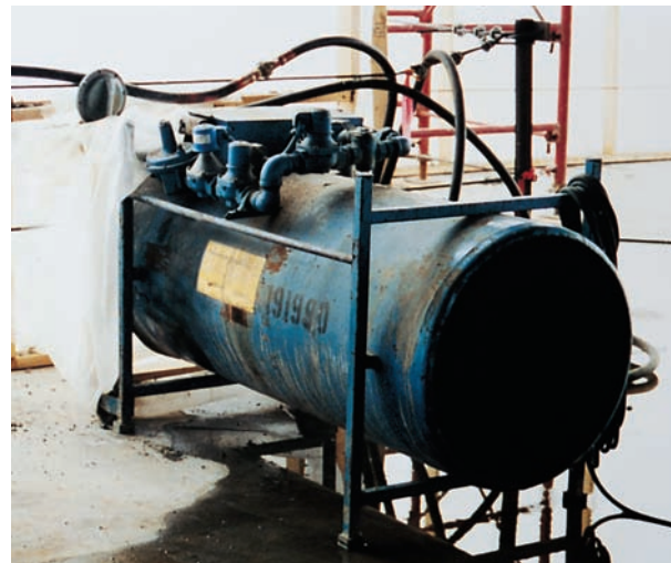
Figure 17-24. A direct-fired heater installed through the enclosure, thus using a fresh air supply.
