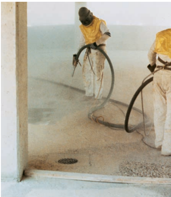
Figure 14-13. Sandblasting can clean any size or shape surface – horizontal, vertical, or overhead. Consult local environmental regulations regarding sandblasting.
