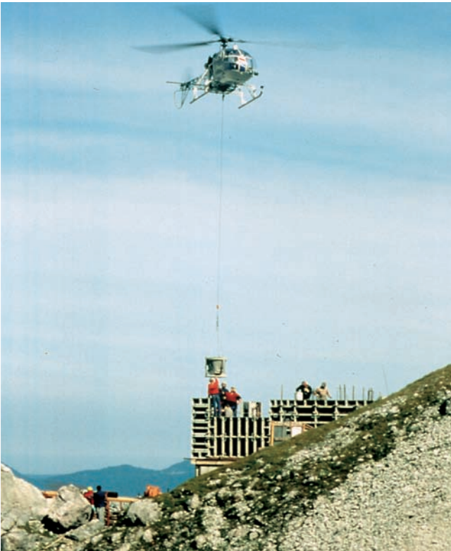
Figure 13-18. For work aboveground or at inaccessible sites, a concrete bucket can be lifted by helicopter (Courtesy of Paschal).
