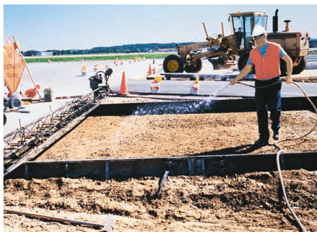
Figure 16-10. Dampening the subgrade, yet keeping it free of standing water will lessen drying of the concrete and reduce problems from hot weather conditions.
