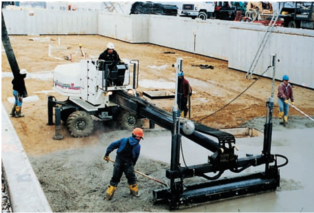
Figure 14-21. A laser level striking the sensors on this screed guides the operator as he strikes off the concrete. Screed poles and chairs are not needed and fewer workers are required to place concrete. Laser screeds interfaced with total station surveying equipment can also strike off sloped concrete surfaces.
