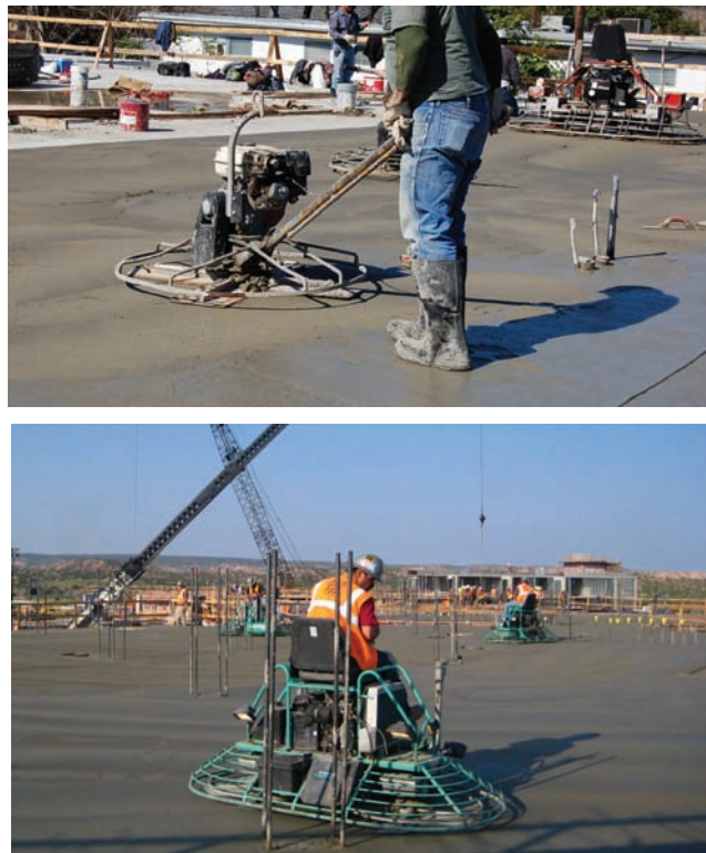
Figure 14-24. Power floating using walk-behind (top) and ride-on equipment (bottom). Footprints indicate proper timing. When the bleedwater sheen has evaporated and the concrete will sustain foot pressure with only slight indentation, the surface is ready for floating and final finishing operations (Courtesy of Baker Concrete).
