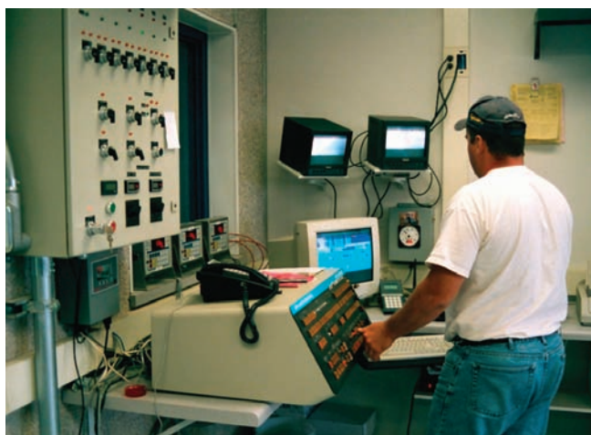
Figure 13-1. Batch control room in a typical ready mixed concrete plant.
