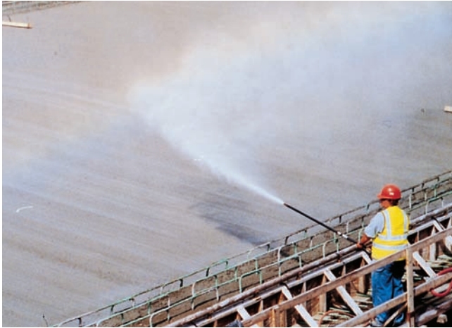
Figure 16-11. Fogging cools the air and raises the relative humidity above flatwork to lessen rapid evaporation from the concrete surface, thus reducing cracking and improving surface durability.
