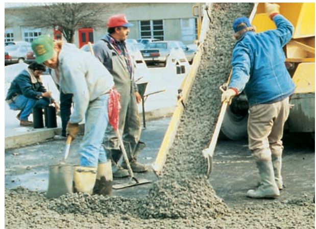
Figure 13-10. Ready mixed concrete is often placed in its final location by direct chute discharge from a truck mixer.
