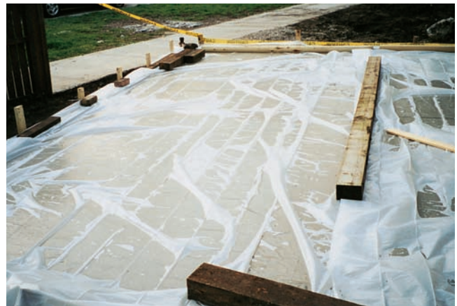
Figure 15-7. Polyethylene film is an effective moisture barrier for curing concrete and easily applied to complex as well as simple shapes. To minimize discoloration, the film should be kept as flat as possible on the concrete surface.
