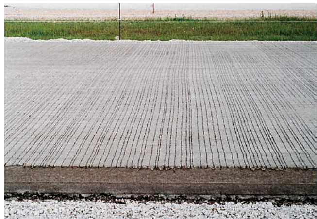
Figure 14-27. (top) This machine is tining the surface of fresh concrete. (bottom) Tining of pavements improves tire traction and reduces hydroplaning.
