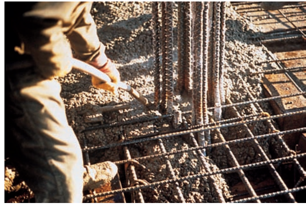
Figure 14-17. Proper vibration makes possible the placement of stiff concrete mixtures, even in heavily-reinforced concrete members.
