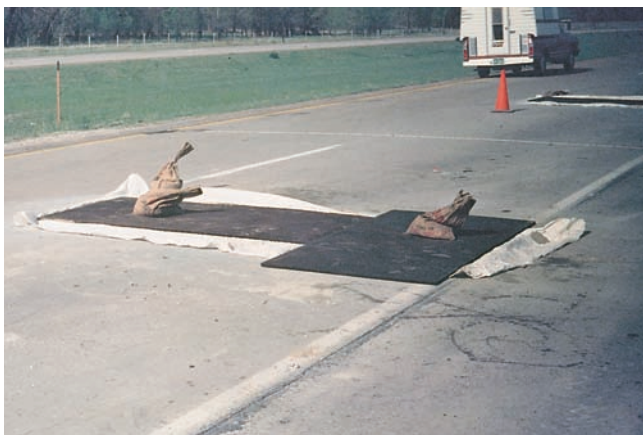
Figure 14-39. Good curing is essential to successful patching. This patch is covered with polyethylene sheeting plus rigid insulation to retain moisture and heat for rapid hydration and strength gain.
