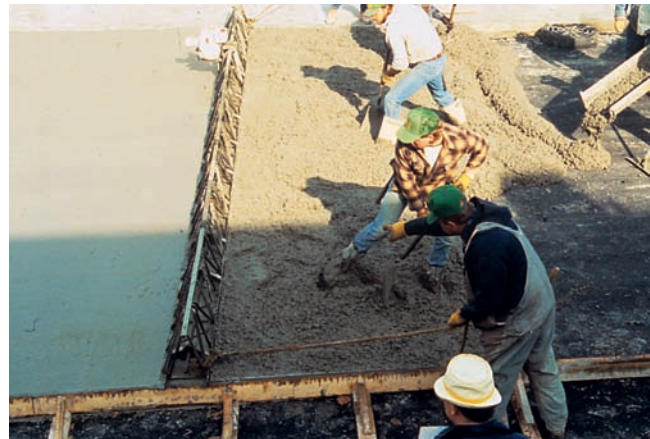
Figure 14-19. Vibratory screeds such as this truss-type unit reduce the work of strikeoff while consolidating the concrete.
