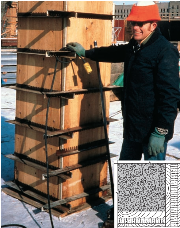
Figure 17-21. With air temperatures down to -23^{\circ}\text{C} ( -10^{\circ}\text{F} ), concrete was cast in this insulated column form made of 19-mm ( 3/4 -in.) high-density plywood inside, 25-mm (1-in.) rigid polystyrene in the middle, and 13-mm ( 1/2 -in.) rough plywood outside. R value: 1.0\text{ m}^2 \cdot ^{\circ}\text{C}/\text{W} ( 5.6\text{ [}^{\circ}\text{F} \cdot \text{hr} \cdot \text{ft}^2\text{)]}/\text{Btu} ).
