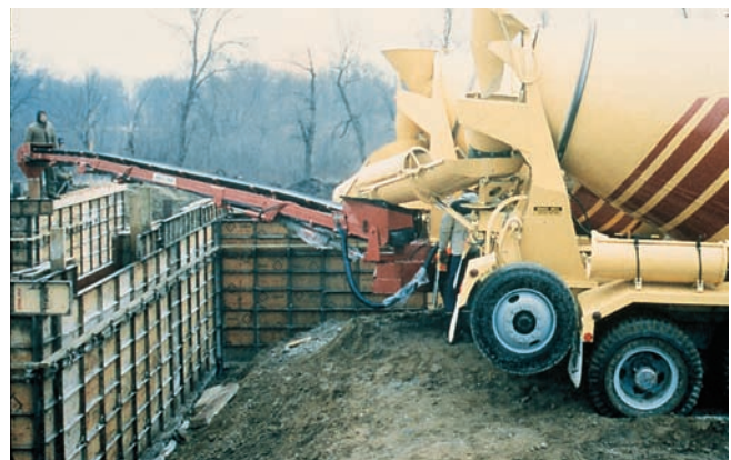
Figure 13-15. A conveyor belt mounted on a truck mixer places concrete up to about 12 meters (40 feet) without the need for additional transporting equipment.
