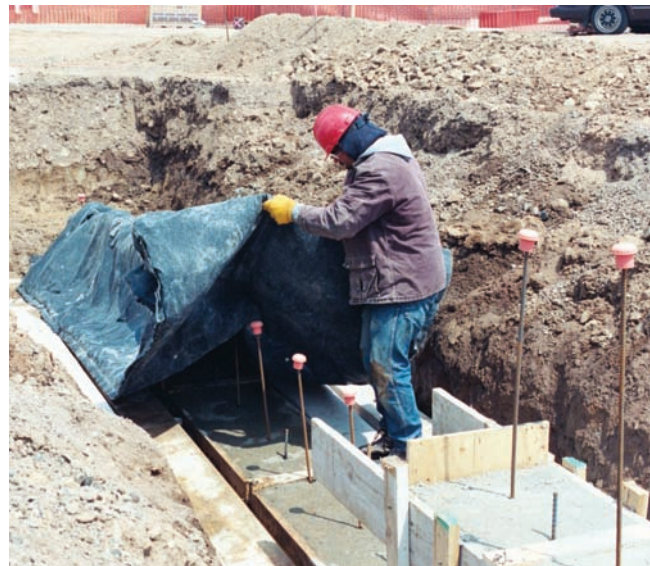
Figure 17-7. Concrete footing pedestal being covered with a tarpaulin to retain the heat of hydration.
