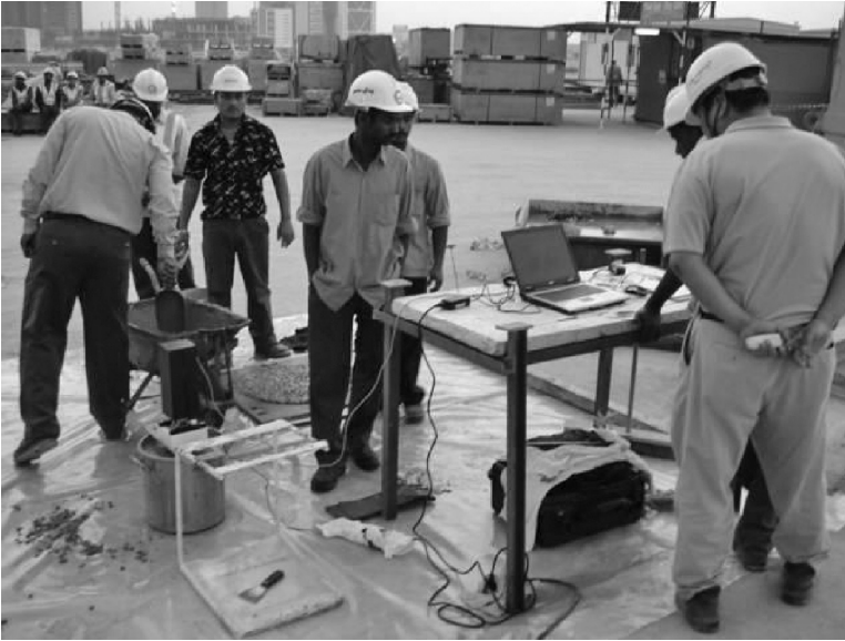
Figure 7.7 The ICAR rheometer being used for rheology measurement on Burj Khalifa project.
