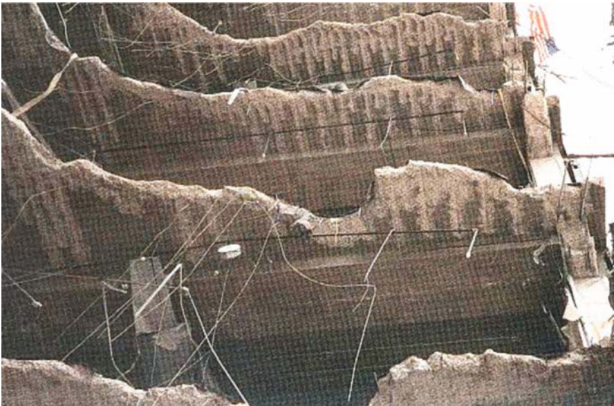
Fig. 10.36. Progressive collapse (courtesy: FEMA, Washinton D.C., U.S.A. – private communication)
