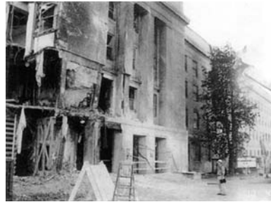
(c) Exterior evidence of fire to the south of the impact area
