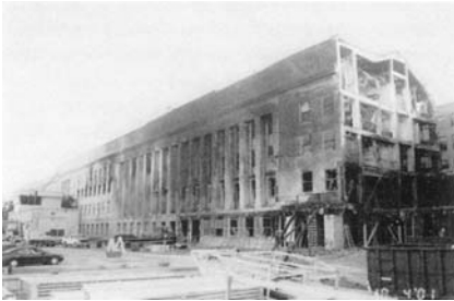
(b) Exterior evidence of fire to the north of the impact area
