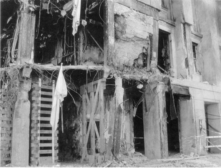
(a) Façade damage to the south of impact area
