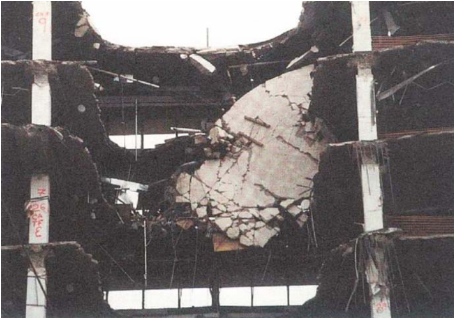
Fig. 10.35. Progressive collapse of the Murrah Building
