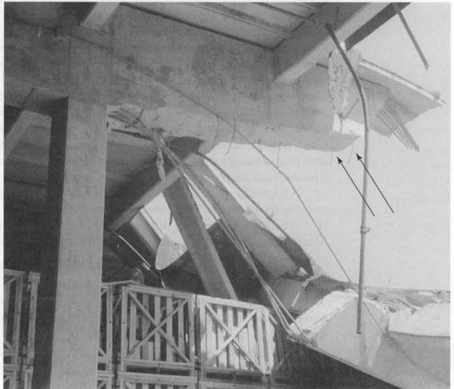
Fig. 6-2 Shear failure: U.S. Air Force warehouse. Note the small size and large spacing of the vertical web reinforcement that has fractured. (Photograph courtesy of C. P. Siess.)
