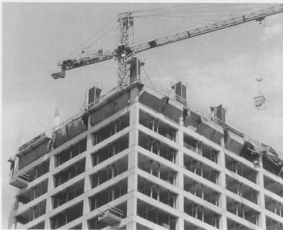
Fig. 10-3 Construction of columns in a tall building. (Photograph courtesy of J. G. MacGregor.)
