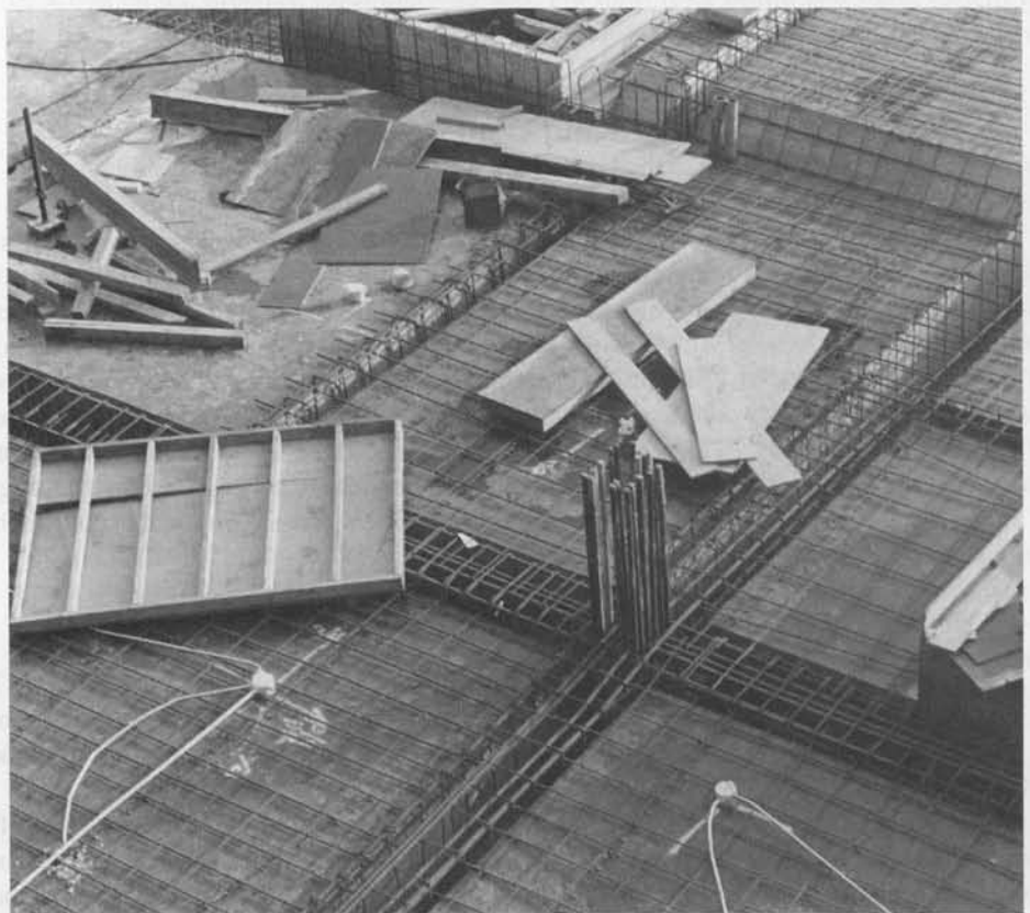
Fig. 10-2 Beam and slab reinforcement in the forms. (Photograph courtesy of J. G. MacGregor.)
