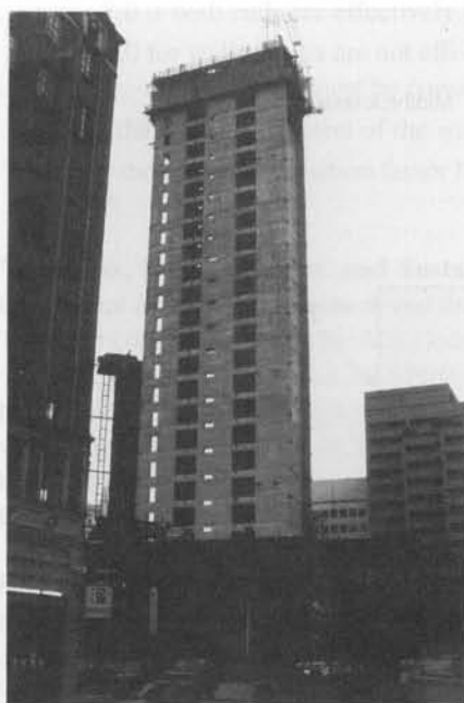
Fig. 18-2 Wall assembly in a building under construction. (Photo- graph courtesy of J.K.Wight.)
