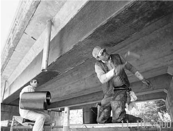
FIGURE 5.13 Preparations for wrapping the beam bottom with CFRP fabrics (Muddy Creek Bridge, West Virginia).
