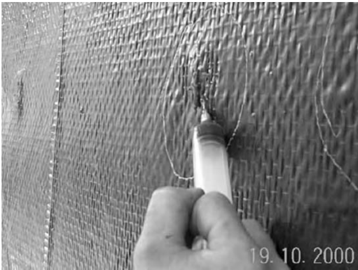
FIGURE 5.14 Removal of air entrapment from the bonded CFRP fabric (Muddy Creek Bridge, West Virginia).
