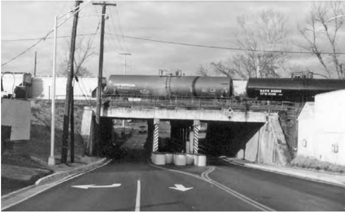
FIGURE 5.3 View of the viaduct with a train running on top (East Street Viaduct, West Virginia).
