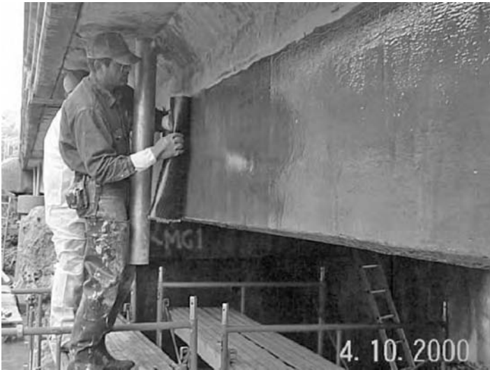
FIGURE 5.12 Wrapping of the beam side with CFRP fabrics (Muddy Creek Bridge, West Virginia).
