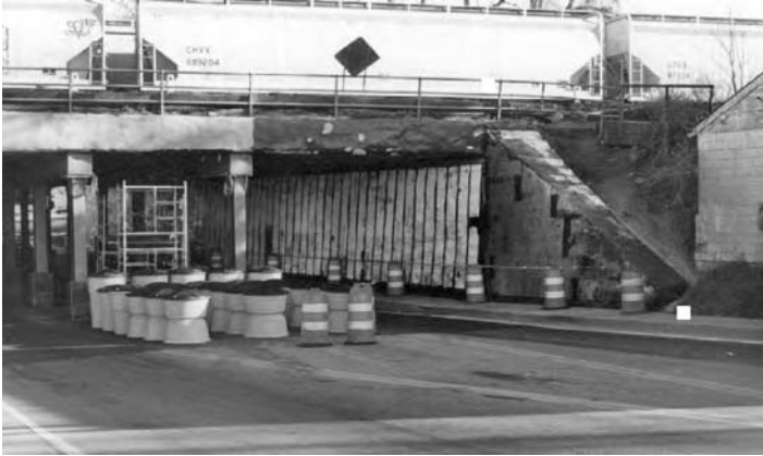
FIGURE 5.5 View of the wing wall and concrete girder being restored with GFRP fabric and the abutment wall with moisture-trap channels (East Street Viaduct, West Virginia).
