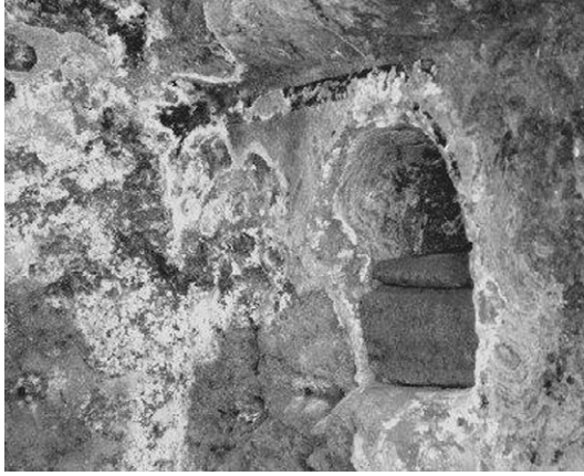
FIGURE 5.5 Salting on the internal walls of the tomb of Servilia, Carmona, Spain.
