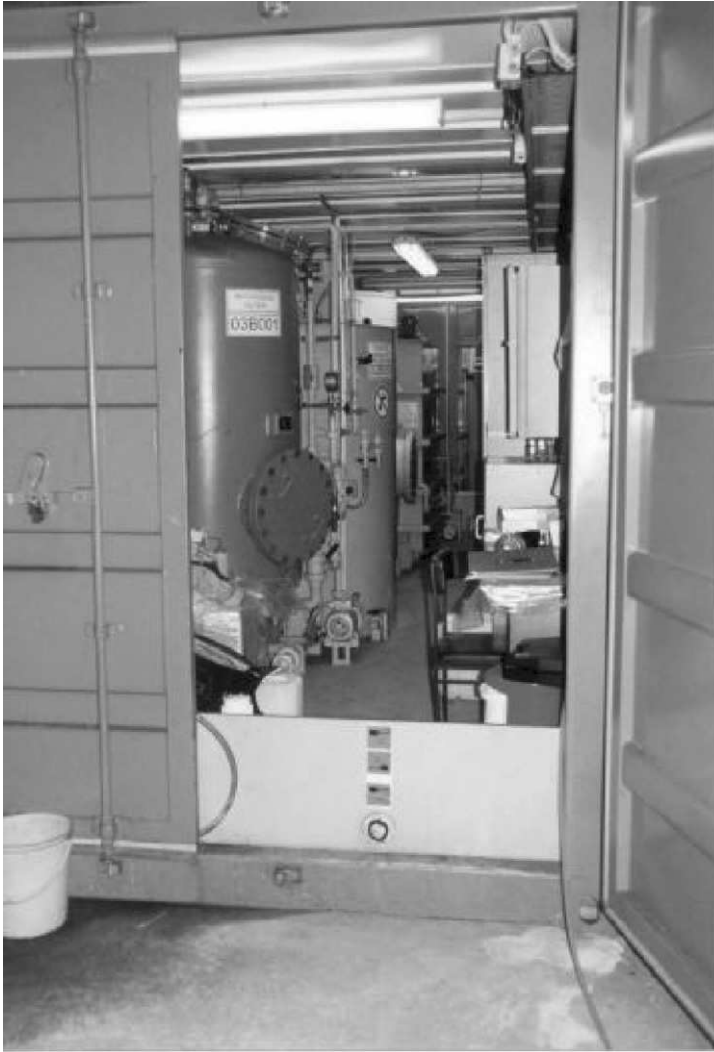
FIG. 4. View of the pilot plant for microbial cleanup of mercury-contaminated wastewater. The plant is located inside a blue standard container ( 2.5 \times 2.5 \times 9 m). On the left side, carbon filter, bioreactor, and pH adjustment tank can be seen. On the right side are the mercury monitors and the computer for data collection, online monitoring, and control. The volume of the bioreactor is 1 \text{ m}^3 . Photograph from Dr. Irene Wagner-Döbler.
