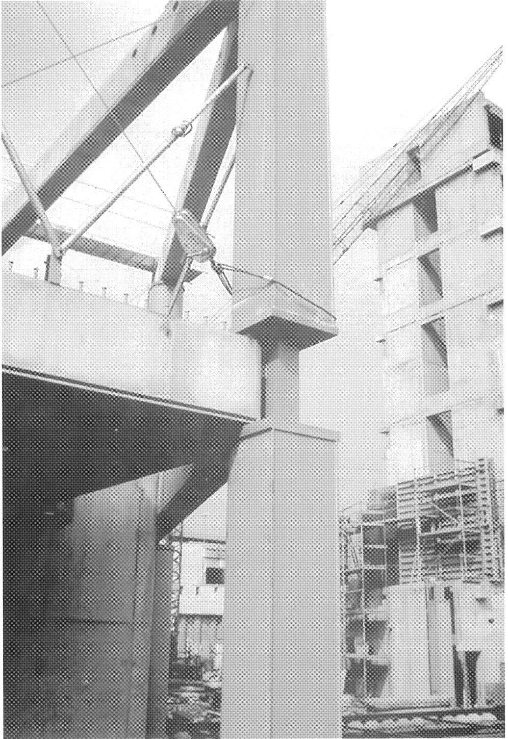
Connection of a composite beam to a concrete filled hollow section column. Loads from the upper column are transduced by a massive steel block to the lower column. The beam is simply laid upon the headplate of the lower column.
