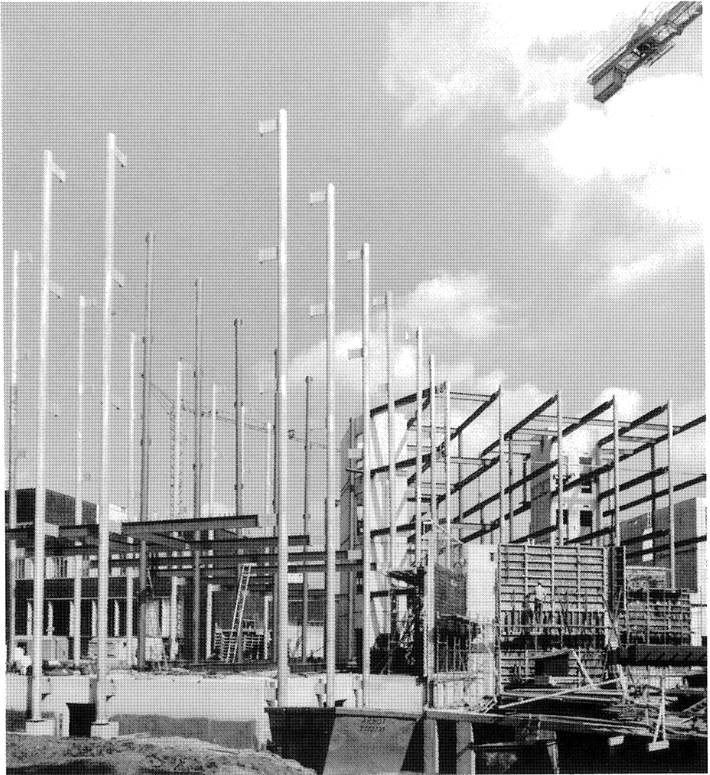
Concrete filled circular hollow section columns for the new VDEh-building in Düsseldorf, Germany.
