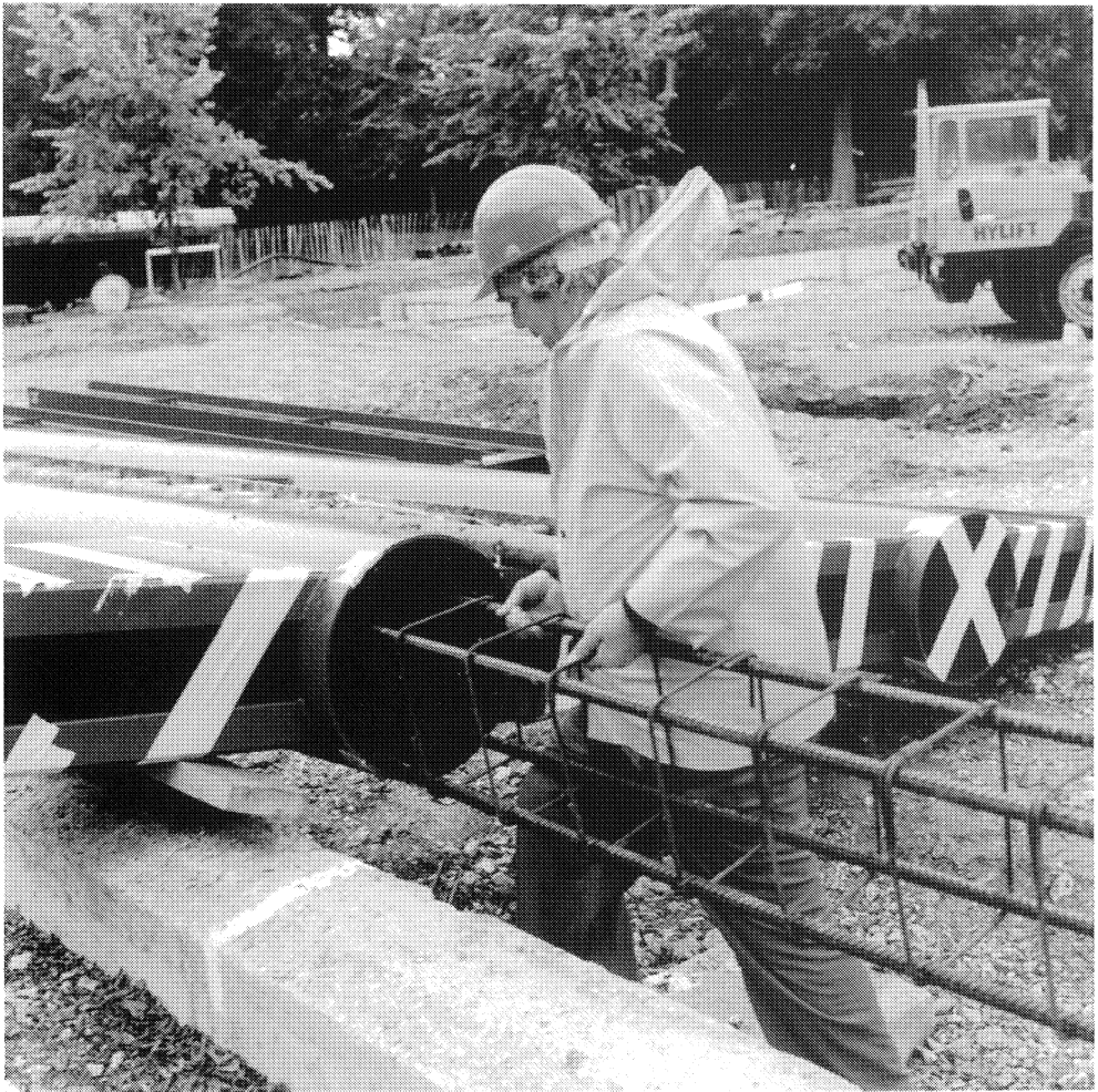
Introducing reinforcement bars before concrete filling (especially increasing the fire resistance time).
