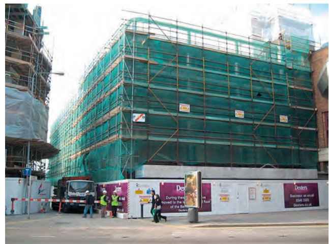
Figure 7.7 Protection of the public in main shopping area
