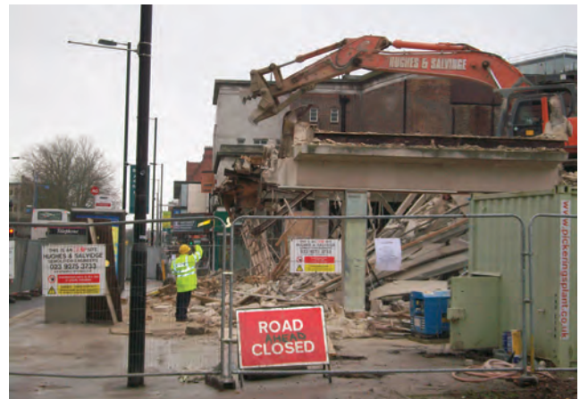
Figure 18.6 Demolition site should be well planned and properly signed and controlled throughout the project
