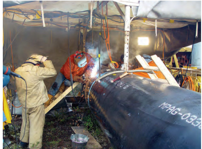
Figure 4.25 A hot work permit is usually essential for welding, cutting and burning except in designated areas like a welding shop
