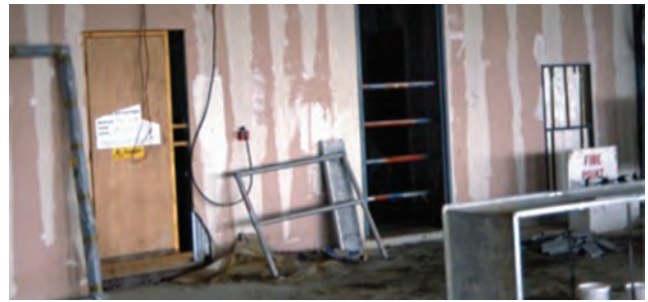
Figure 13.19 Plasterboard partitions such as this can form effective compartmentation. It is important that all gaps are filled in. In this case, there are holes in the top of the partition and service ducts in the side rooms that need to be sealed
