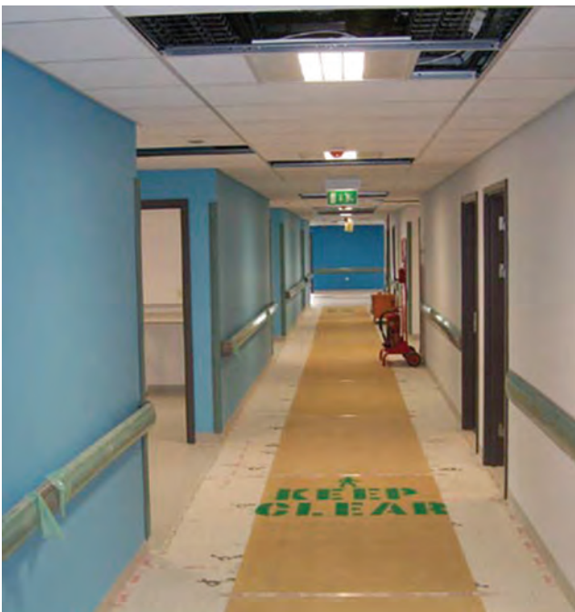
Figure 13.26 Fire escape route clearly signed and free from obstructions
