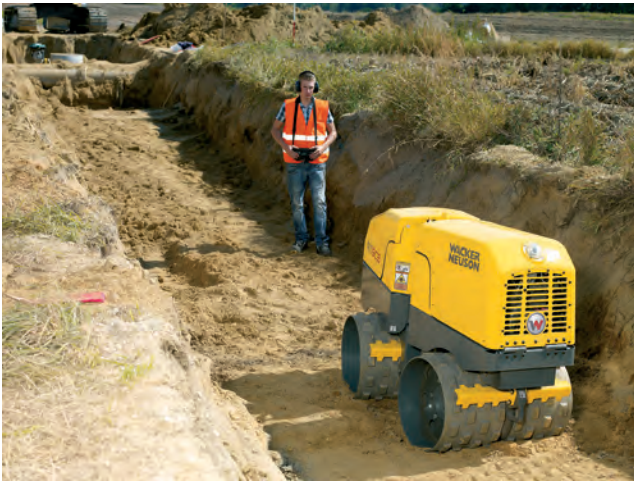
Figure 11.36 (b) Ground consolidating roller using remote control which eliminates the whole-body vibration exposure of the operator
