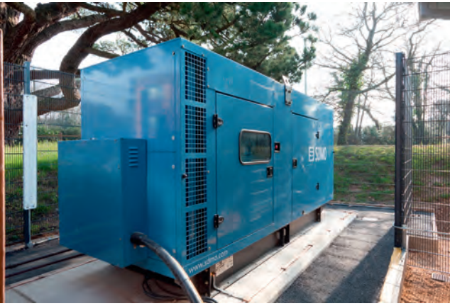
Figure 11.40 Larger transportable diesel-powered electric generator in an enclosure
