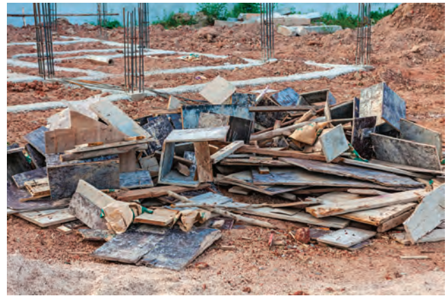
Figure 3.7 Most construction rubbish can burn. Make sure that it is swept up and removed from the site as soon as possible
