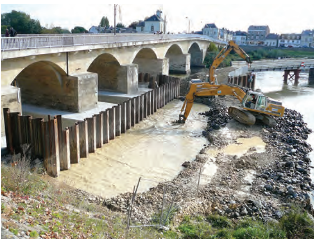
Figure 17.4 (b) Cofferdam built for repairing bridge piers in a river to be removed after construction completed
