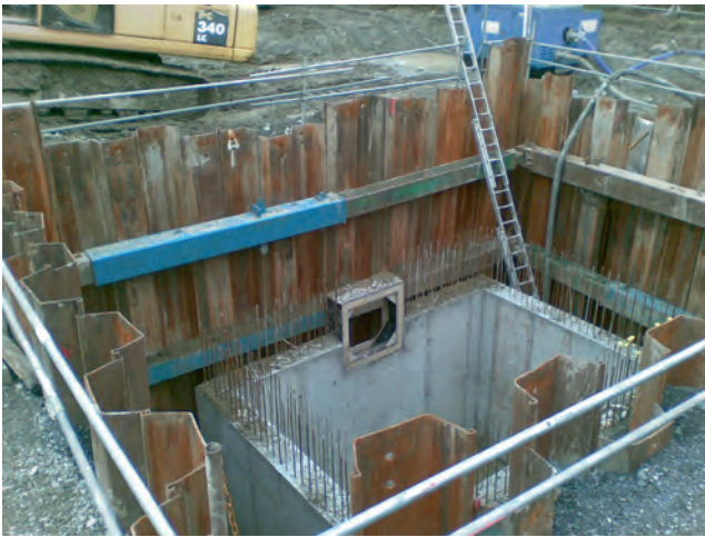
Figure 17.4 (a) Cofferdam for building a below-ground shaft and concrete tank – cofferdam removed and backfilled after construction
