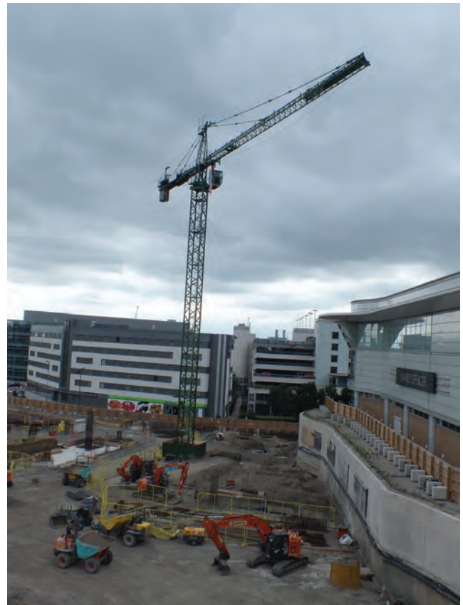
Figure 7.6 (b) Large site (over 30 days, more than 20 workers simultaneously or exceeds 500 person days): CDM applies and client must notify the relevant enforcing authority
