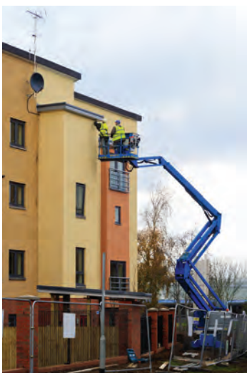
Figure 16.17 Mobile elevating work platform (MEWP) – cherry picker with harness and lanyard attached to cradle
