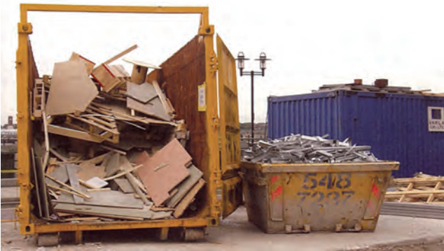
Figure 14.21 A designated waste collection area with two types of skip commonly used for waste collection. Heavy materials would be transported in the smaller skip. Sizes of skip range from about 4 cu metres (small skip shown) to about 35 cu metres (large skip shown)
