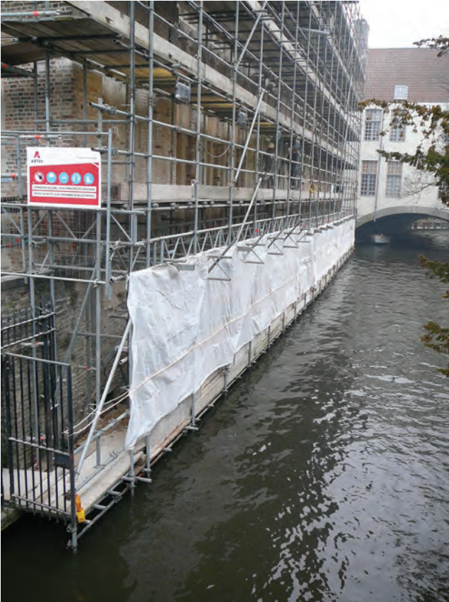
Figure 16.21 Working over or near water – large scaffold with protection screens and a small boat moored under the bridge in case rescue is needed
