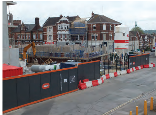
Figure 8.3 Secure site access gate with added protection to prevent vehicles entering at night or on Sundays
