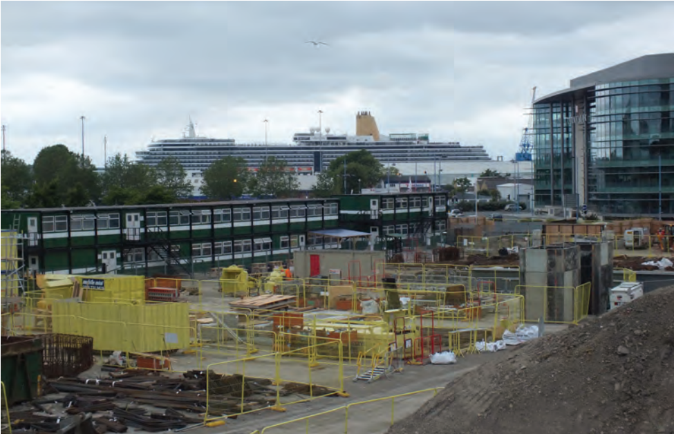
Figure 8.5 Well organised site with internal storage compounds and site accommodation behind with means of escape staircase in case of fire (also from the UK, in background on Southampton water)
