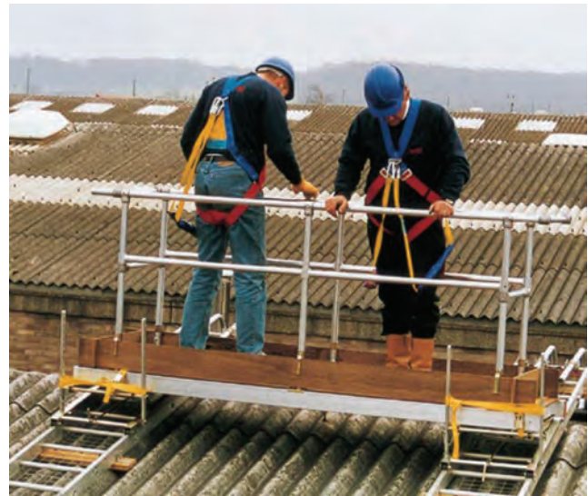
Figure 16.4 Proper precautions should always be taken when working on or near fragile roofs – access system for short-term work
