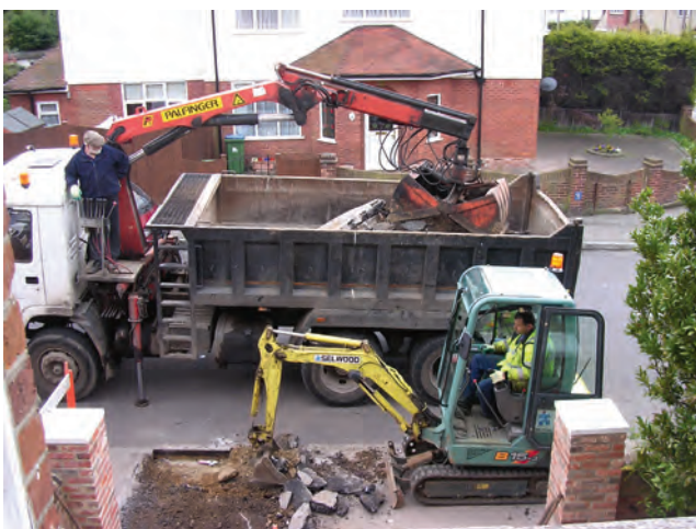
Figure 7.6 (a) Domestic client: CDM applies but only a short duration contract, no notification required – would be notifiable if a large project
