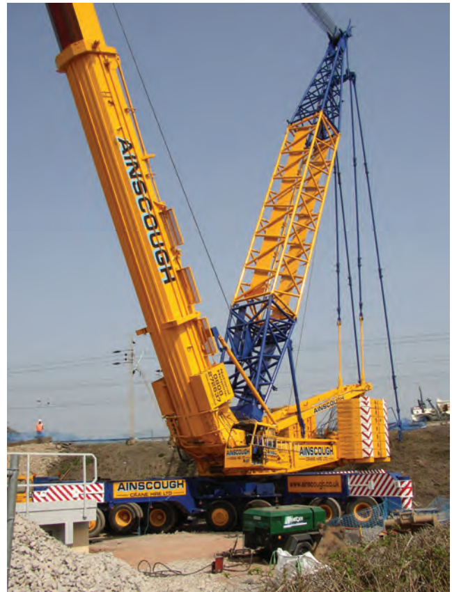
Figure 9.12 Occupational road risk increases when construction work is undertaken – cranes like this have to be driven to their operating location and operated when on site
