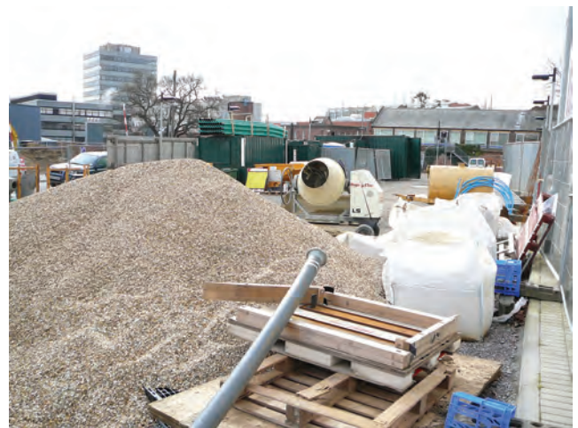
Figure 8.12 Tripping hazards on untidy site
