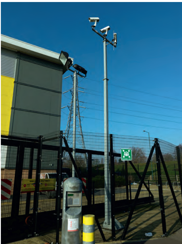
Figure 8.10 Security access and surveillance CCTV camera
