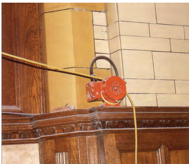
Figure 13.22 A temporary wired-in fire alarm during major renovation of a large and multi-storey complex building
