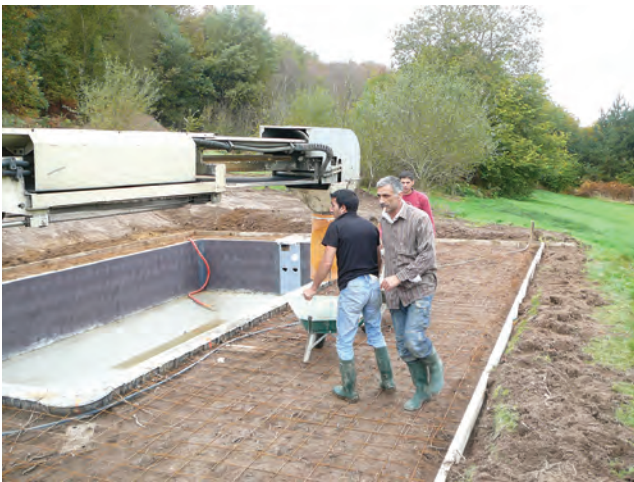
Figure 7.3 Recent migrant workers, whose standards may not match those in Europe, are employed in the UK and the EU in general. In this instance, language was a problem, hard hats and gloves would have helped, boots were good protection but not steel-toed. Concrete delivery equipment was very up to date
