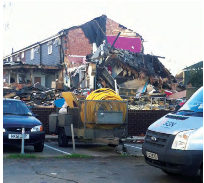
Figure 20.10 Gas explosion during the night in Southampton 2015 – two people escaped unhurt
