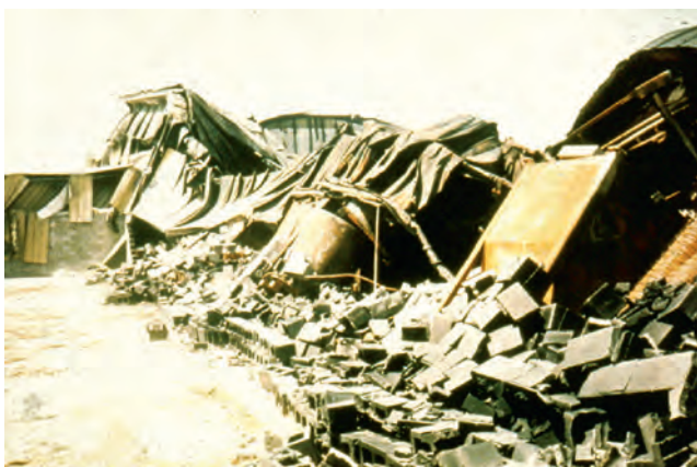
Figure 13.17 Steel structures can collapse in the heat of a fire
