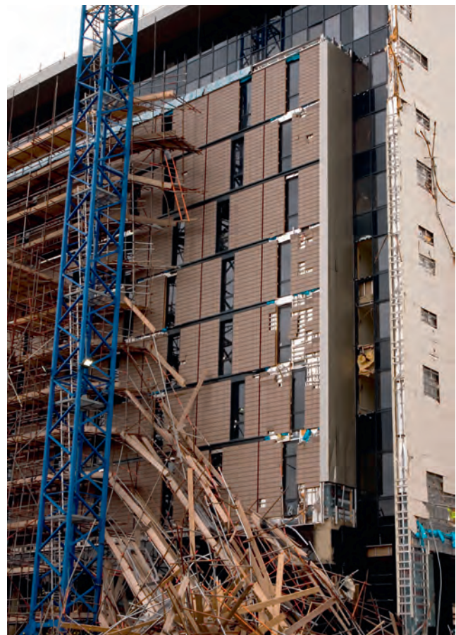
Figure 22.6 Scaffold collapse, Milton Keynes
