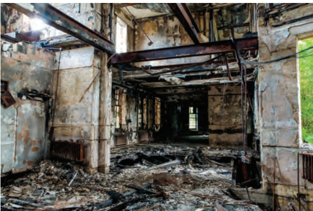
Figure 5.5 Dangerous occurrence: aftermath of a fire
