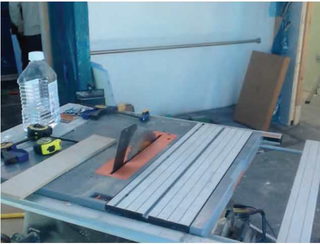
Figure 7.4 A serious accident waiting to happen on a small building site: no top guard on the circular saw – a very common safety fault
