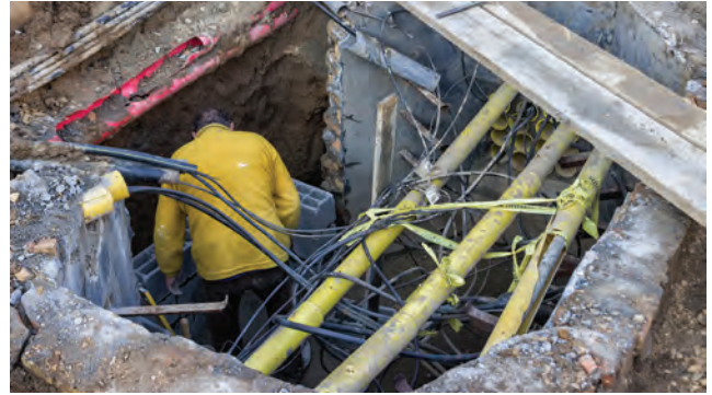
Figure 13.14 Electrical cabling can often get damaged and overloaded during a construction project. Other poor features here include: lack of head protection; confined space entry; edge protection and trench supports
