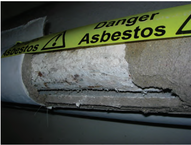
Figure 14.17 Damaged asbestos lagging on pipework
