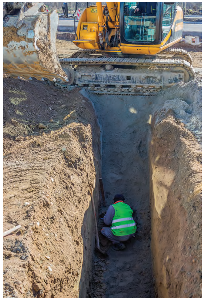
Figure 17.1 A very hazardous situation for the worker with a deep trench, a heavy machine very close to the edge and no trench supports
