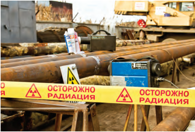
Figure 15.9 X-ray generating unit used for weld testing on site in Russia. The tape states: 'beware of radiation' (shows the value of pictorial signs)
