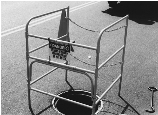
FIGURE 7.15 A typical confined space with a barrier and warning sign
