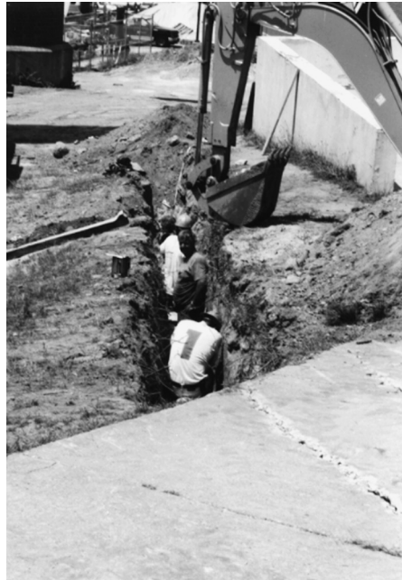
FIGURE 7.34 Workers in an unprotected trench
