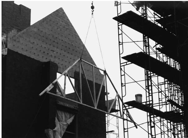
FIGURE 8.24 Example of wire rope slings being used
