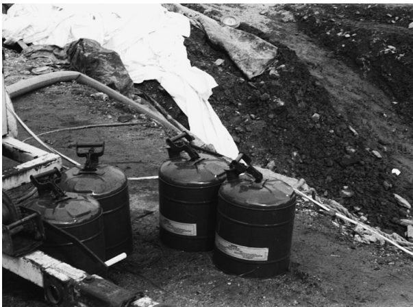
FIGURE 7.53 Containers for flammable or combustible liquids
