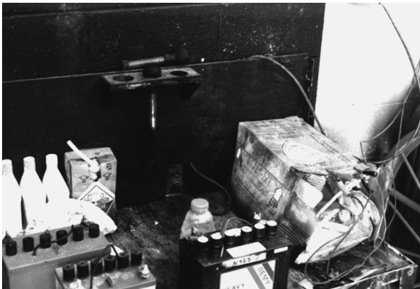
FIGURE 7.7 Poorly designed battery charging area
