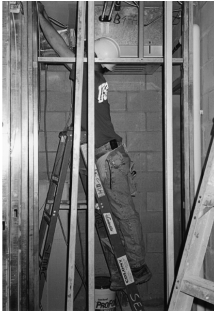
FIGURE 11.9 Electrician in a work position which causes him to have to raise his arms above his shoulders
