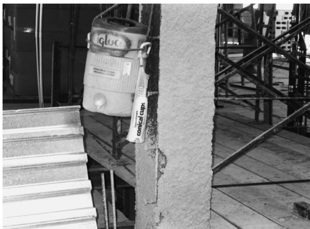
FIGURE 8.14 Potable water container with disposable cups
