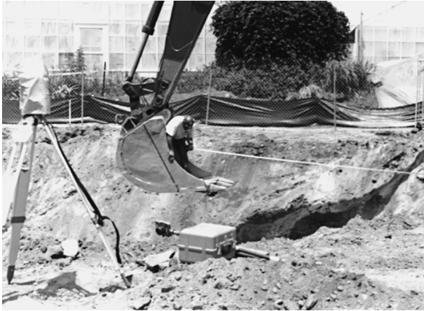
FIGURE 1.8 Unsafe act — worker riding in bucket
