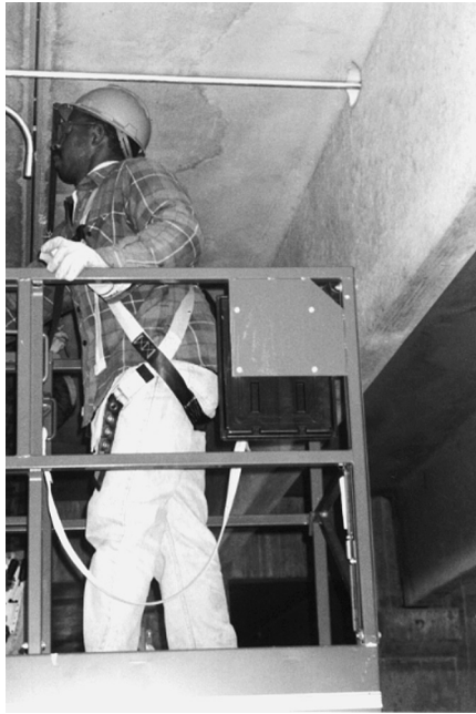
FIGURE 7.48 Personal fall protection system
