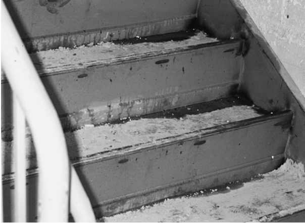
FIGURE 8.43 Unfilled stair pans create a real slip/trip/fall hazard
