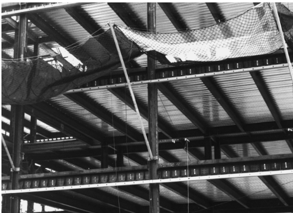
FIGURE 7.47 Example of a perimeter safety net
