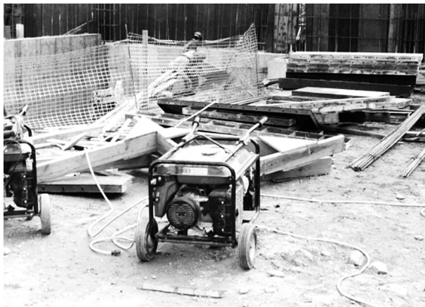
FIGURE 7.29 Example of portable electrical generator
