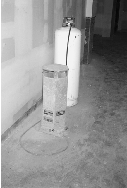
FIGURE 7.59 Example of a temporary heater
