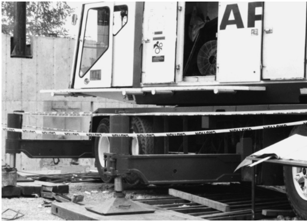
FIGURE 7.20 Crane with outrigger deployed and warning barriers
