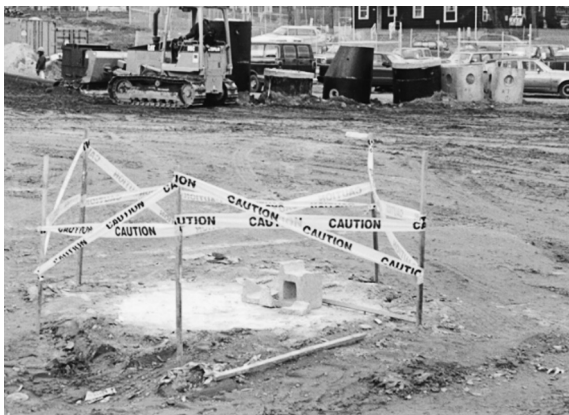
FIGURE 7.6 A barrier marked with caution tape
