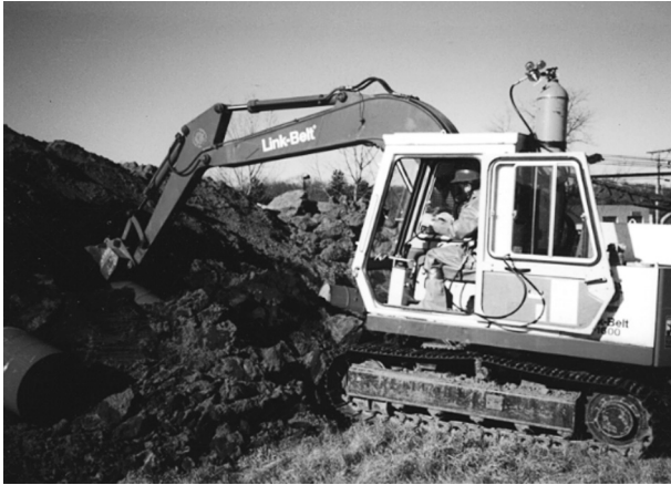
FIGURE 10.17 Site clean-up clothing is dependent on the hazards anticipated. Courtesy of the Operating Engineers, Local #478, Meriden, CT
