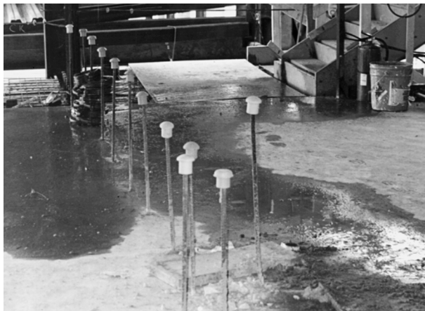
FIGURE 7.10 Protected rebar to guard against impalement
