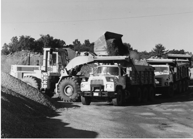
FIGURE 8.49 Dangers due to loading and movement of truck traffic frequently occur on construction Sites
