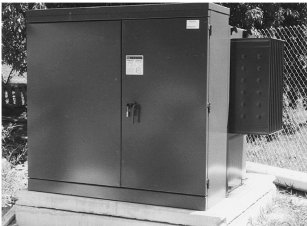
FIGURE 7.25 Electrical enclosure accessible to qualified persons
