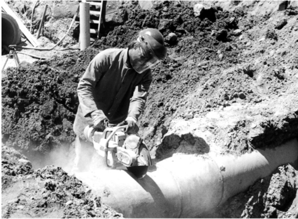
FIGURE 9.18 Cutting pipe could generate dust containing asbestos
