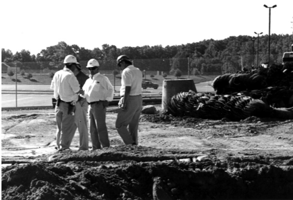
FIGURE 18.4 The contractor's presence and communication demonstrate his or her commitment to a safe and productive construction site
