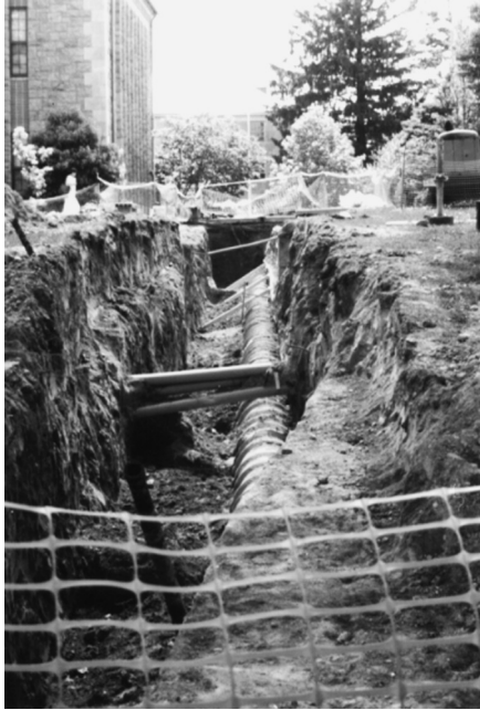
FIGURE 7.35 Unsupported trench and underground installations
