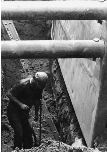
FIGURE 7.39 Worker using a trench box as a shield with a ladder for egress
