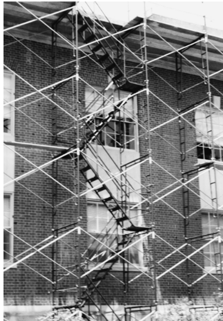
FIGURE 8.35 Built-in scaffold access ladders
