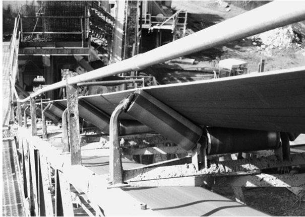
FIGURE 7.19 Example of conveyor hazards with some guarding
