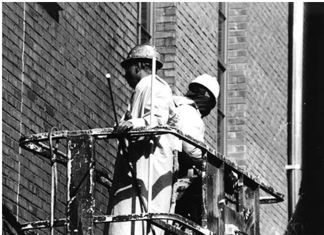
FIGURE 9.21 Cleaning buildings with high pressure chemicals may generate hazardous mists or vapors
