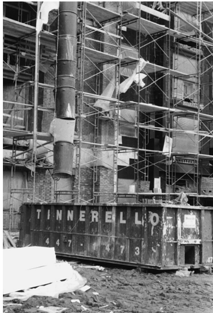
FIGURE 7.23 Enclosed disposal chute on exterior of building
