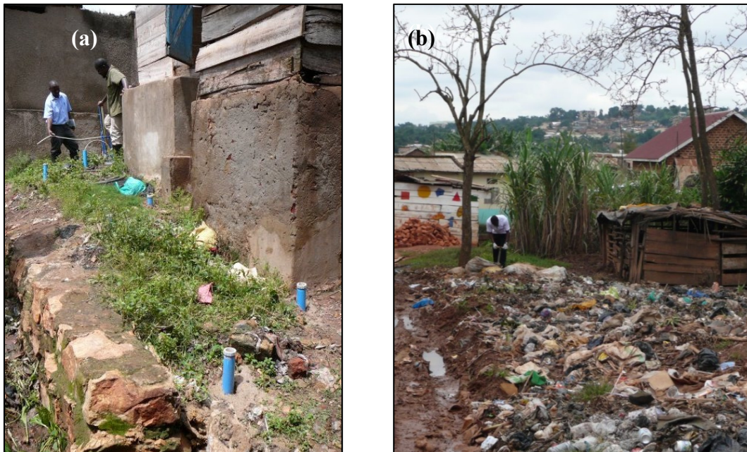
Figure 4.3: Installation of the monitoring wells at (a) the pit latrine site and (b) the solid waste dump site.
