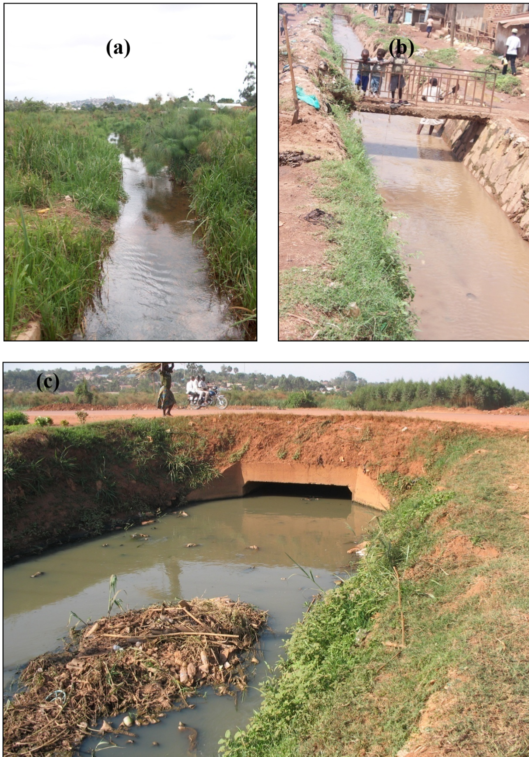
Figure 3.3. Photos of drainage channels (a) An unlined secondary channel in the upstream areas of the catchment, (b) a lined secondary channel in downstream areas of the catchment and (c) a lined primary Nsooba channel immediately before discharging into Lubigi wetland.
