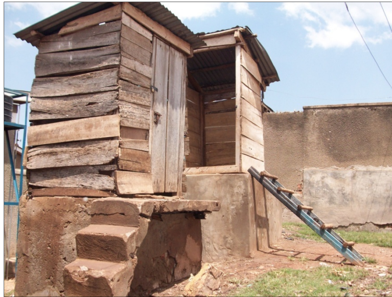
Figure 5.2: A typical elevated pit latrine in Bwaise III parish slum, Kampala Uganda. The pit latrines are usually elevated or raised above the ground due to the high water table in the area. This prevents the pits from filling up with water. Also see Fig. 4.3a
