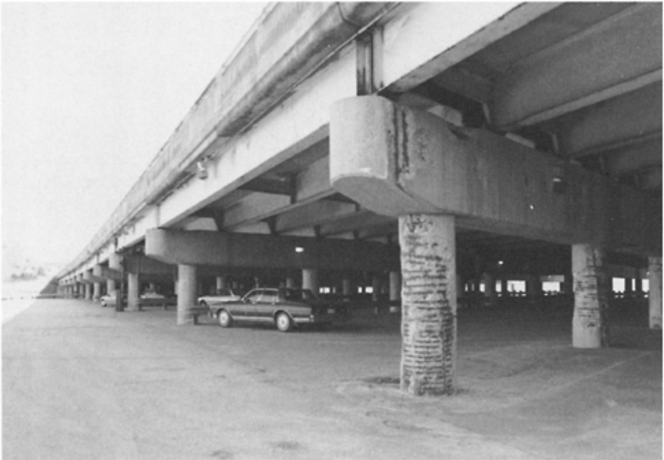
Fig. 1. Damaged bridge along highway 401 in Ontario
