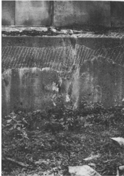
Fig. 7. Delamination in steel fiber reinforced shotcrete at the Stave dam.
