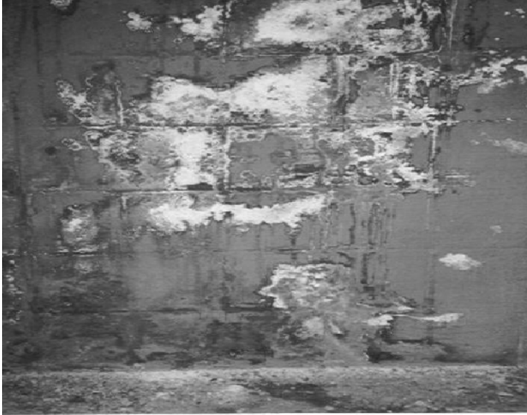
Figure 4.20 Penetration of sulfate-bearing ground water through a retaining wall exposed to atmospheric changes (wetting–drying, heating–cooling) (Photo J. Skalny).
