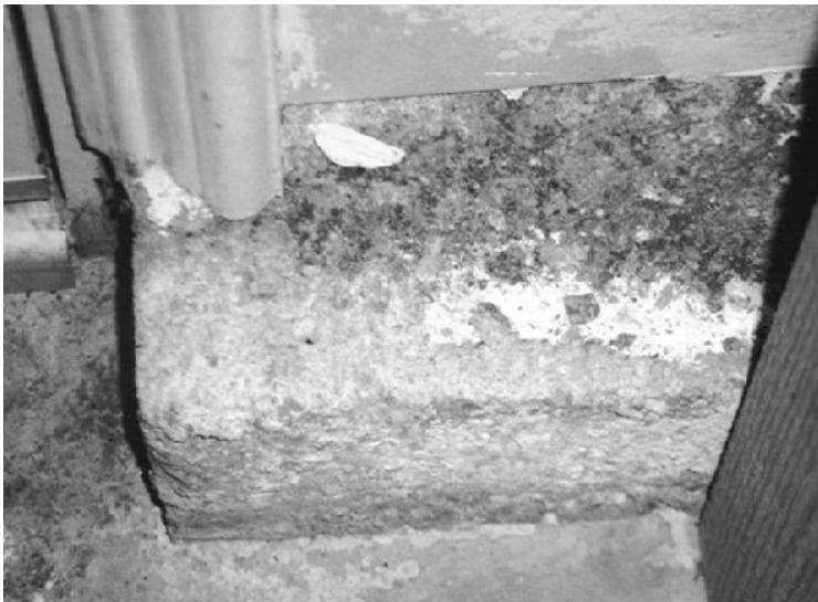
Figure 8.1 California residential house footing exposed to sulfate-containing ground waters. Note spalling and efflorescence (Photo: J. Skalny).
