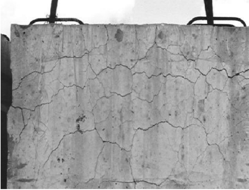
Figure 4.2 Prefabricated concrete beam damaged by combined action of ASR (primary mechanism) and heat-induced ettringite expansion (Photo courtesy of M. Thomas).
