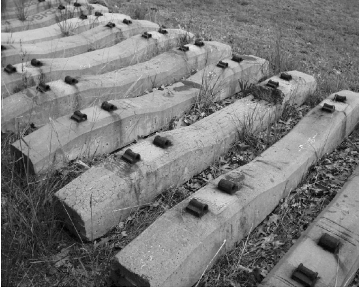
Figure 1.3 Damaged and undamaged railroad ties (Photo courtesy of N. Thaulow).
