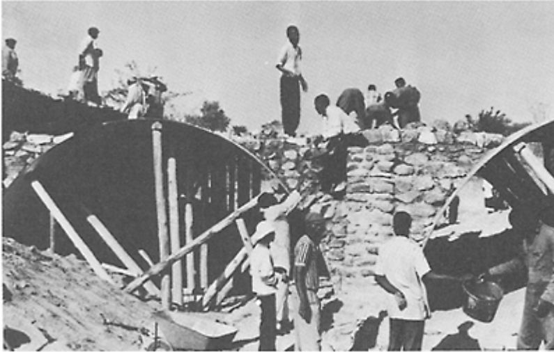
Figure 1 Construction of a typical bridge showing the temporary corrugated iron and gum pole centering used to form a 2, 7m radius arch.
