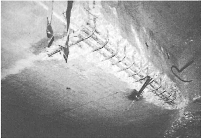
Figure 3—Congestion due to inadequate bar spacing resulting in rock pocket.
