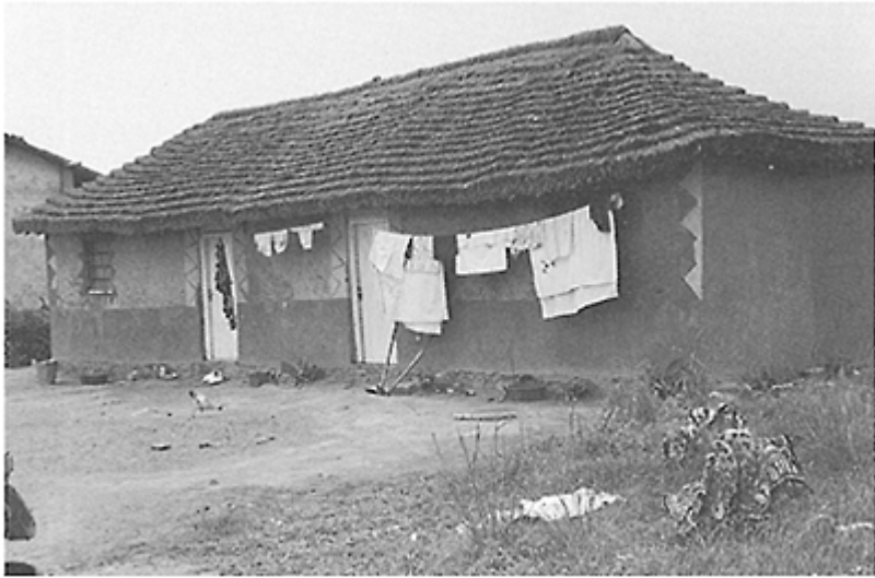
Fig. 1. Building used by MRHP near Missungwi, Tanzania, to evaluate the durability of different types of plaster layers.
