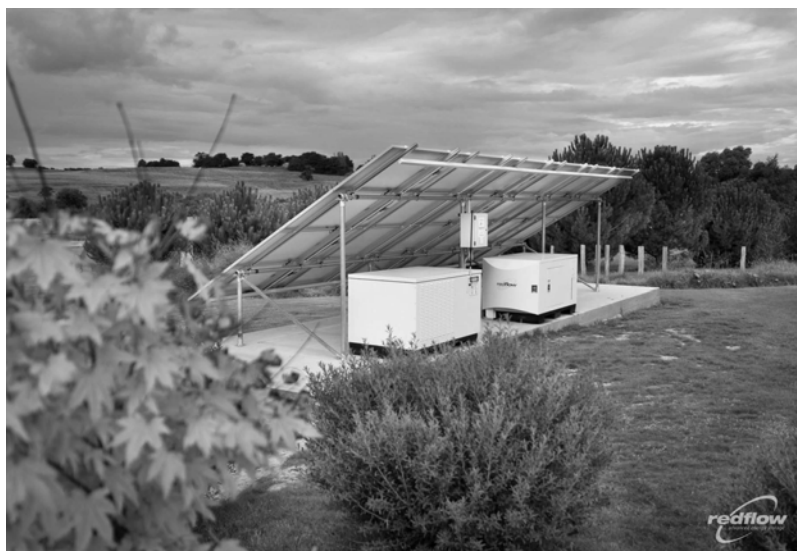
Figure 12.23. Zinc-bromine battery installation in solar power system application. Source: Photo courtesy of Redflow
