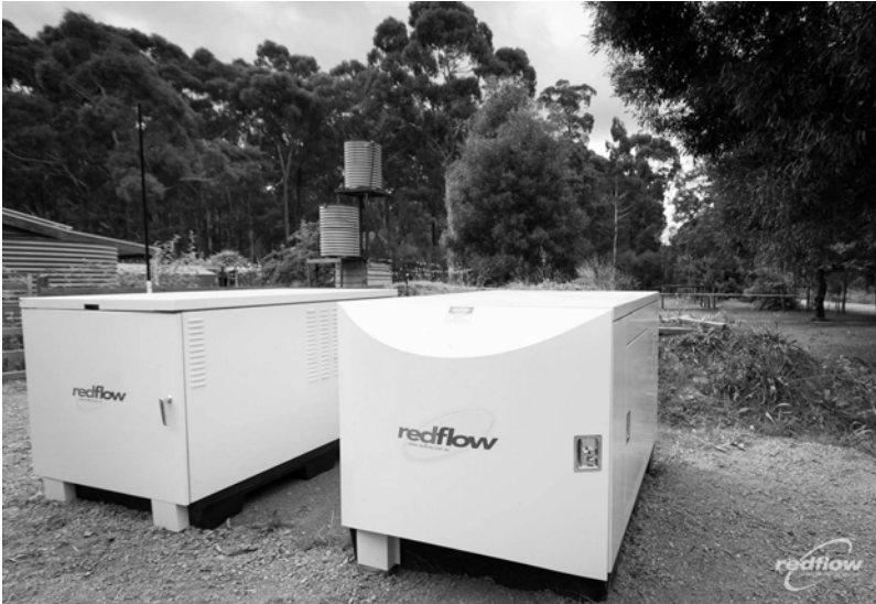
Figure 12.22. Zinc-bromine battery installation.
