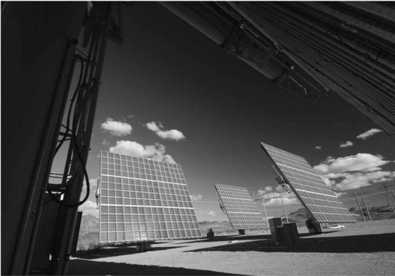
Figure 8.26. A dual axis solar power system.
