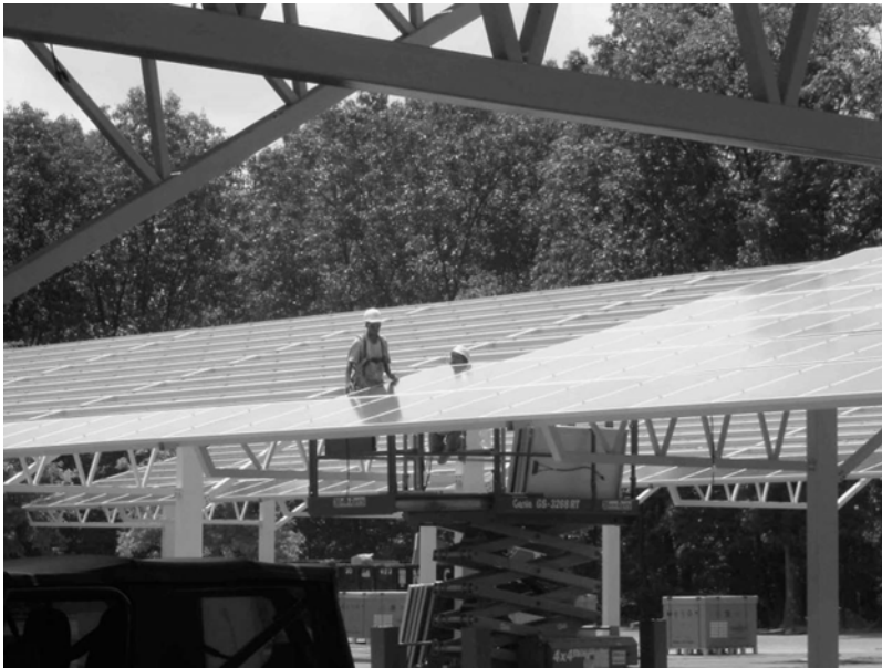
Figure 3.6. Solar power carport system. Source: Vector Delta Design Group, Inc.
