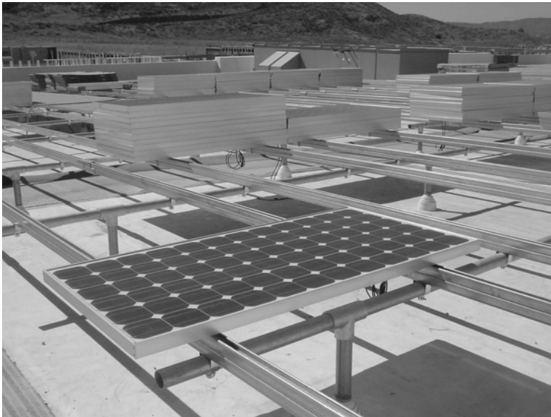
Figure 3.22. Solar PV module system installation.
