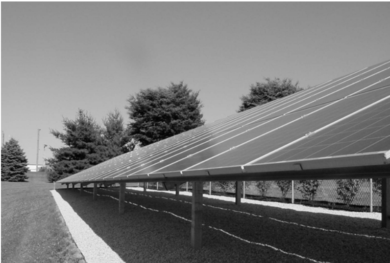
Figure 3.15. A fixed angle solar power system.
