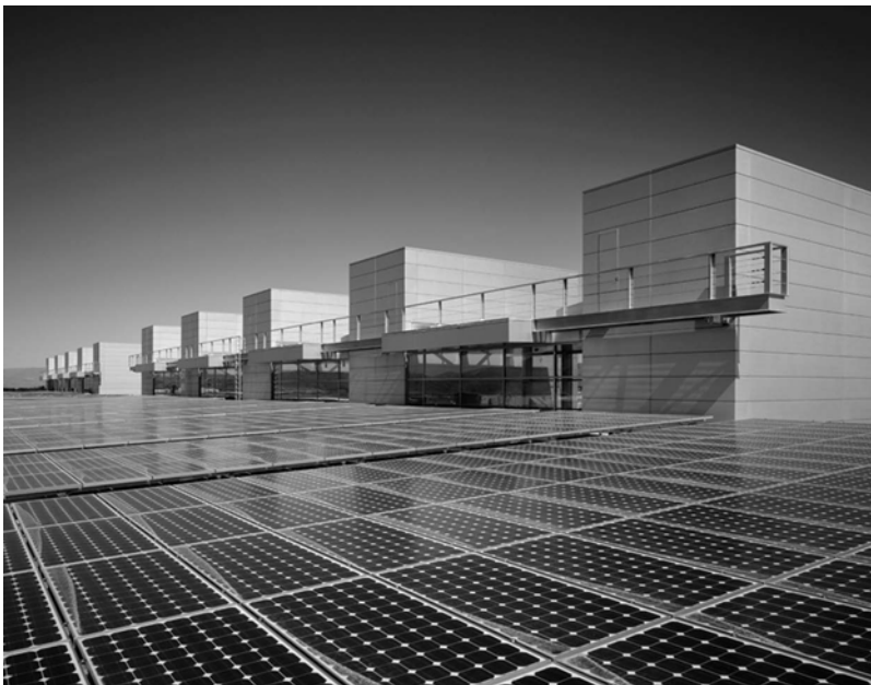
Figure 3.7. A roof mount solar power system. Source: Vector Delta Design Group, Inc.
