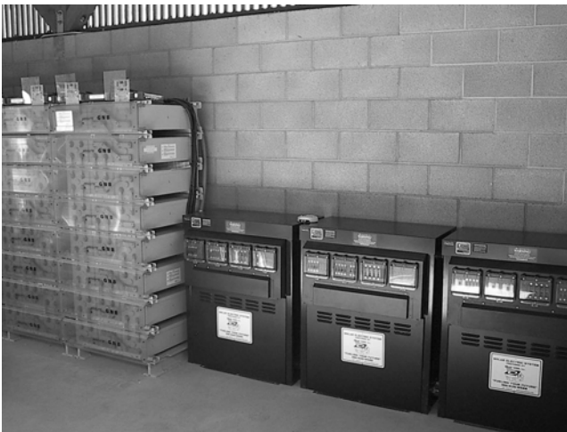
Figure 12.3. Deep-cycle lead acid battery pack.
