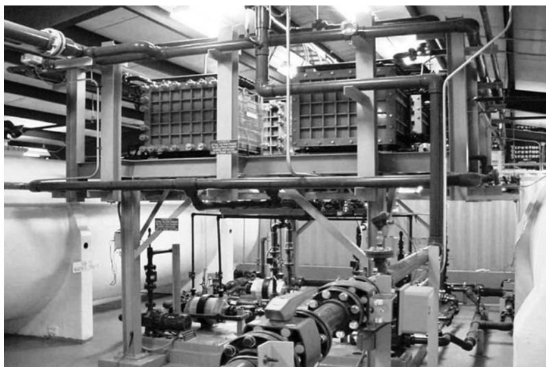
Figure 12.20. A 200-kW vanadium redox flow battery installation. Source: Photo courtesy of VRB-ESS, Utah, United States
