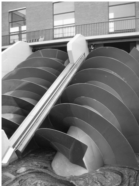
Figure 8.3 Archimedean screw pumps in Kinderdijk, The Netherlands.
