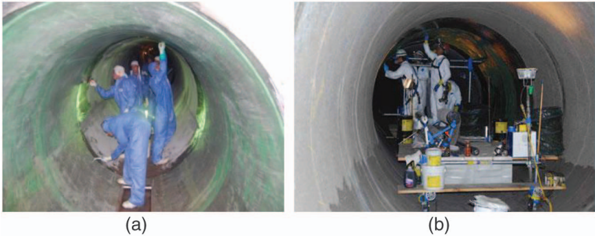
Fig. 5-16. (a) Application of tack coat to upper half of pipe; (b) bottom half of pipe sealed with saturating resin
