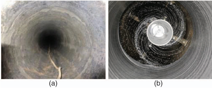
Fig. 5-6. (a) Pipe after the cleaning and (b) lining process with the spray head in the pipe's center
