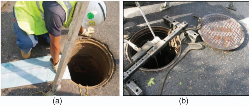
Fig. 5-2. (a) Impregnated tube inserted in entry pit; (b) use of winch to pull impregnated tube Source: Insituform Technologies, LLC; reproduced with permission
