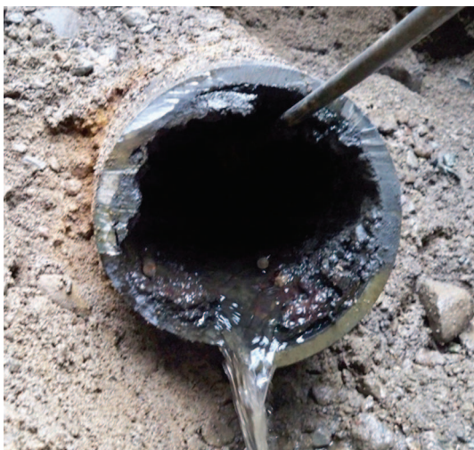
Fig. 1-1. Effects of tuberculation, age, and corrosion on water pipes Source: 3M Water Infrastructure; reproduced with permission
