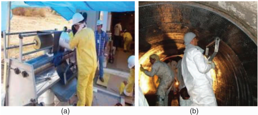
Fig. 5-17. Wet layup method: (a) saturation of the carbon fiber sheet and (b) application of the carbon fiber sheet
