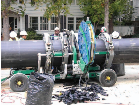
Fig. 5-9. Fusion of 30-in. DIPS HDPE pipe Source: Plastics Pipe Institute; reproduced with permission
