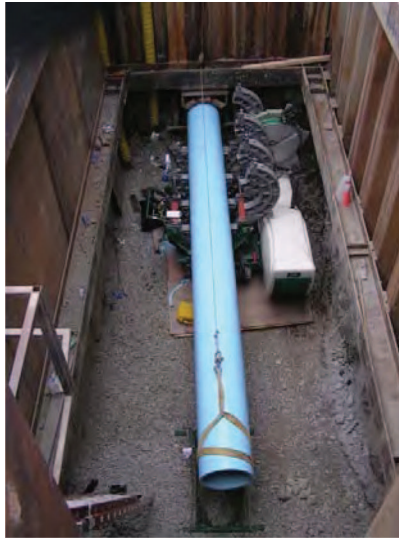
Fig. 5-10. In-pit fusion of 24-in. PVC Source: Underground Solutions, Inc.; reproduced with permission
