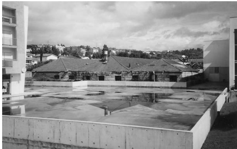
Fig. A2.4 Roof detailing. The flat roof needs expensive and disruptive repair every ten years or so and is a well-known source of problems in wet climates. By comparison the pitched roof needs less maintenance with an average of 50 years between repairs. The pitched roof is a better example of detailing with nature than the flat roof.
