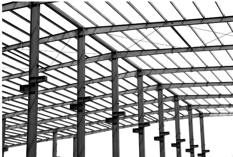
FIGURE 7–1 (See color insert.) Elements loaded in bending require more analysis than those with simple axial loads, and proper calculation and design is critical. Look at all the beams in this building, and consider the serious responsibility of the designer to assure that, once completed, these beams can safely support the roof panels, the roofing material, and all other loading.
