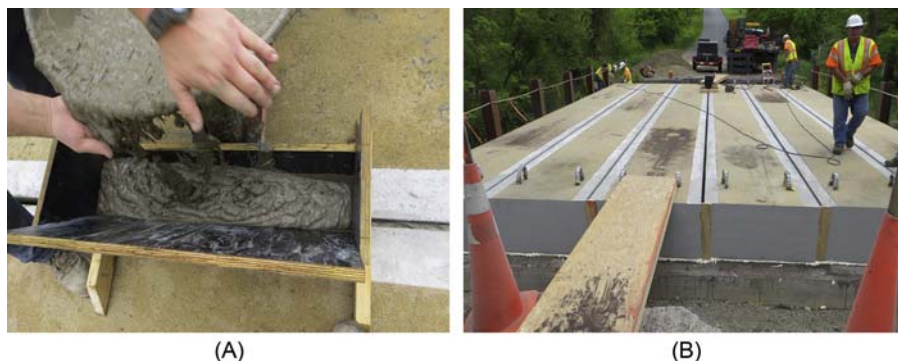
Figure 15.24 (A) Engineered Cementitious Composites (ECC) placement through the joint (B) completed shear keys with ECC.
