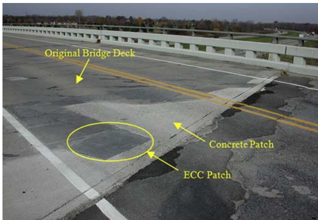
Figure 15.22 Engineered Cementitious Composites (ECC) patch repair placed alongside concrete patch on Michigan bridge deck (Şahmaran and Li, 2016).
