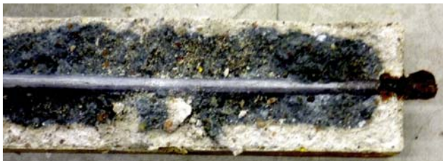
Figure 2.9 Specimen C4, made with seawater after 10 years continuous exposure, after breaking open, showing dark interior, typical of concrete made with sulfate resistant cement and the light outer zone found to be devoid of alkalis such as calcium hydroxide.
