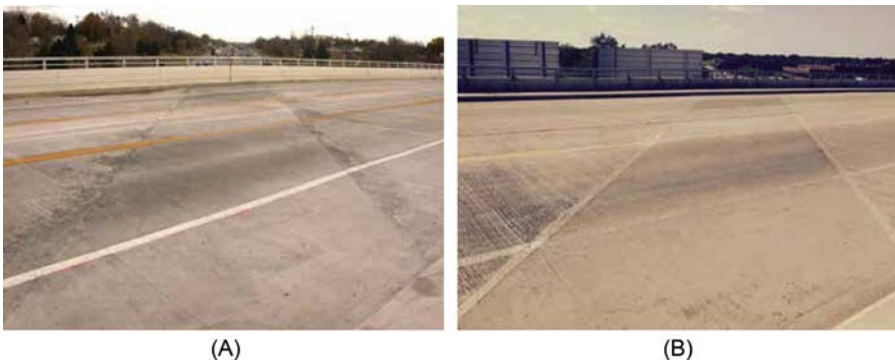
Figure 15.23 After 10 years of service, Engineered Cementitious Composites (ECC) link slab on Grove Street Bridge, MI (A) immediately after construction in 2005, and (B) in 2015 (Şahmaran and Li, 2016).
