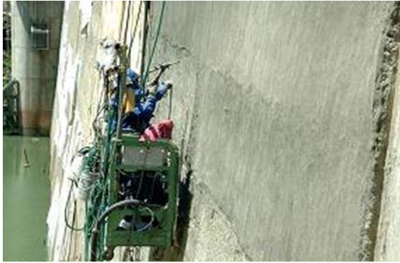
Figure 15.21 Spray repair of the Mitaka Dam with Engineered Cementitious Composites (ECC) for waterproofing (Kojima et al., 2004).
