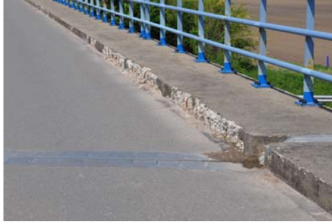
Figure 9.6 Concrete deterioration of the sidewalk.
