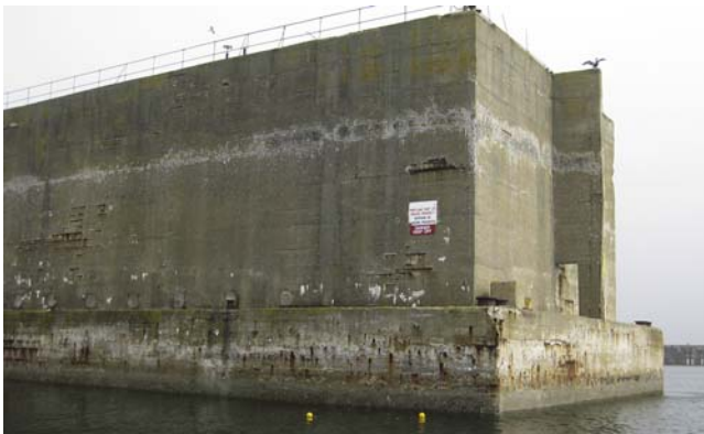
Figure 2.5 End view in 2009 of one of the two Phoenix caissons used as breakwaters in Portland Harbour, UK, showing typical condition of the concrete. Both caissons were constructed in 1943 and intended for use with the Mulberry harbours, but not used.
