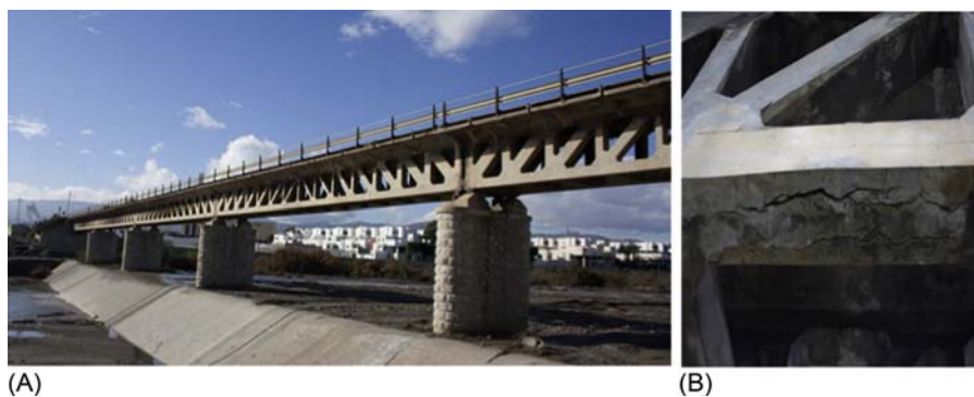
Figure 10.3 (A) Elevation of the Molinos Bridge and (B) Detail of the cracking of its lower chord.
