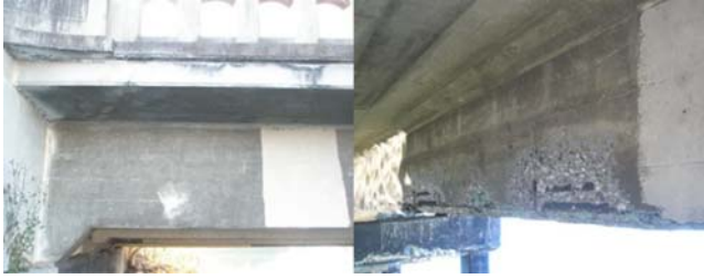
Figure 4.1 Two photos of the same reinforced concrete girder showing no concrete damage on the ocean-facing side (left) and corrosion damage on the face of the beam opposite the ocean (right).
