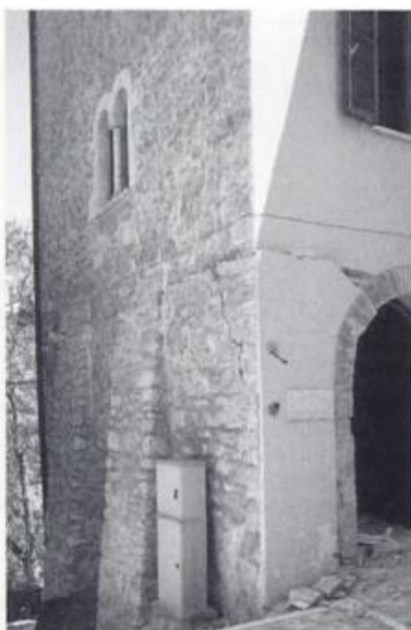
Figure 17. Damage due to new r.c. slab, which pushed out parts of masonry wall.
