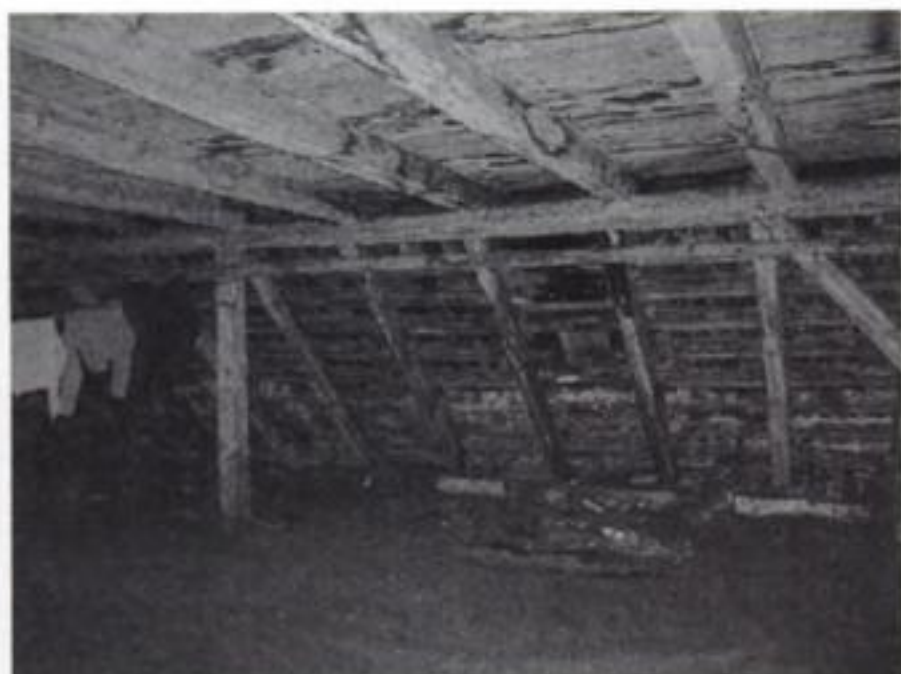
Figure 6. Deterioration of a wooden roof structure.
