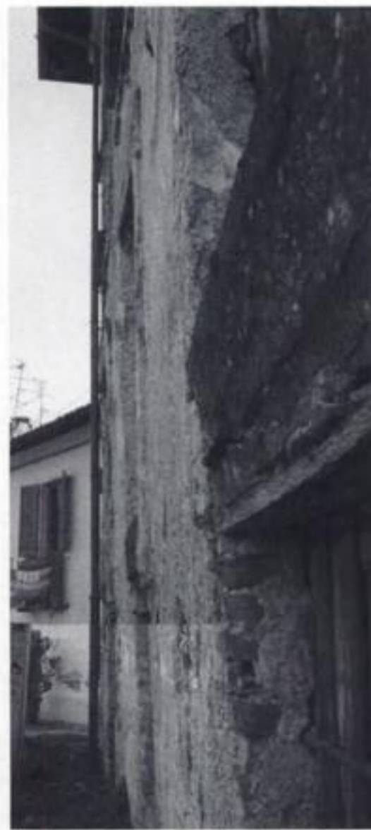
Figure 9. Vista of the left portion of the North elevation with spalling of wall.
