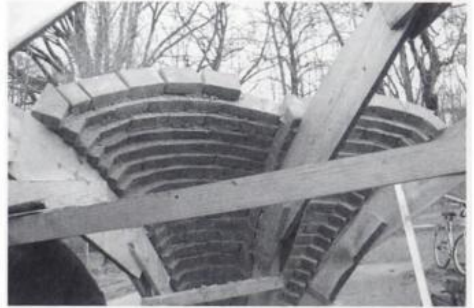
Figure 17. The cap masonry during construction; the shifting of the courses outwards is visible (prototype).
