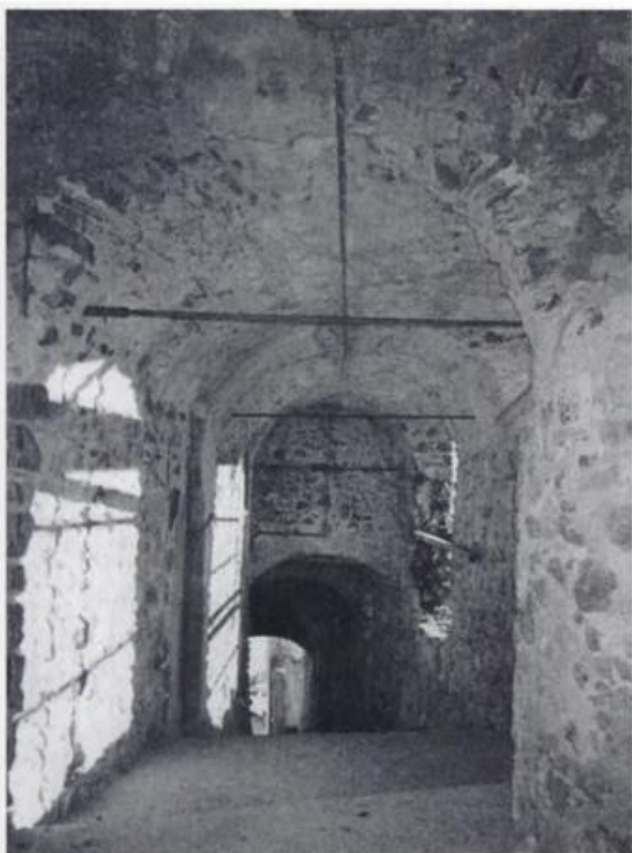
Figure 1. The habitable buttressing arch built with stones and bricks in the old town of Sillano.
