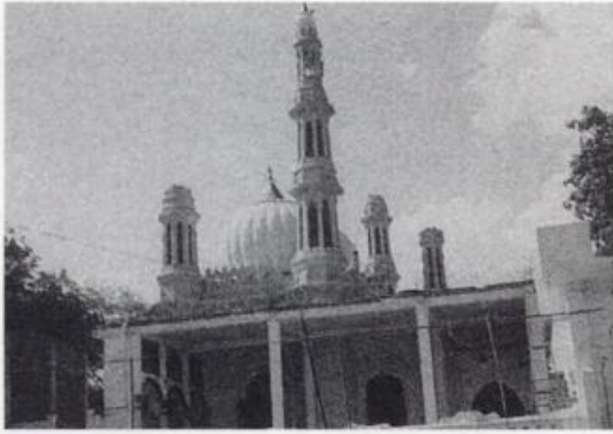
Figure 8. Mosque with collapsed minarets during Jabalpur earthquake.
