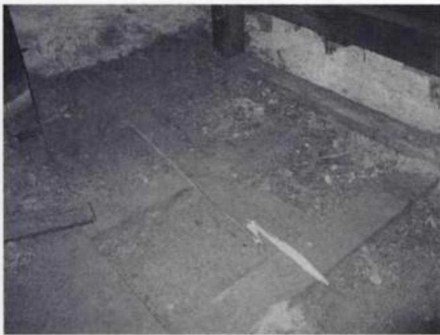
Figure 4. The deterioration of a wooden floor under a roof.
