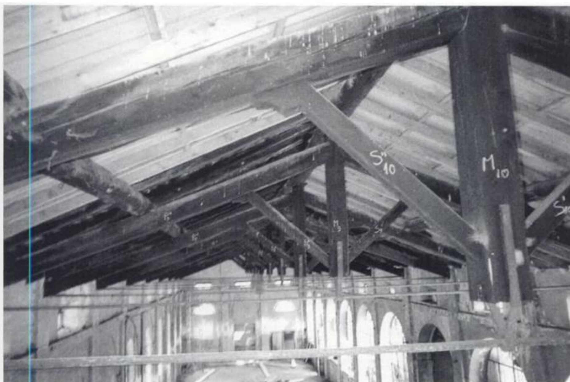
Figure 4. View of the South building's trusses from the East end of roof.
