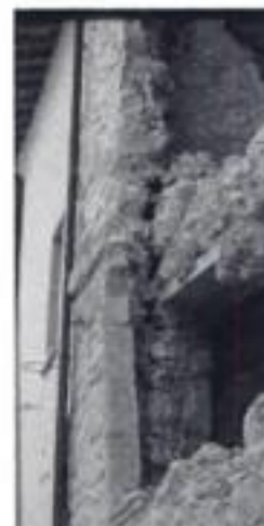
Figure 1. Collapse of a repaired walls.
