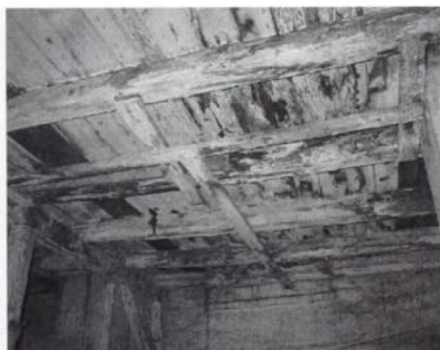
Figure 7. Details of wooden roof biological corrosion.
