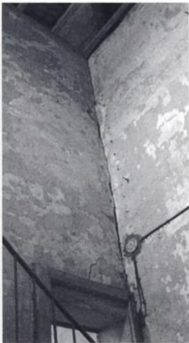
Figure 8. Crack running vertically at the corner between bracing wall and longitudinal wall in the staircase.
