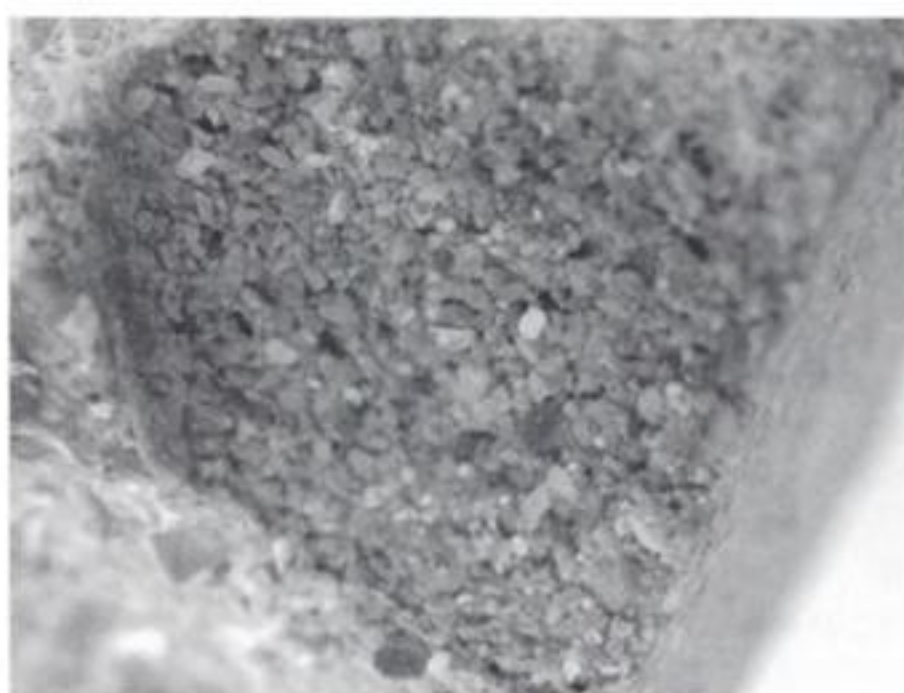
Figure 14. Mortar enlargement showing the absence of cementitious component.
