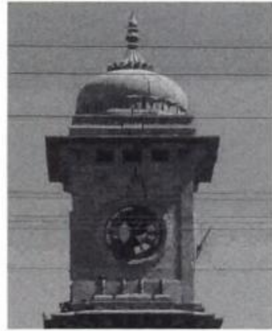
Figure 10. Earthquake damaged clock tower at Morbi, Gujarat.
