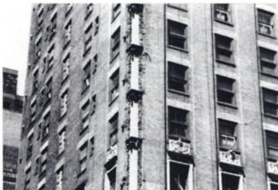
Figure 6. Corner column masonry removed and column cleaned and painted at Four Park Avenue.
