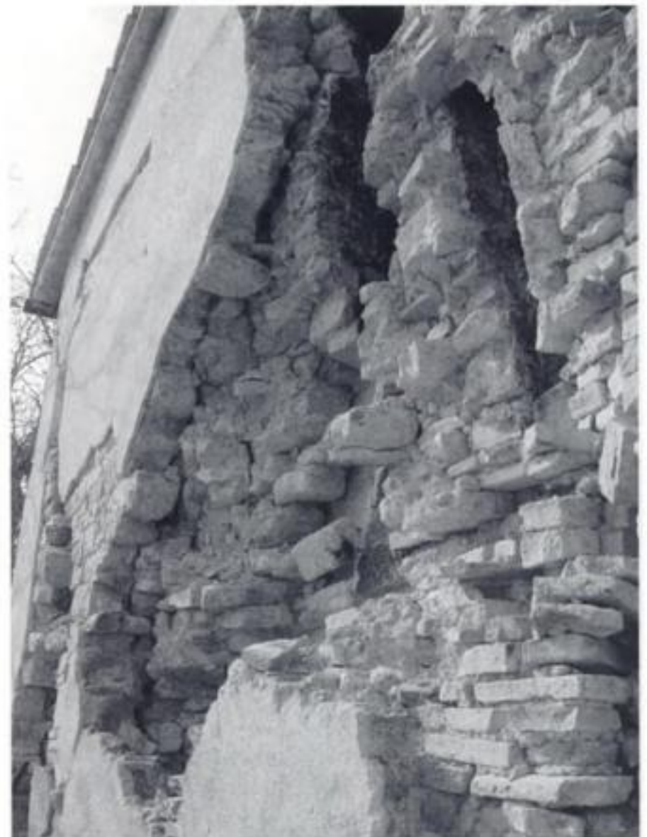
Figure 1. Failure of a multi-leaf stone wall, from Nocera Umbra (Italy).
