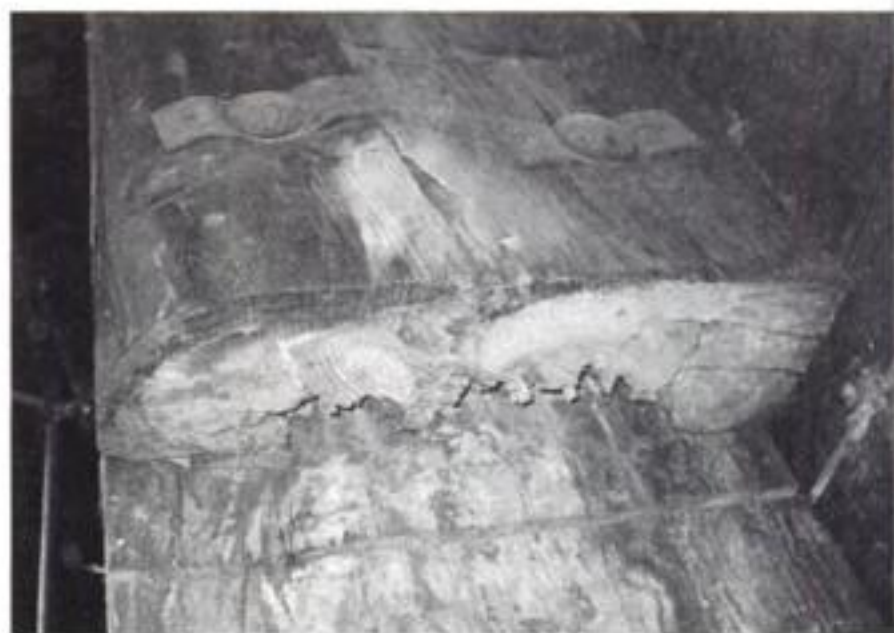
Figure 3. Detail of the deterioration of the ribs detected in the joints.
