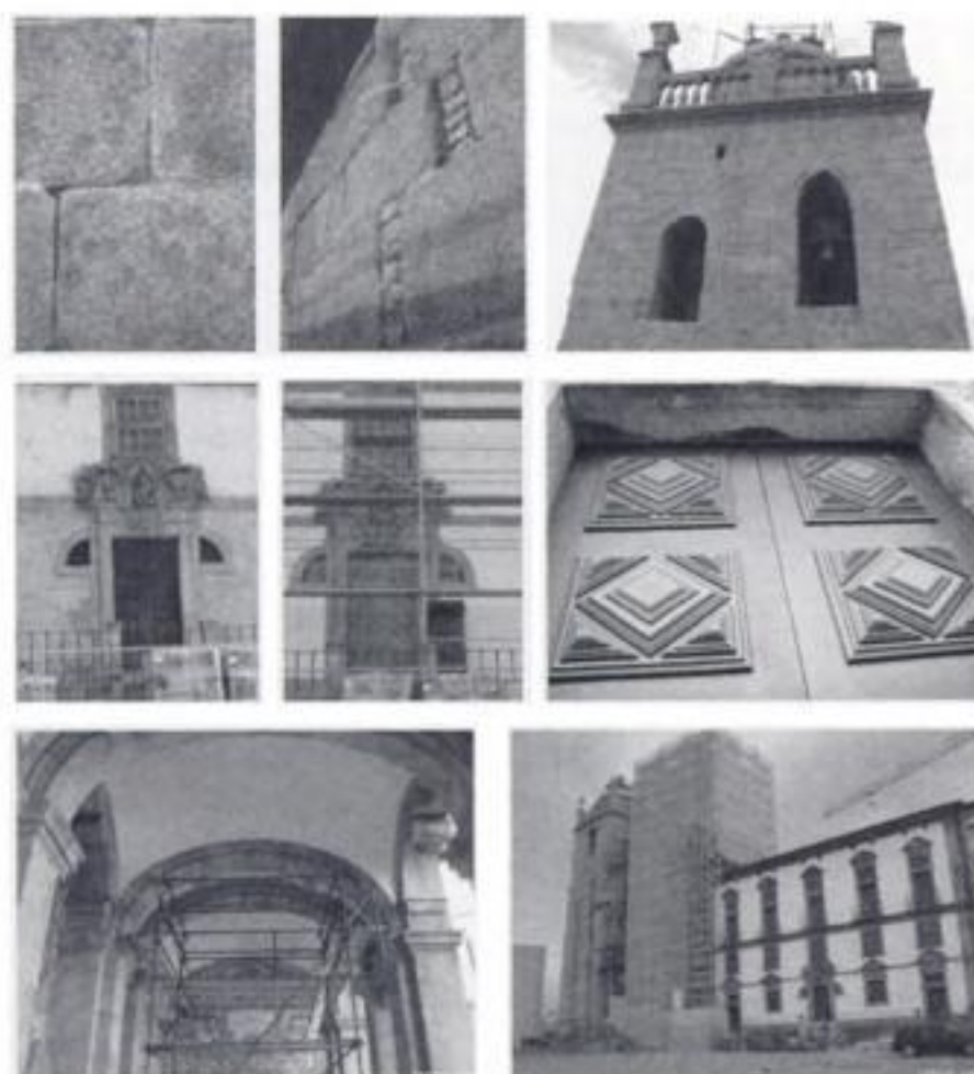
Figure 9. Repair of finishings included repointing of masonry joints with lime mortar and repainting of wood with traditional oil paints.
