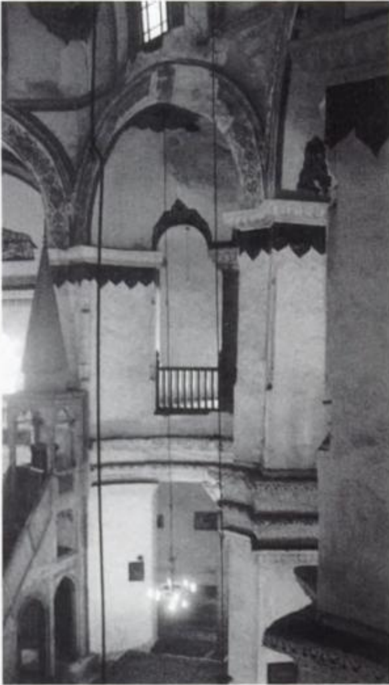
Figure 1. Deformation of piers.
