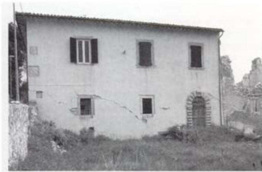
Figure 7. Typical shear cracks in the walls of a historic stone-masonry house.
