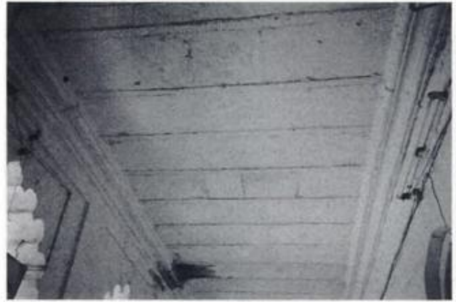
Figure 16. Jack arch floor of the circuit house which underwent severe cracking.
