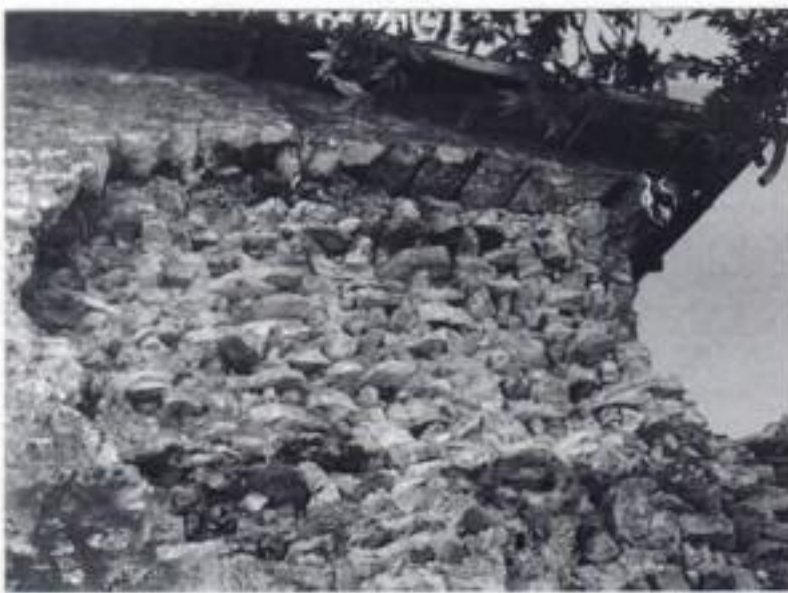
Figure 8. Damages after Umbria earthquake: collapse of the outer leaf of the wall.
