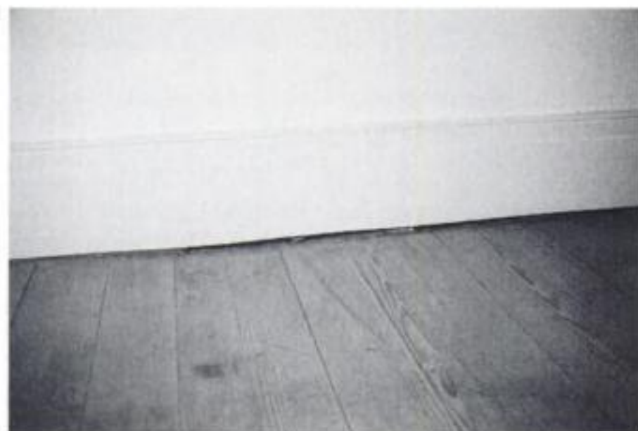
Figure 12. Gap between wall and floor exposes brick nogging.
