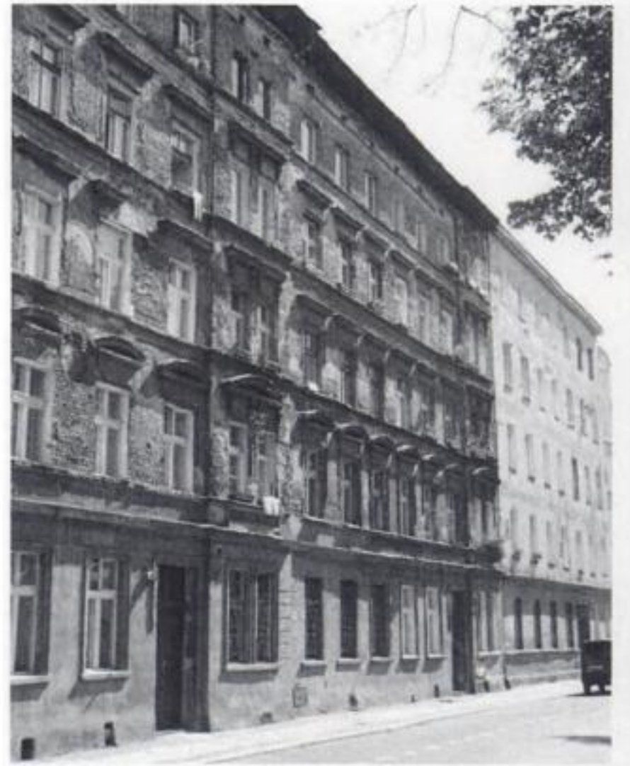
Figure 1. An example of a deteriorated front façade.
