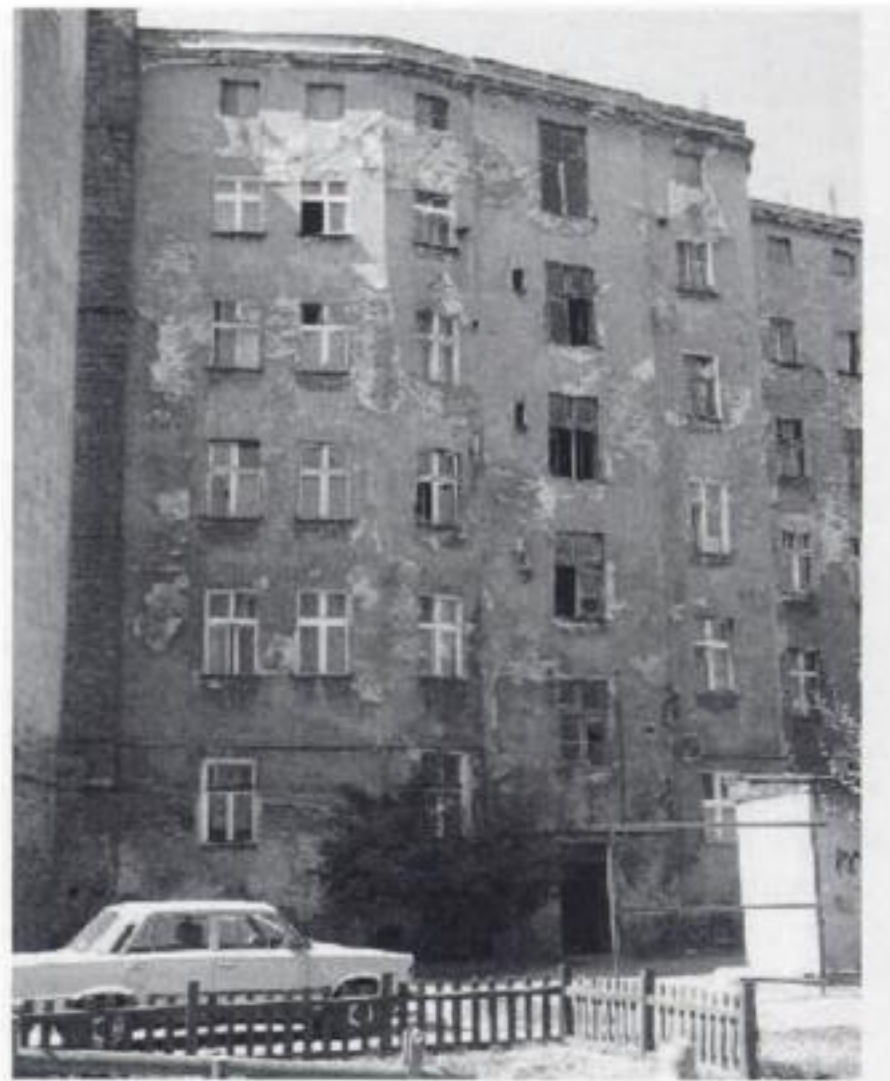
Figure 2. An example of a deteriorated back façade.
