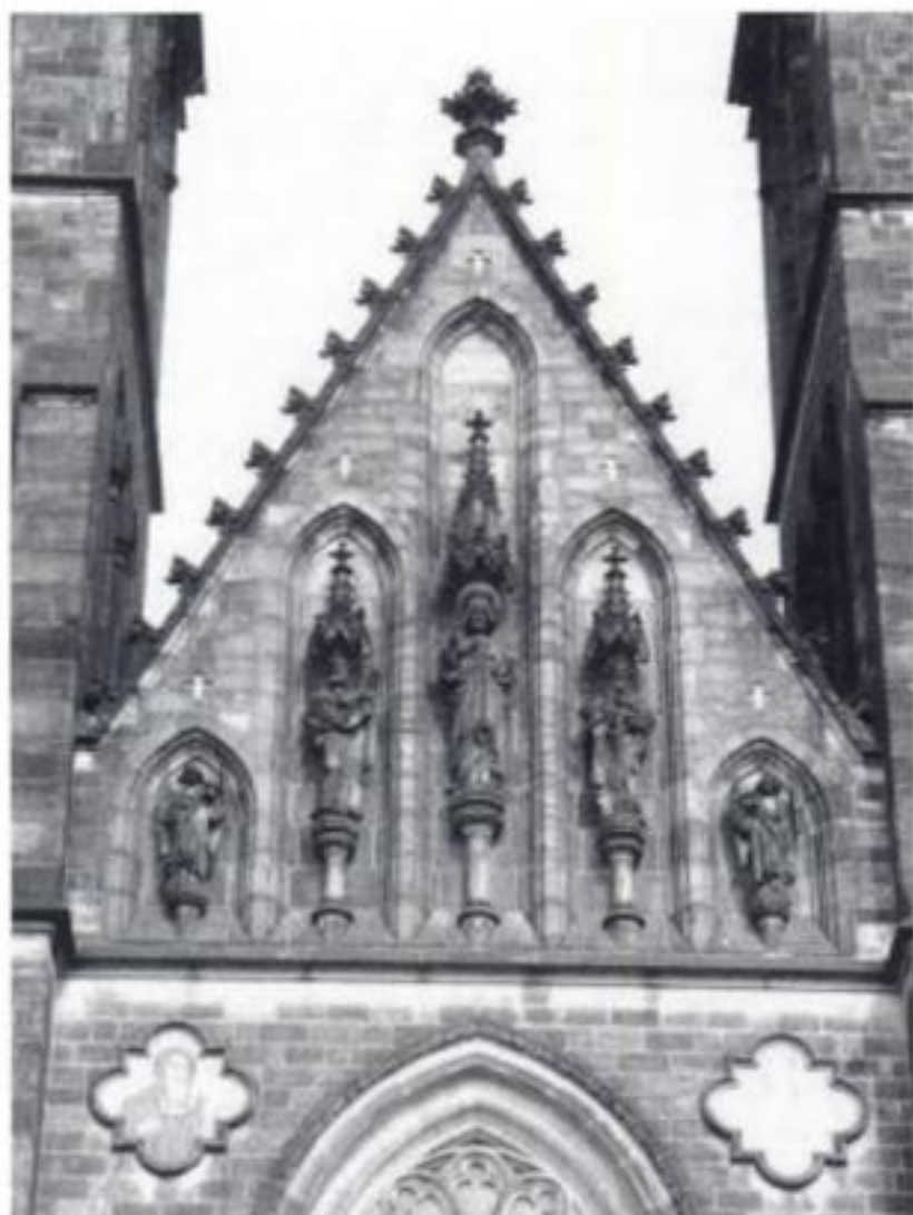
Figure 8. The wobbling gable.
