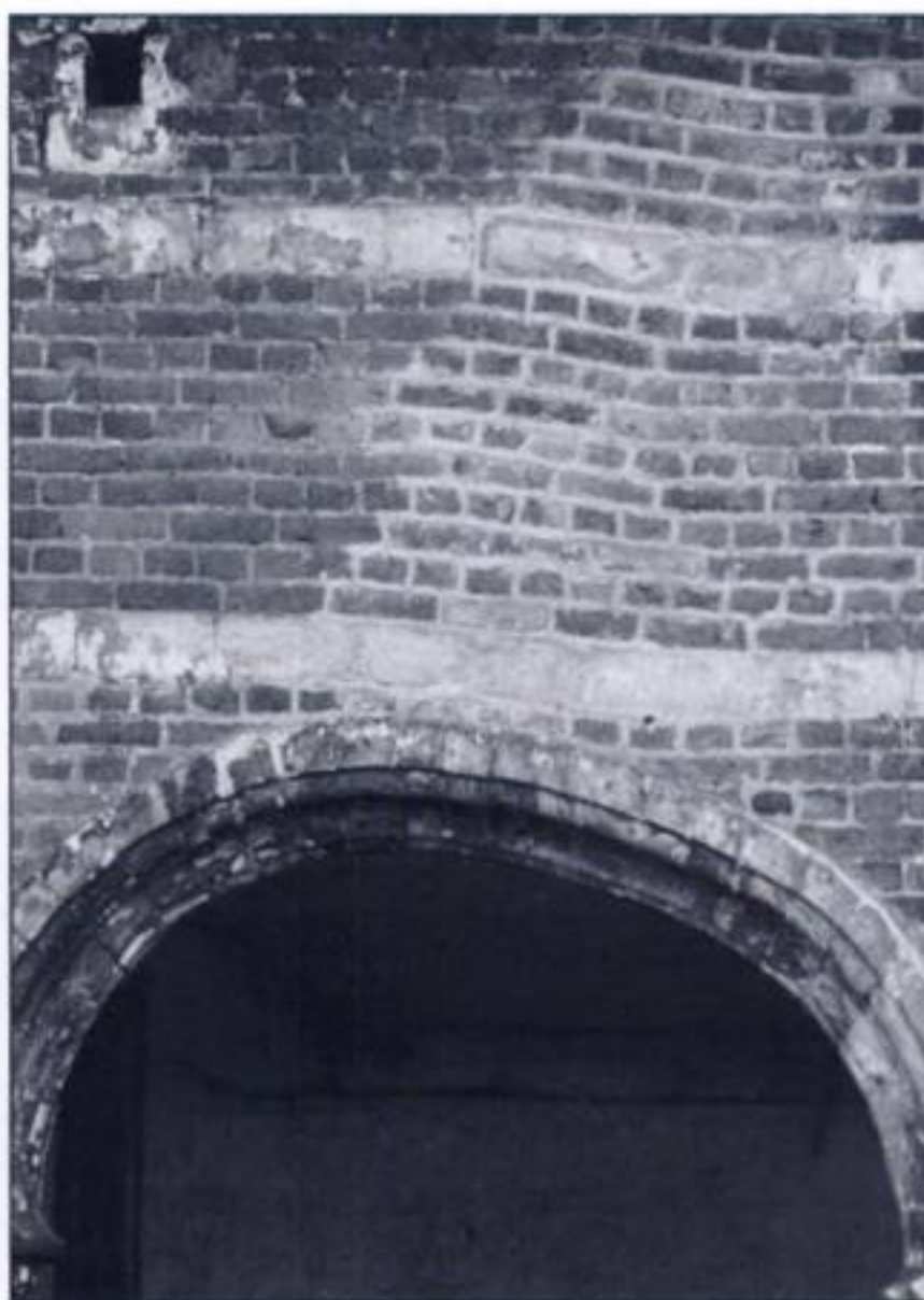
Figure 1. Settlement of a historical masonry structure without actual structural failure of the structure.
