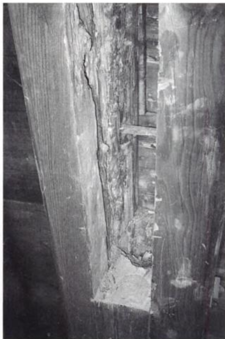
Figure 4. Deterioration of the internal part of the ribs.
