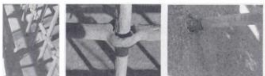
Figure 7. Repair of grilles included control of anchors and new anchors, and measures for proper rainwater flow.
