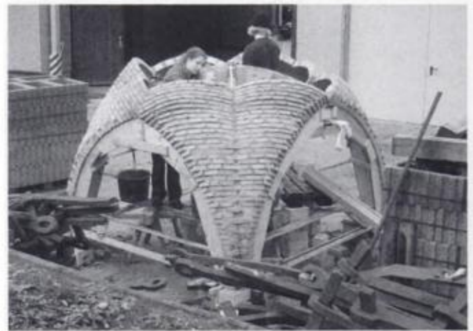
Figure 10. Experimental construction of a cross vault without formwork, using the dovetail pattern. The design reproduces in scale 1:4 a late gothic church vault in northern Germany. Dimensions in plan: 2.50 × 2.30 m. Dresden University of Technology, 2003.
