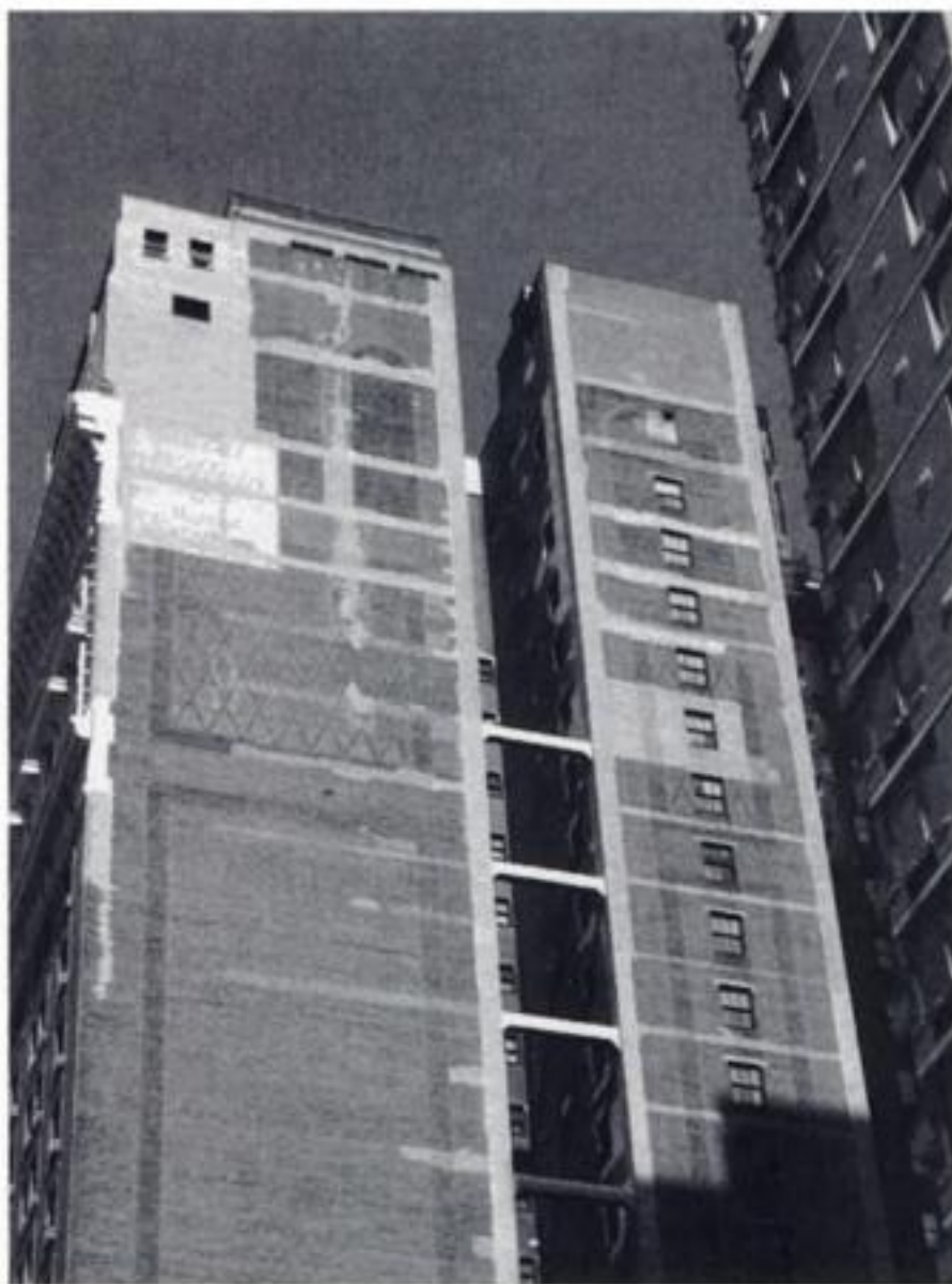
Figure 5. Old beam and corner column masonry repairs at the rear façade 50 West 34th Street.
