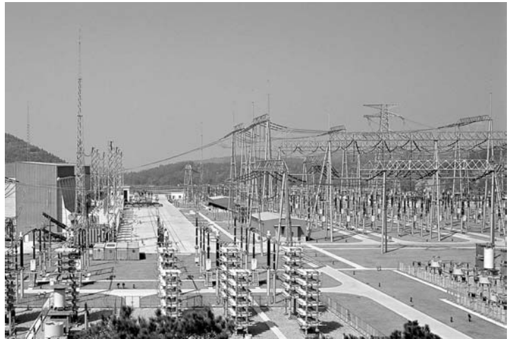
Zhaoqing power converter station for high-voltage direct-current transmission line, Guangdong province, China Siemens press picture, © Siemens AG
