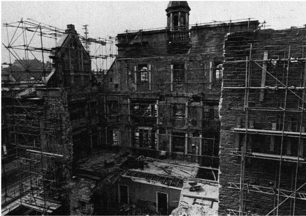
Figure 7.78 3-13, George Street, Edinburgh: retained facade near completion of demolition works showing elements of temporary support system.
