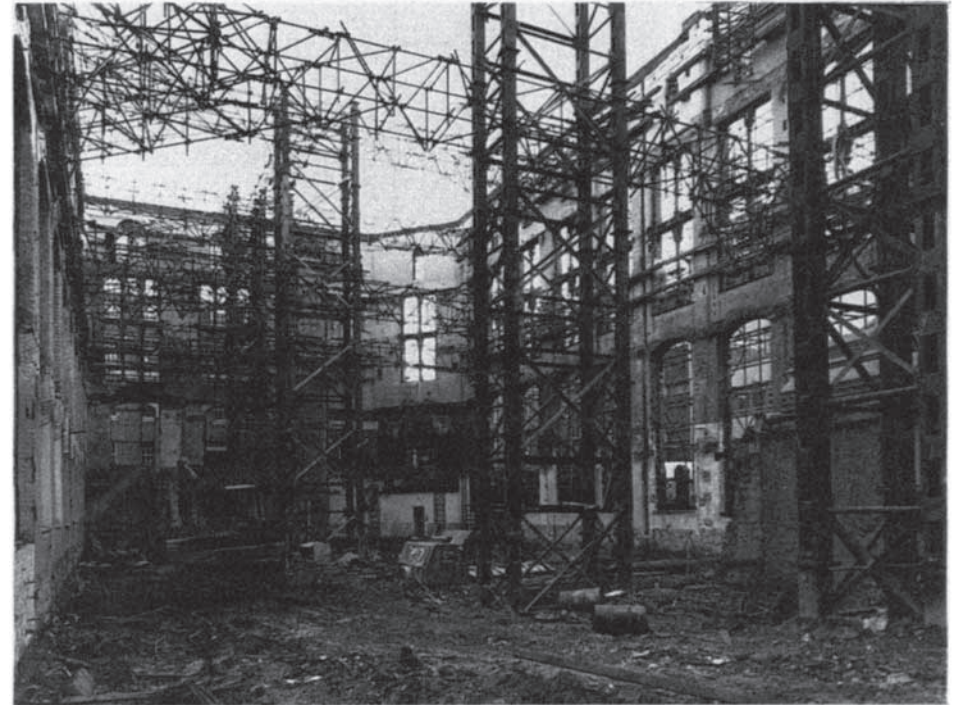
Figure 7.23 St Paul's House, Leeds: interior view showing temporary support towers and flying shores.
