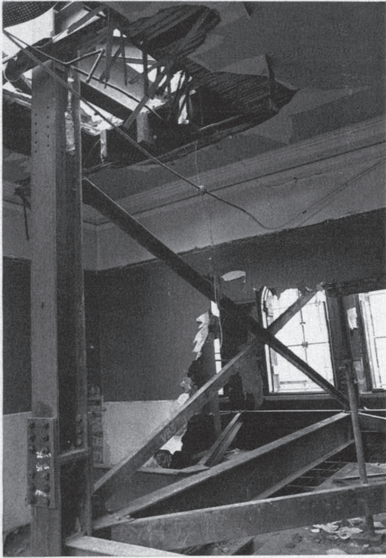
Figure 7.11 118–120 Colmore Row, Birmingham: elements of temporary support system threaded into the existing structure.
