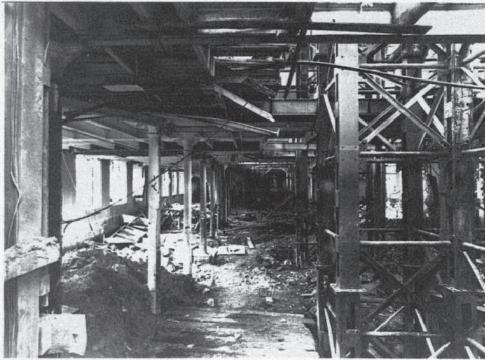
Figure 7.22 St Paul's House, Leeds: elements of temporary support system erected within the existing structure.
