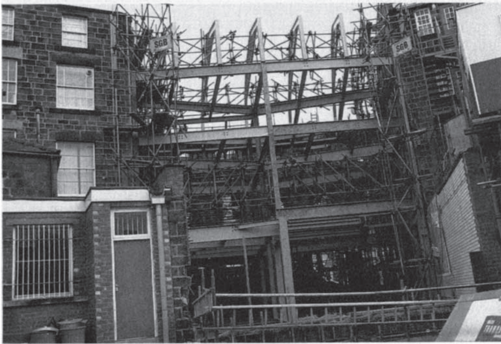
Figure 7.38 Lloyds Bank, Harrogate: view from rear showing temporary support system and new steel frame.
