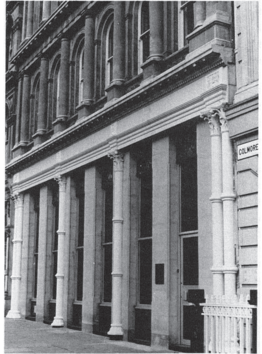
Figure 7.97 Barclays Bank, Birmingham: after redevelopment showing the original cast iron columns retained as part of the new ground floor frontage.
