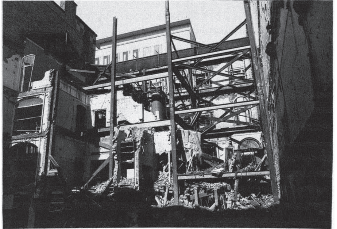
Figure 7.12 118–120 Colmore Row, Birmingham: view from rear showing elements of temporary support system during demolition work.
