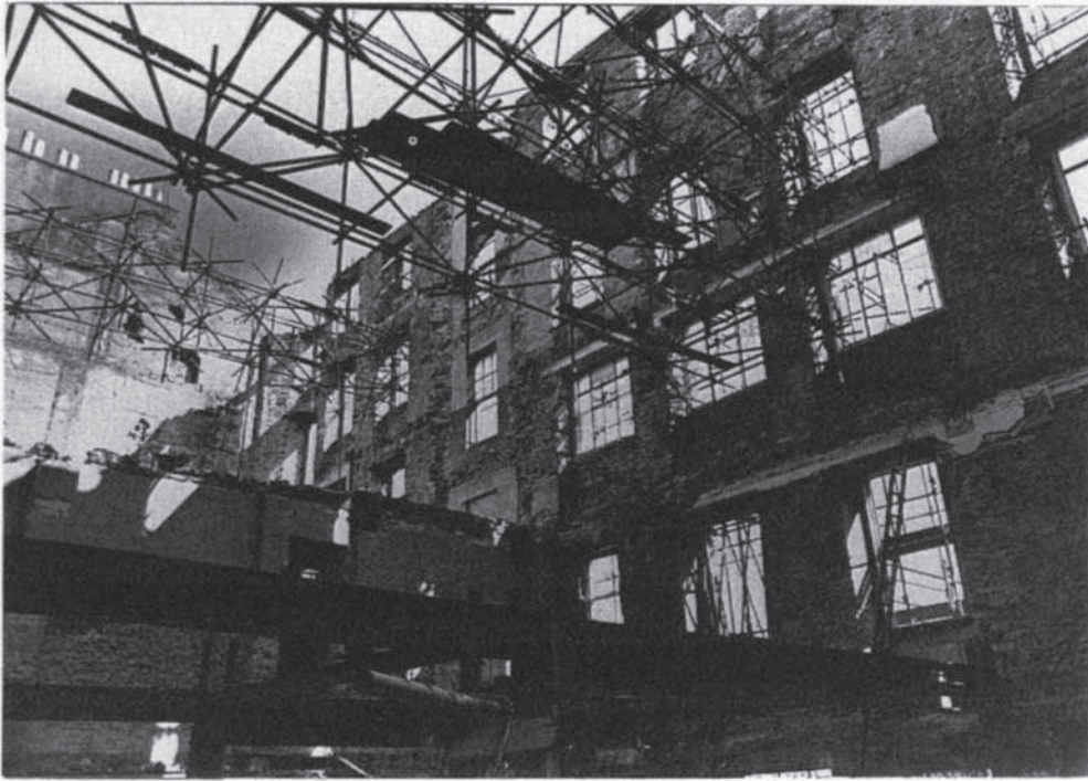
Figure 7.67 1-3, Baxter's Place, Edinburgh: interior view after completion of demolition works showing temporary flying shores.
