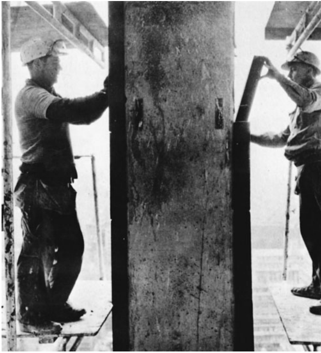
Figure 15-3 Insulating a Column against Temperature Changes. (Reprinted by permission of Pittsburgh Corning Corp.)
