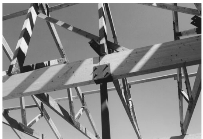
Figure 8-15 (a to f) Typical Noncontinuous Beam-to-Column Connections. (g) Single-Span Glulam Beams Supported by Steel Saddle and Column.
