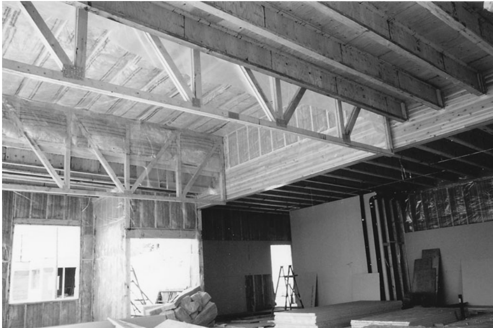
Figure 12-28 Glued-Laminated Roof Girder Supporting Roof Trusses and I-Shaped Wood Joists at 24 in. (600 mm) on Center.
