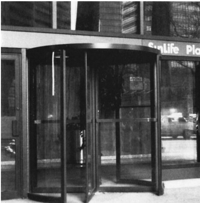
Figure 16-17 Revolving Doors are Efficient in Controlling Air Loss from an Air-Conditioned Building.
