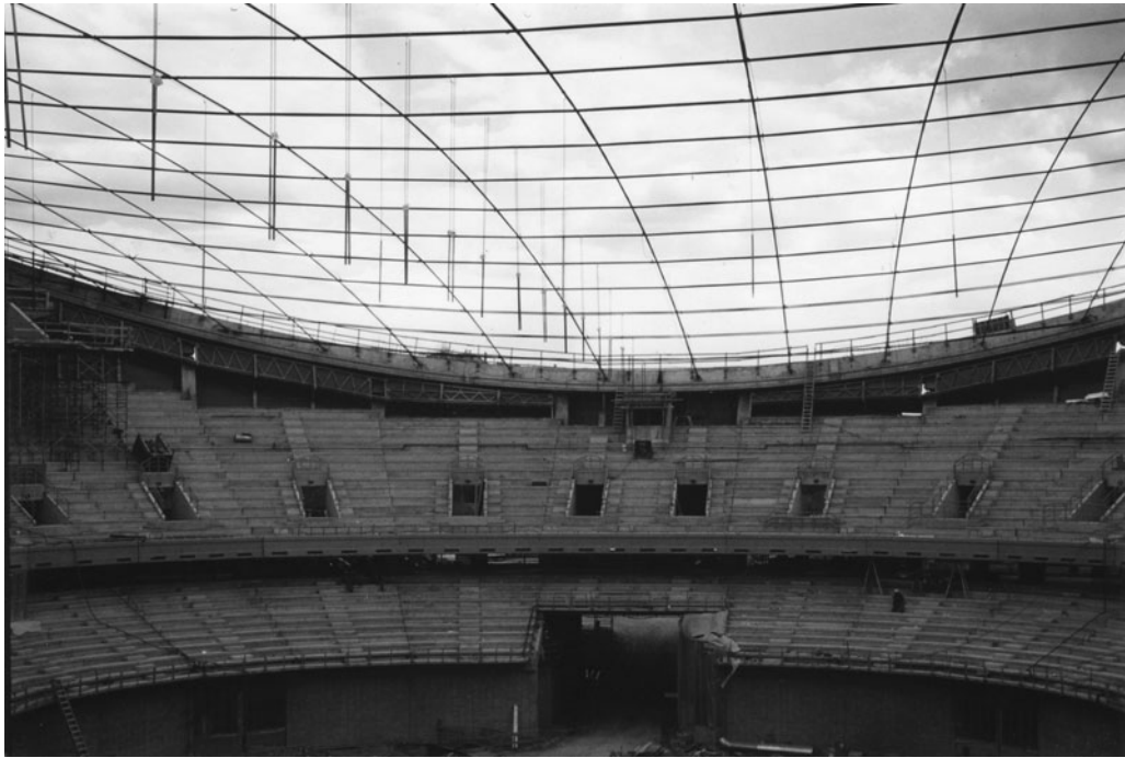
Figure 12-52 Support Cables in Place for Cable-Supported Roof.
