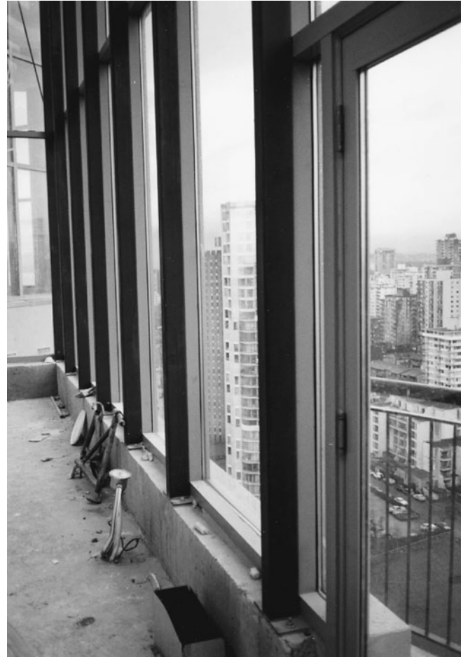
Figure 14-45 Hollow Structural Steel Sections Used as Lateral Support Framing for Glass Curtain Wall.
