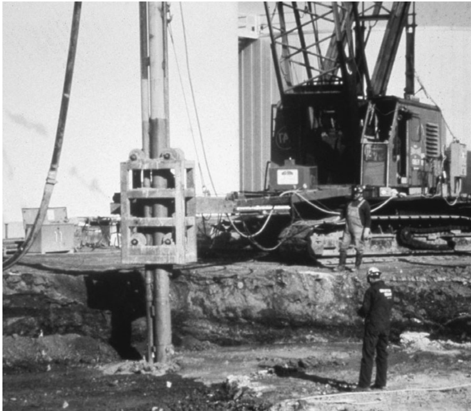
Figure 5-40 Soil Stabilization as a Result of the Vibration Process. (Courtesy Hayward Baker Inc.)
