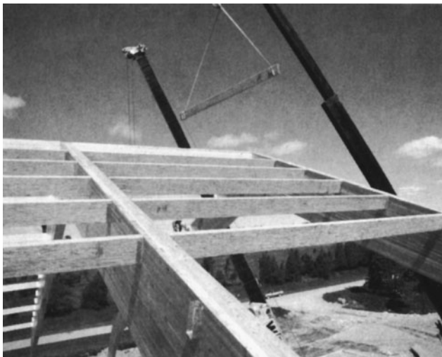
Figure 8-19 Intermediate Beams Framed with Hangers. (Reprinted by permission of Canadian Wood Council.)
