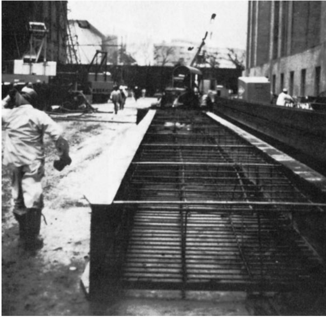
Figure 3-56 End Beams and Reinforcing Cage Welded Together. (Reprinted by permission of I.C.O.S. Corp. of America.)
