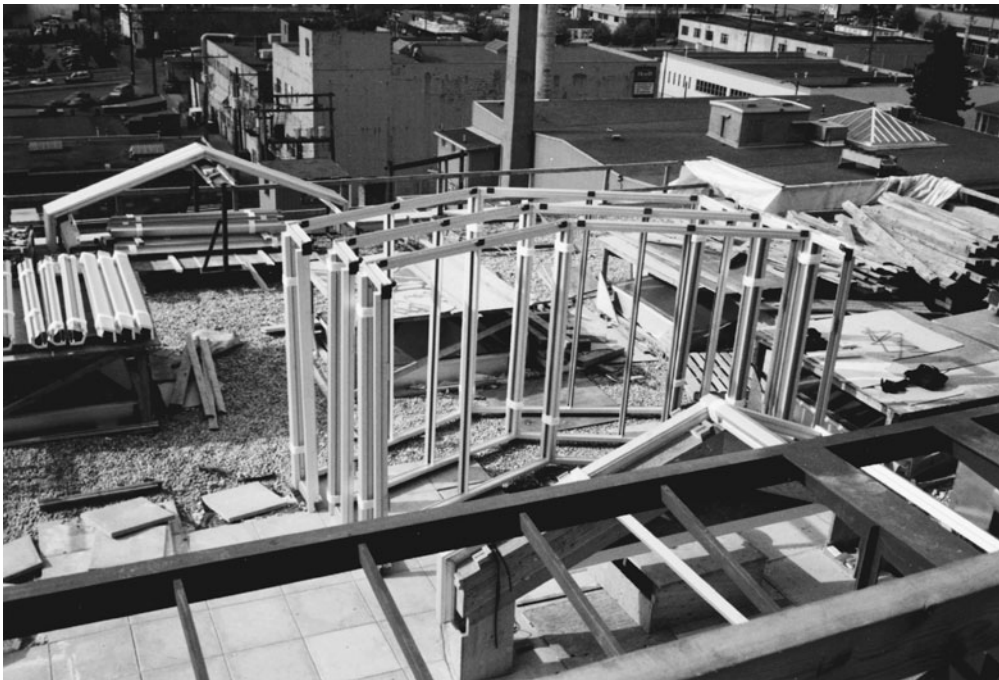
Figure 14-43 Precut Extruded Aluminum Sections for Glass Curtain Wall Framing Assembled on Site.
