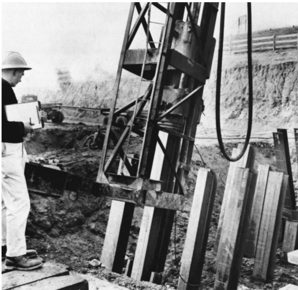
Figure 5-19 Air Hammer Driving Steel HP-Shape Piles. (Reprinted by permission of Bethlehem Steel Co.)
