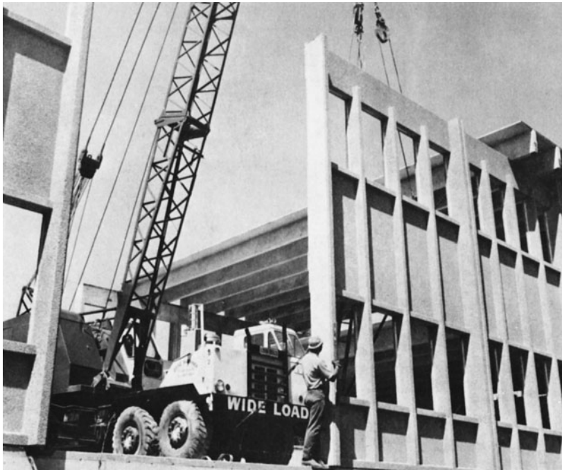
Figure 9-50(a) Erecting Load-Bearing Wall Panel. (Reprinted by permission of Precast/Prestressed Concrete Institute.)
