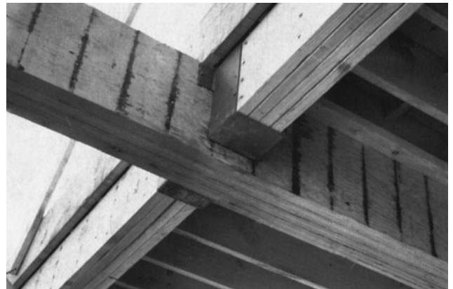
Figure 8-50 Laminated-Veneer Built-Up Girder Supporting Dimensioned Lumber Beam. (Reprinted by permission of Canadian Wood Council.)
