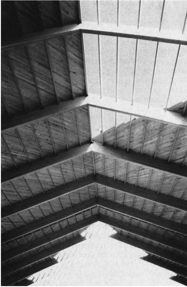
Figure 8-1 Diagonal Decking Adds Rigidity to Structural Frame. (Reprinted by permission of Canadian Wood Council.)
