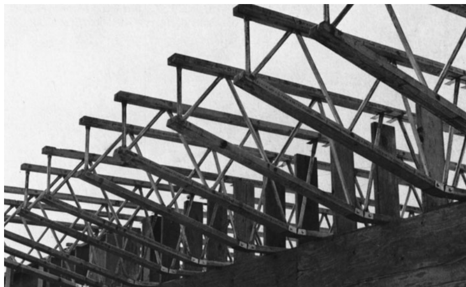
Figure 12-22 Sloping Soffit Formed with Overhanging Open-Web Joists. (Courtesy of Trus Joist, a Weyerhaeuser business.)
