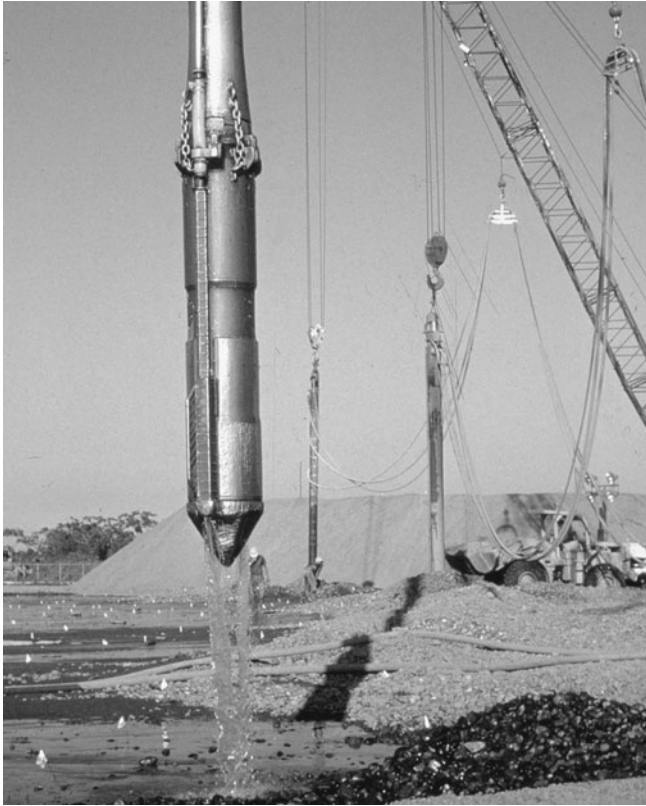
Figure 5-37 Vibrator Ready for Action with Water Jet On. (Courtesy Hayward Baker Inc.)
