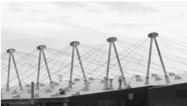
Figure 12-2 Flashing around Cable Supports.
