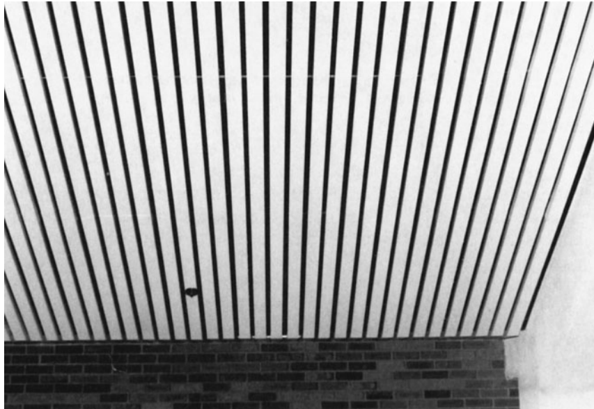
Figure 16-51 Ribbed Metal Ceiling Panels Serve as Grilles for Air Distribution.
