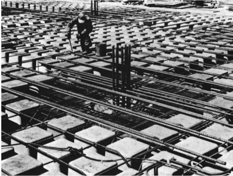
Figure 11-36 Dome Pans for Waffle Floor in Place. (Reprinted with permission of Portland Cement Association.)
