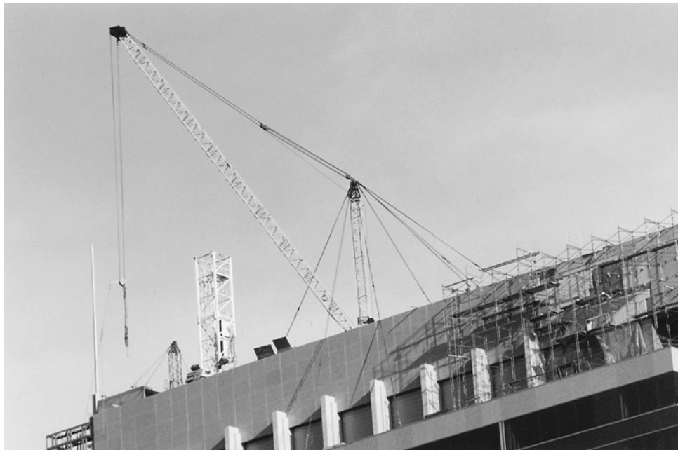
Figure 10-43 Guyed Derrick Used for Removing Tower Crane from Top of High-Rise Building.
