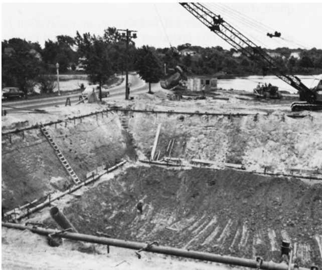
Figure 3-4 Excavation Surrounded by Well-Point System. (Reprinted by permission of Moretrench American Corporation.)
