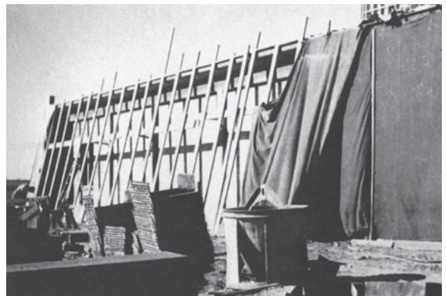
Figure 7-43 Removing Part of Protective Enclosure. (Reprinted by permission of Portland Cement Association.)
