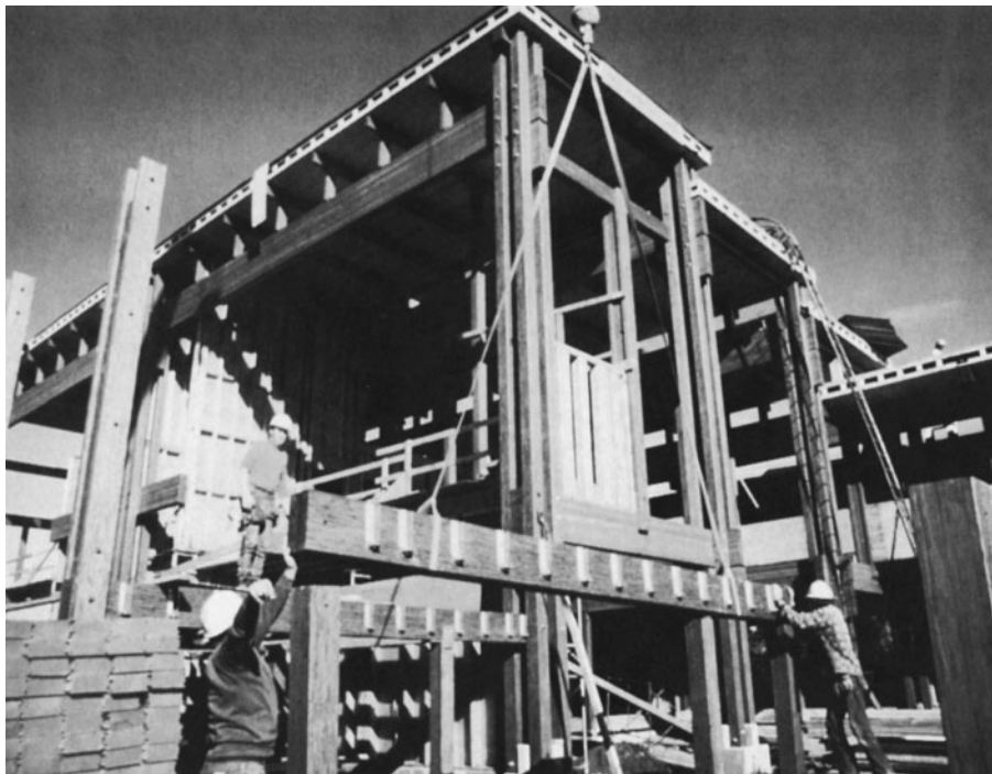
Figure 8-52 Parallel-Strand Beam Fitted with Steel Joist Hangers Being Placed into Position. (Reprinted by permission of Trus Joist, a Weyerhaeuser business.)
