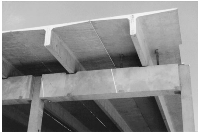
Figure 9-38 Single-T Prestressed Girders.
