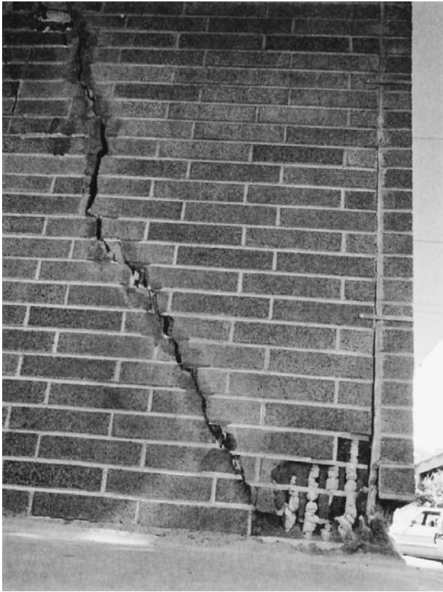
Figure 1-1 Severe Structural Damage to Building Wall Due to Unstable Foundation Conditions.
