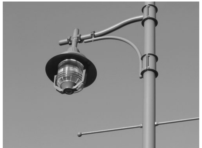
Figure 4-22 Decorative Street Lighting Fixture.
