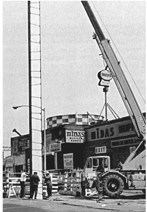
Figure 3-58 End Beam Being Lowered into Trench. (Reprinted by permission of I.C.O.S. Corp. of America.)
