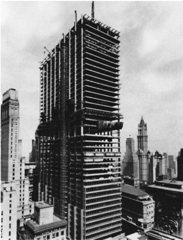
Figure 10-1 Steel Frame High-Rise Office Building. (Reprinted by permission of Bethlehem Steel Co.)
