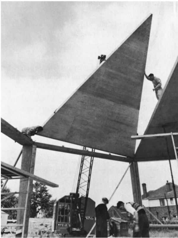
Figure 8-60 Stressed-Skin Roof Panels. (Reprinted with permission of Council of Forest Industries of British Columbia.)
