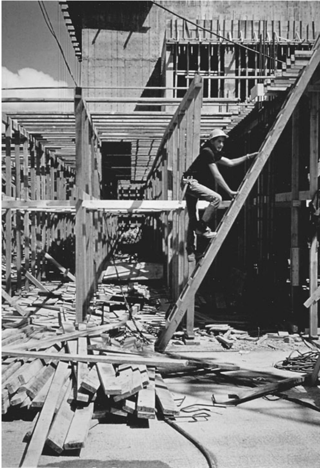
Figure 6-70 Supports for Ribbed Slab Floor.
