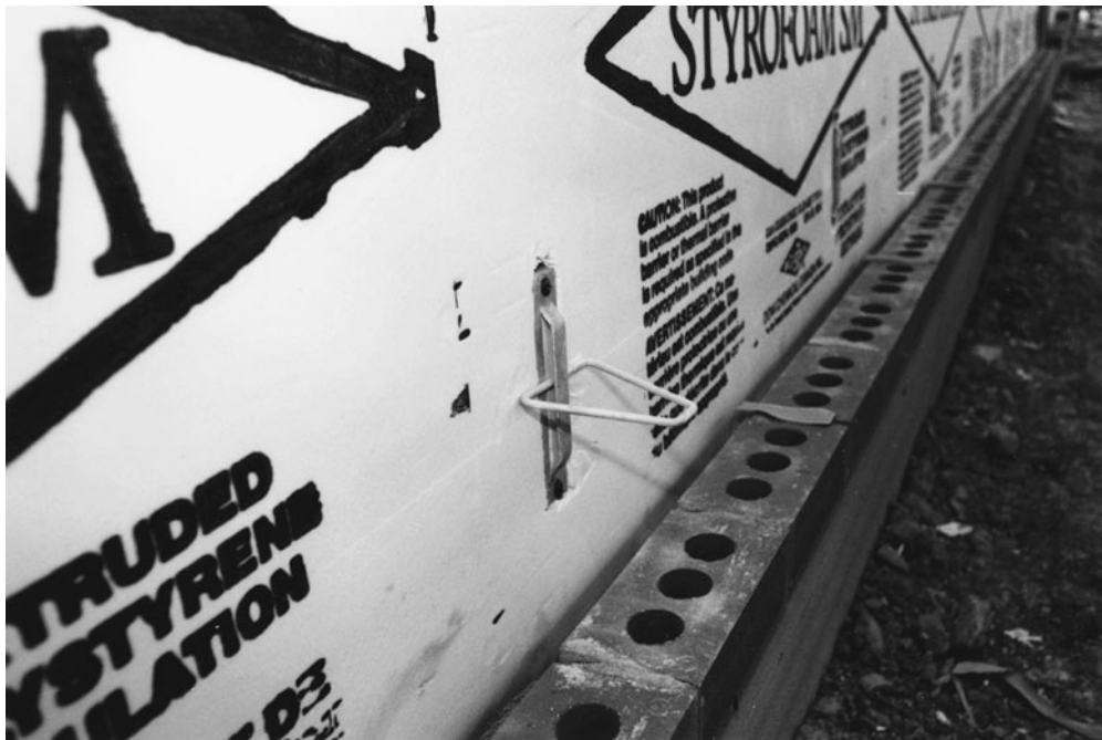
Figure 14-14 The Construction of a Brick-Faced Curtain Wall. The Brick Anchor Is Fastened through the Insulation into the Structural Frame Which Will Provide the Lateral Stability for the Brick Veneer. In This Application, the Brick Veneer Is Being Placed Directly on the Reinforced Concrete Grade Beam.
