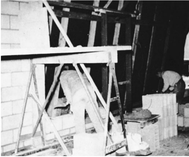
Figure 13-50 Laying Block Behind a Protecting Tarpaulin. (Reprinted with permission of Portland Cement Association.)
