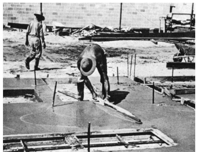
Figure 14-27 Placing Concrete for Tilt-Up Panels. (Reprinted with permission of Portland Cement Association.)
