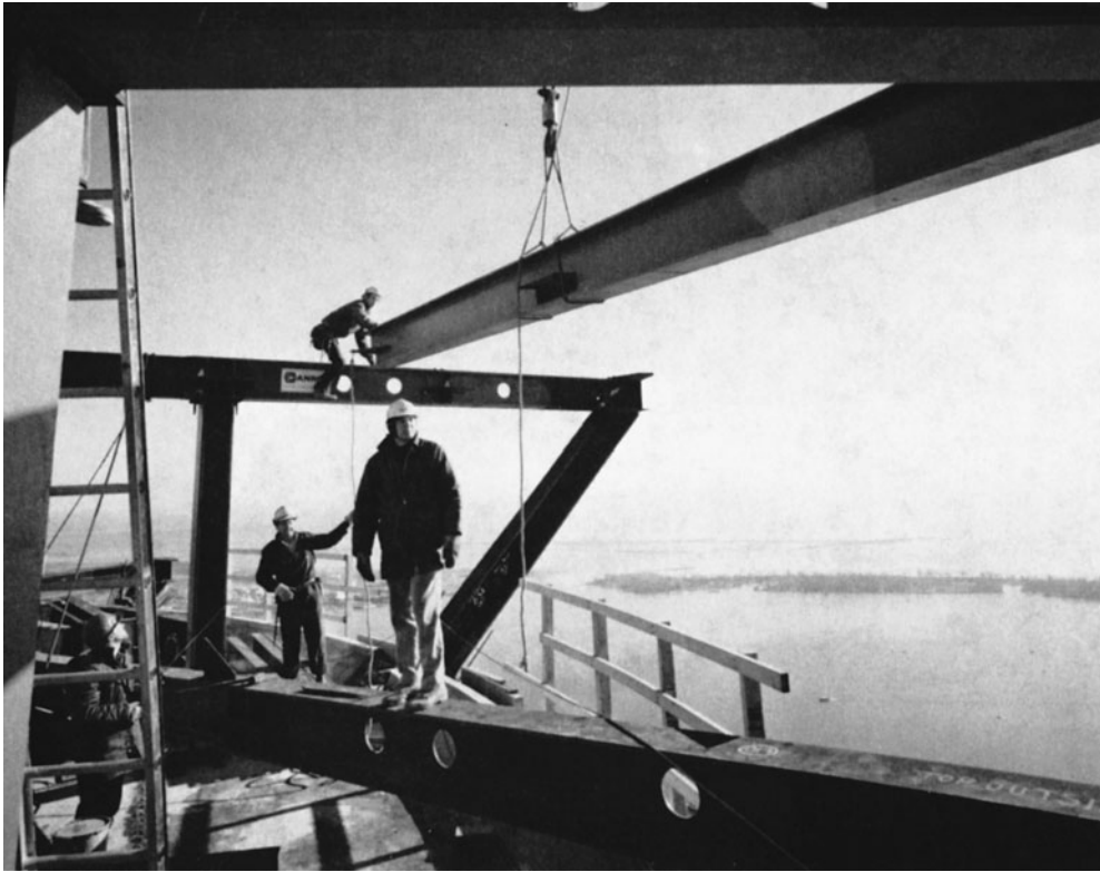
Figure 10-48 Iron Workers Erecting Steel Frame. (Reprinted by permission of Canadian Institute of Steel Construction.)
