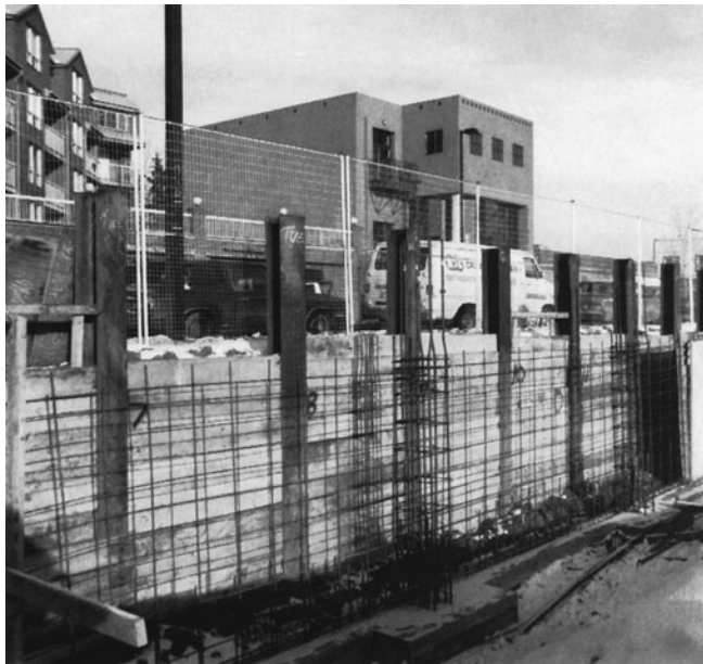
Figure 3-49 I-shaped Steel Sections and Horizontal Timbers Restrain the Soil at the Edge of the Excavation.
