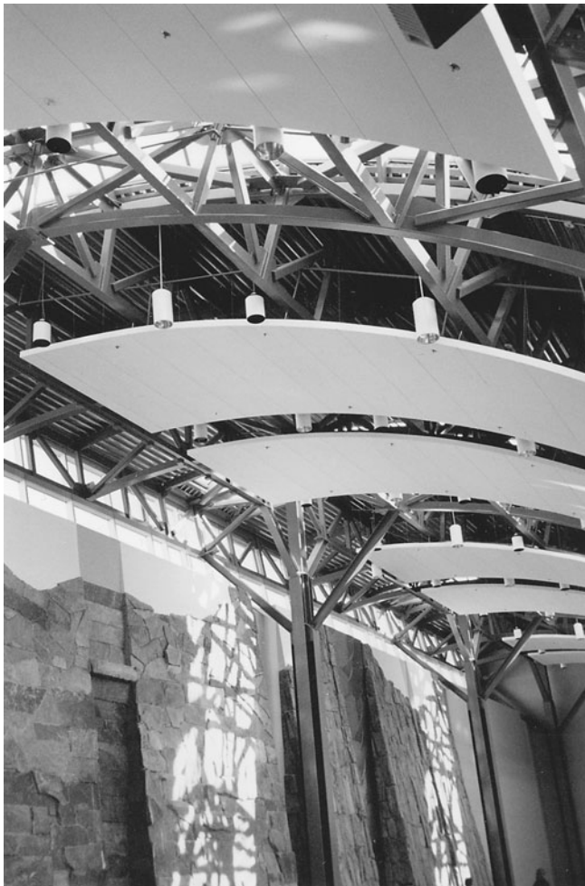
Figure 15-34 Acoustic Panels Suspended from Roof Framing in a Large, Open Area.
