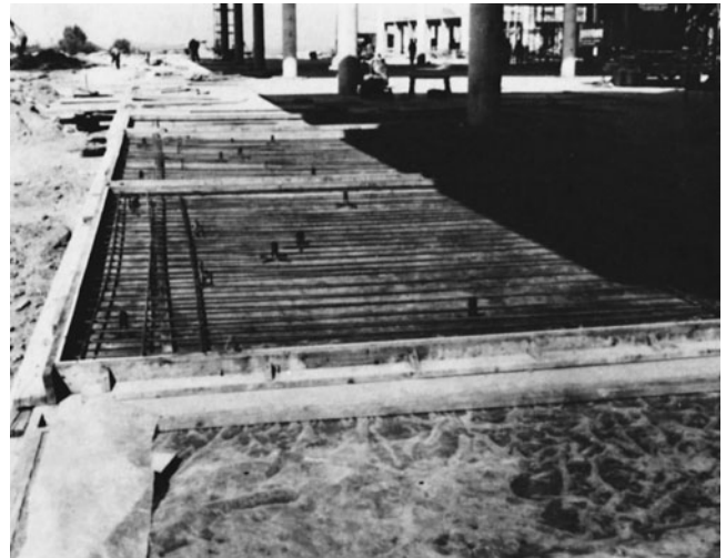
Figure 9-73 Casting Panels on Floor Slab. (Reprinted with permission of Portland Cement Association.)
