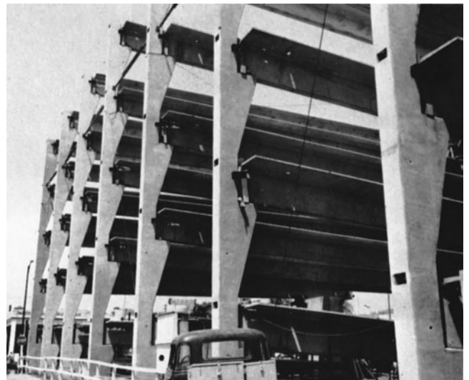
Figure 9-35 Prestressed Precast Concrete Structural Frame. (Reprinted with permission of Portland Cement Association.)
