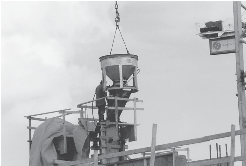
Figure 7-21 Placing Concrete into a Column Form Using a Bucket Equipped with a Chute.
