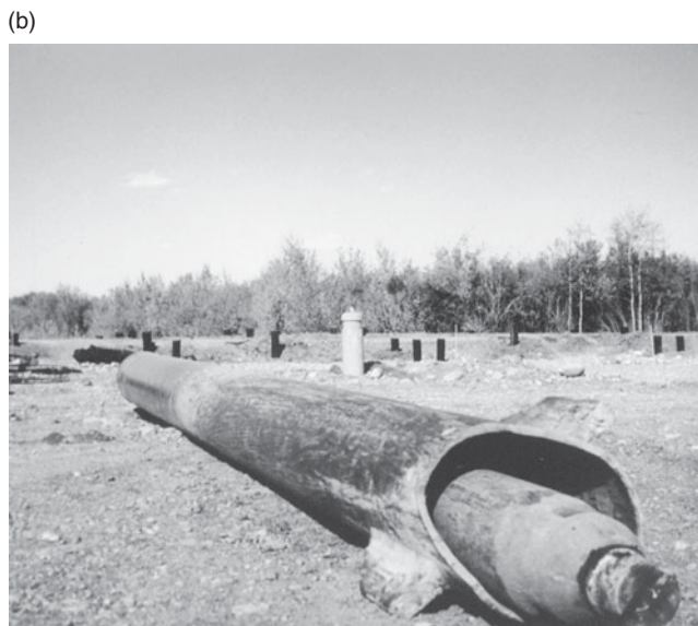
Figure 5-15 (a) Driving a Shell with Drop Hammer and Concrete Plug. (b) Typical Steel Shell with Drop Hammer.
