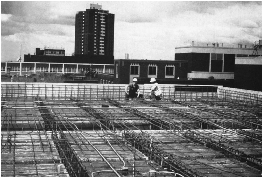
Figure 11-38 Pan Forms for a Beam and Joist Two-Way Ribbed Slab. Note the Heavy Reinforcing for the Beams.
