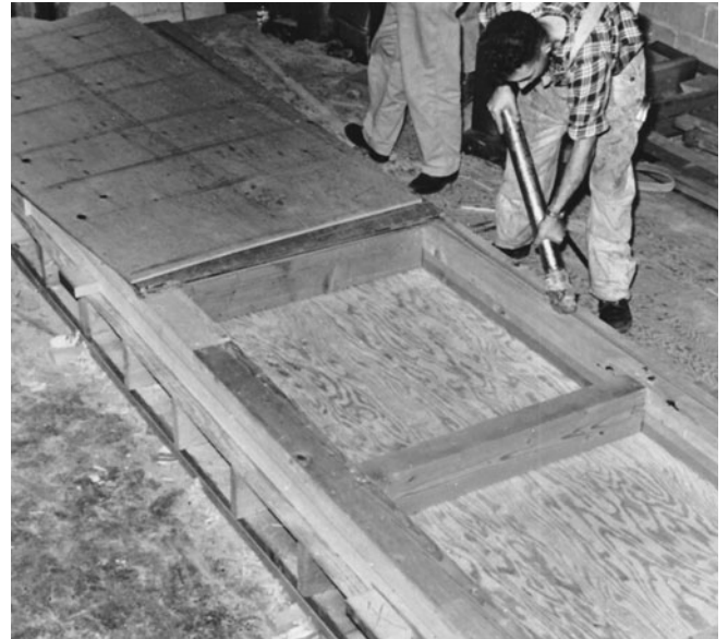
Figure 8-56 Large Plywood Web Beam under Construction. (Reprinted with permission of Council of Forest Industries of British Columbia.)
