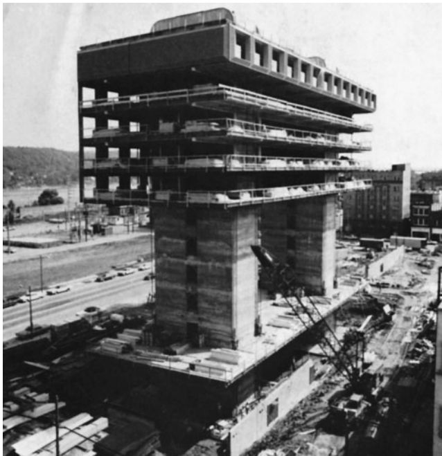
Figure 10-49 Structural Steel Floor Frames Hang from Straps. (Reprinted by permission of Bethlehem Steel Co.)
