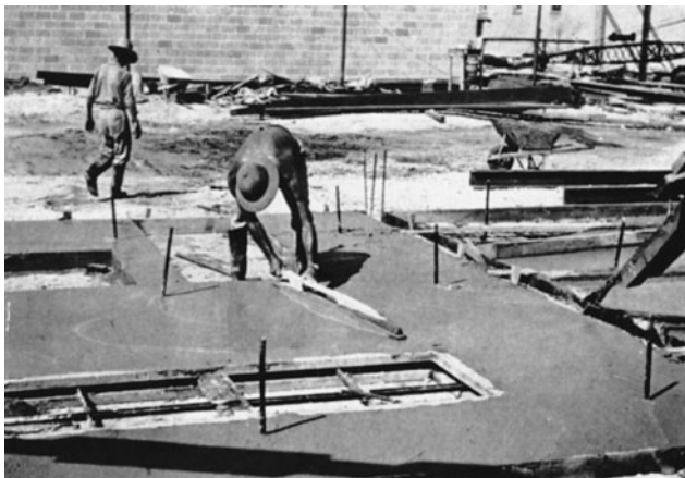
Figure 9-76 Openings Cast in Tilt-Up Panels. (Reprinted with permission of Portland Cement Association.)
