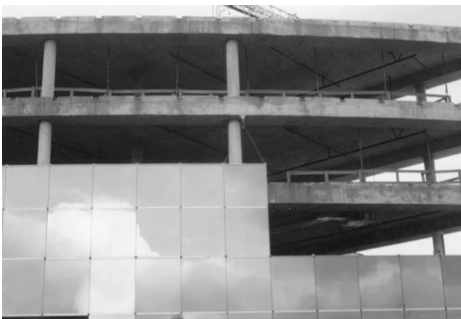
Figure 14-46 Reflective Glass Panel Curtain Wall Being Attached to Reinforced Concrete Building Frame.
