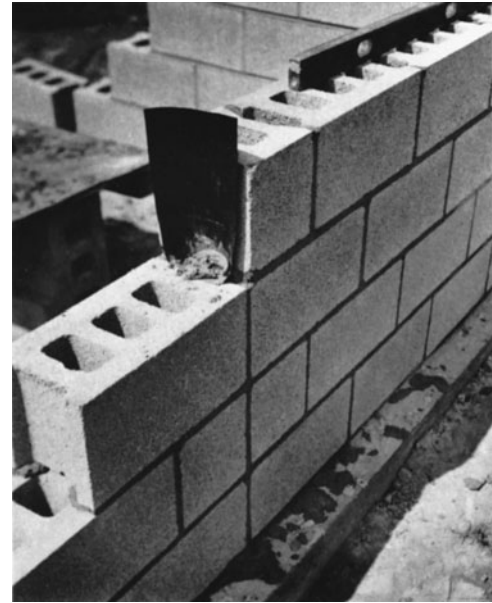
Figure 13-8 Control Joint in Block Wall. (Reprinted with permission of Portland Cement Association.)
