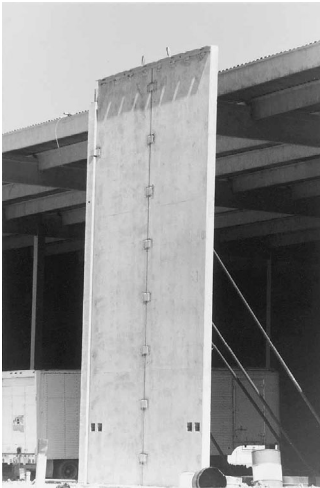
Figure 14-24 Placement of Precast Wall Panels after the Precast Concrete Frame Has Been Erected.
