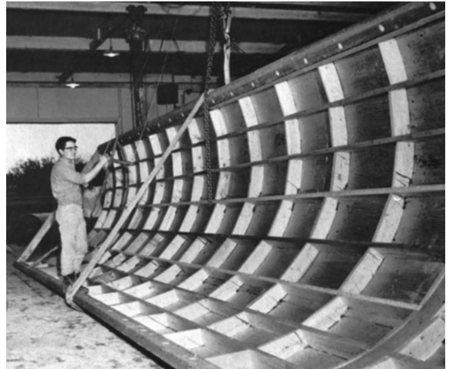
Figure 8-61 Curved Panel for Vaulted Roof. (Reprinted with permission of Council of Forest Industries of British Columbia.)
