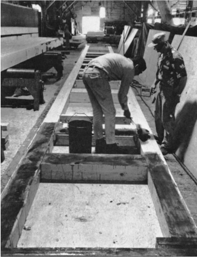
Figure 8-54 Large Box Beam under Construction. (Reprinted with permission of Council of Forest Industries of British Columbia.)
