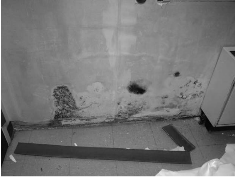
FIGURE 12.3 Moldy drywall due to moisture. (Courtesy of Gobbell Hays Partners, Inc.)
