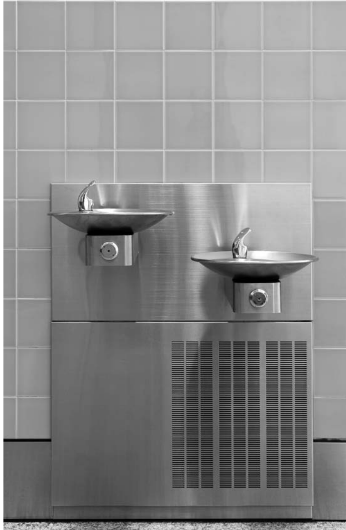
FIGURE 2.9 Combination accessible and normal height drinking fountain.
