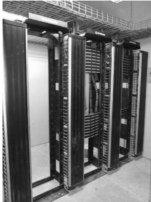
FIGURE 11.20 Technology equipment room.
