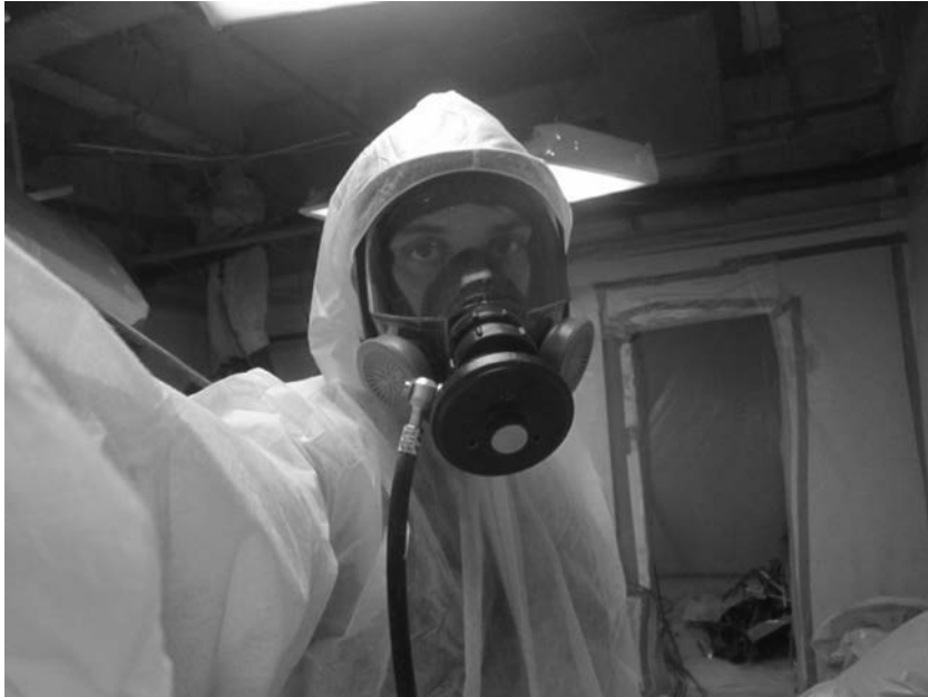
FIGURE 12.7 Type C respiratory protection for asbestos abatement of sprayed on fireproofing. (Courtesy of Gobbell Hays Partners, Inc.)
