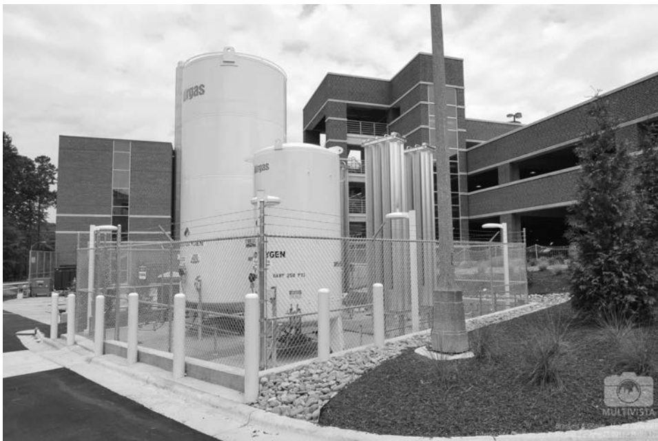
FIGURE 9.2 Tank farm for medical gas behind central energy plant. (Courtesy of Multivista and Moses Cone Hospital.)
