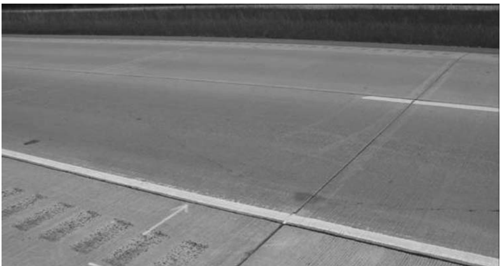
Figure 3. Characteristic pattern of edge-restraint cracking.
