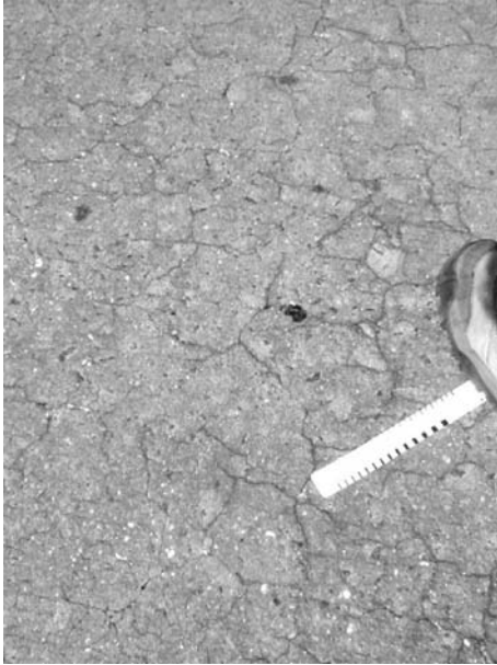
Figure 1. Map cracking in a concrete pavement.
