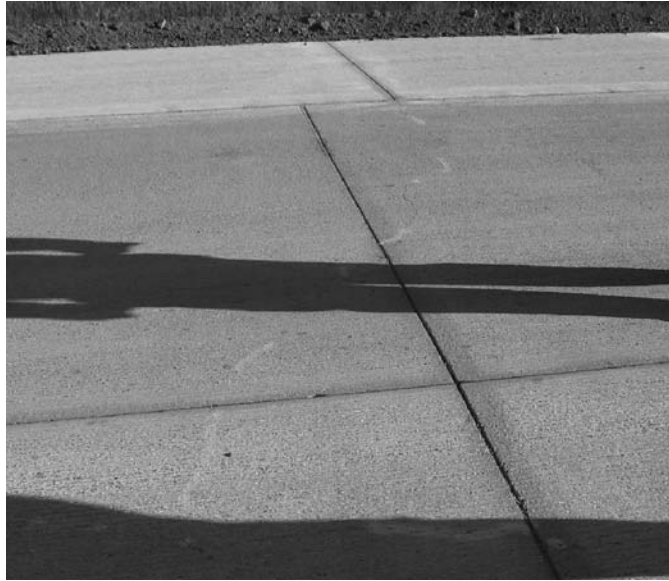
Figure 6. Cracking along a transverse sawcut on I-94, North Dakota.
