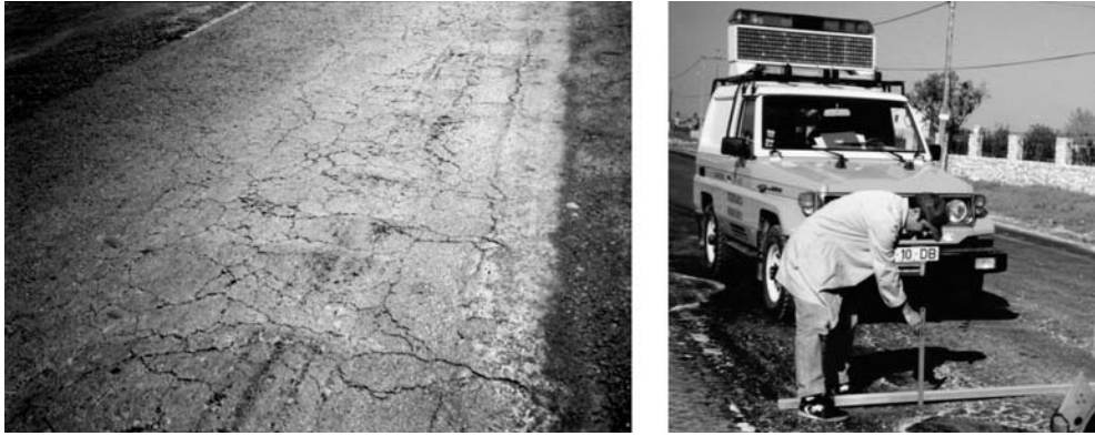
Figure 1. Pavement condition before rehabilitation.
