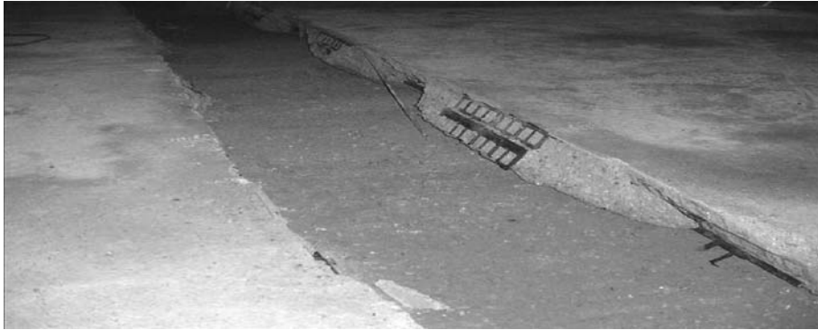
Figure 3. Crack shape between slabs.
