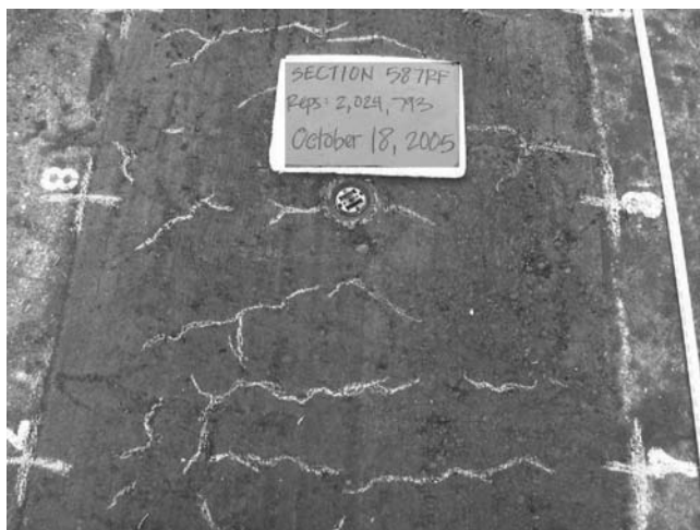
Figure 3. Typical fatigue cracking on HVS test section (RAC-G section).
