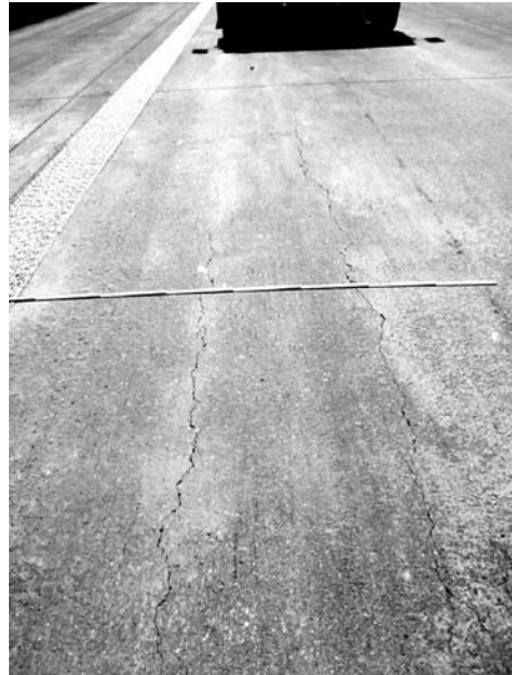
Figure 2. Transversal longitudinal cracks in a concrete pavement.
