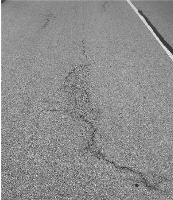
Figure 1. Cracking on Quivira Road.
