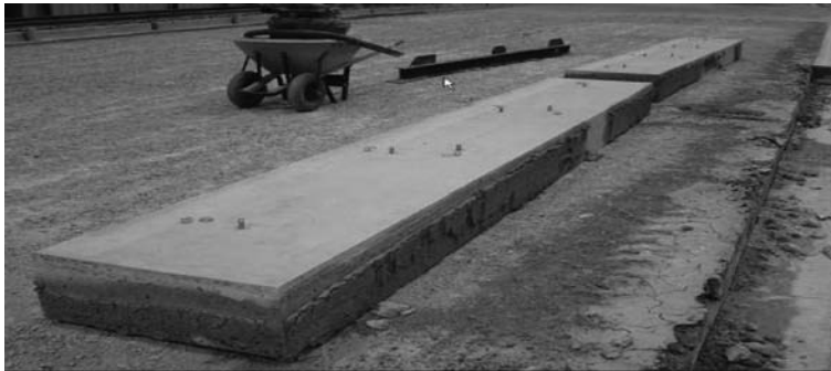
Figure 2. Strip 30.5 cm (12 inch) wide by 22.86 m (5 slabs length, 75 ft) were saw-cut and removed.
