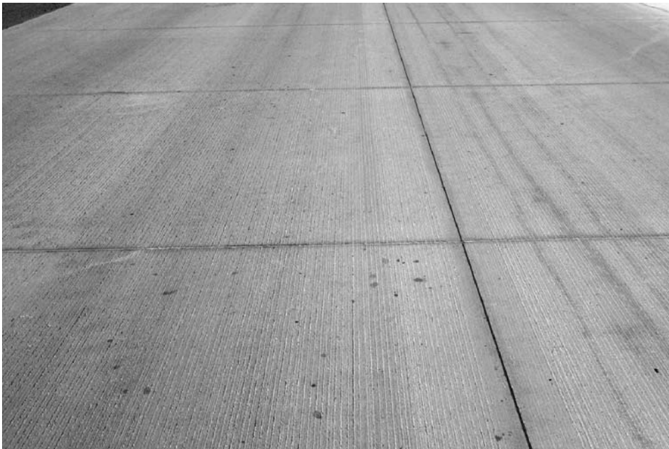
Figure 5. Early-age, longitudinal cracking on I-94, North Dakota.
