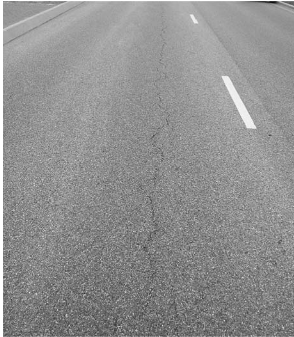
Figure 2. Cracking encountered on 127th Street.
