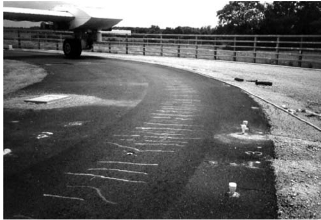
Figure 6. Transversal cracking observed on structure 9.
