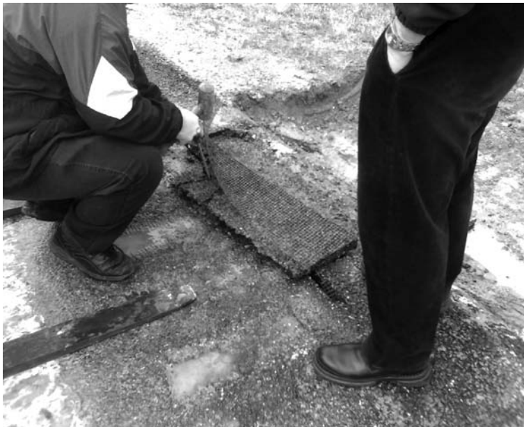
Figure 8. Geogrid sample recovery during forensic study.
