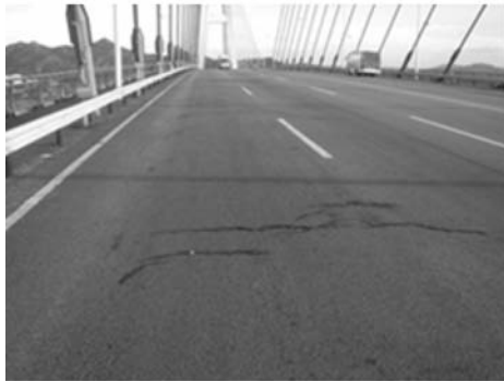
c: SMA transverse crack
