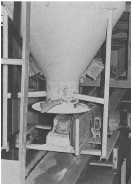
Fig. 29. Additive hopper and feeder for introducing barium carbonate to the clay blend
