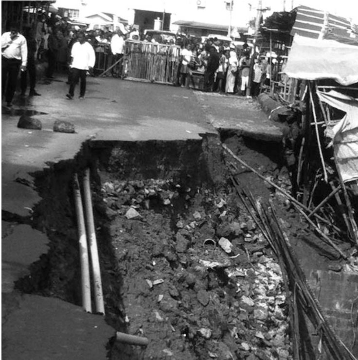
Fig. 10.2 Sierra Leone's collapsed King Jimmy bridge along Wallace Johnson Street in Freetown, August 2013
