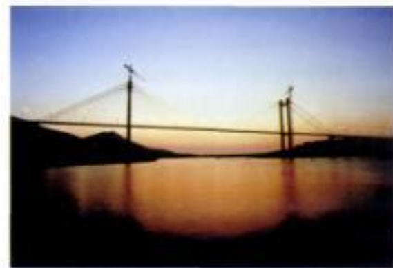
8.54-8.56 Views of Evripos bridge during free cantilevering construction and after completion in 1992
