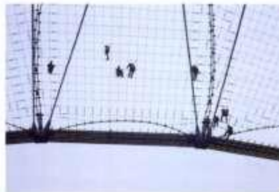
5.15 The main multiple cable forming the edge of the stadium roof and the adjacent cable nets (see 5.41)
