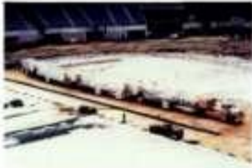
7.21 Transport of the membrane into the stadium (compare the size of the truck)
