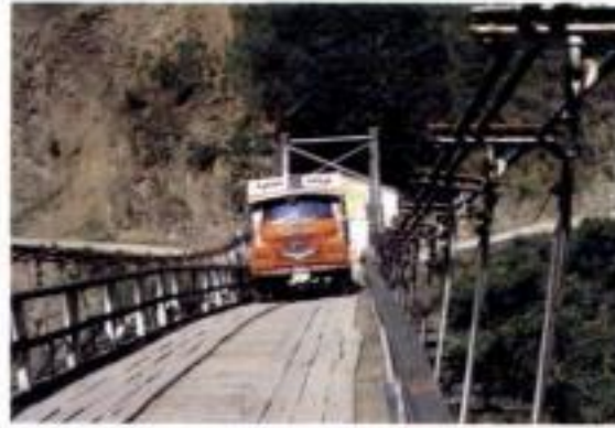
8.39 Akkar: the old suspension bridge sloping and listing heavily under the weight of a truck
