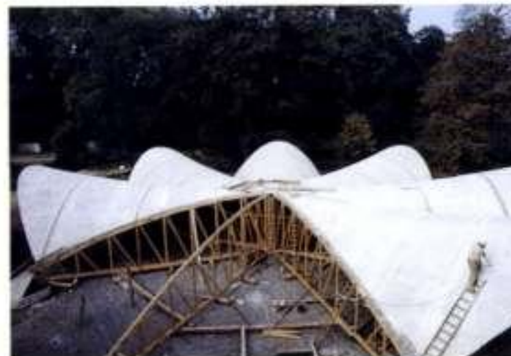
Six segments in their final position temporarily supported only at their common edges
