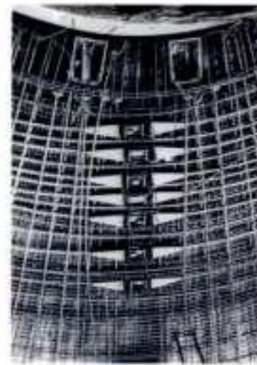
3.7 Cables and anchorages for circumferential prestressing of a platform (view from above)
