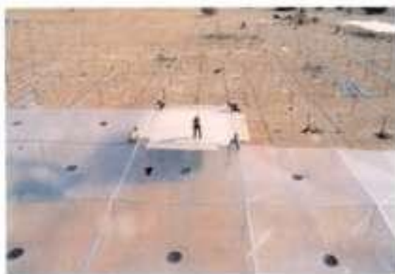
11.46 + 11.47 Fabrication of the initial plastic collector roof (diameter 250 m) by unskilled labour.
