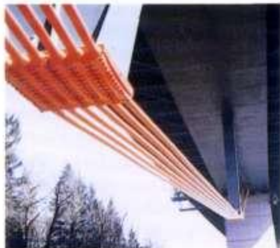
8.62 The inverted saddles at the lower end of the vertical and the V-shaped props
