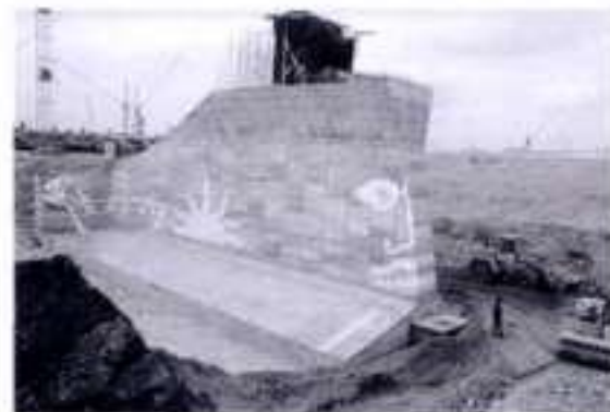
5.17 The huge anchor block for the main cable of the stadium roof, designed to resist a horizontal force of about 4500 tons
