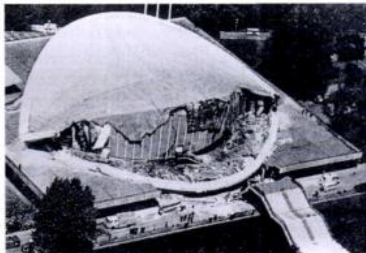
4.42 Bird's eye view showing the collapsed arch
