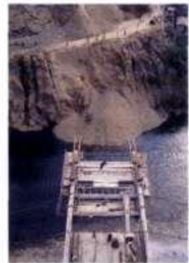
B.42 + B.43 Construction of the deck as bal- anced cantilevers using simple concreting gantries
