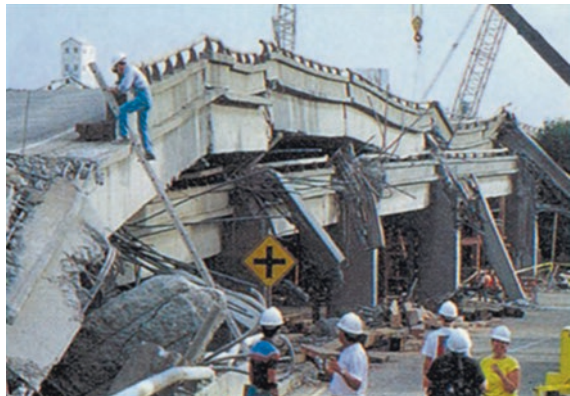
Fig. 3.15 Collapse of the MacArthur Maze (Cypress Viaduct) in Oakland from the 1989 Loma Prieta earthquake
