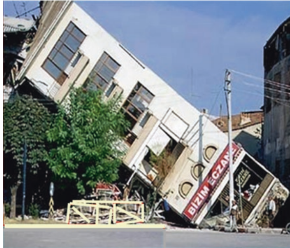
Fig. 3.14 Liquefaction of the subsurface strata from the earthquake event in 1999 made this masonry structure collapse (Adapazari; Turkey)
