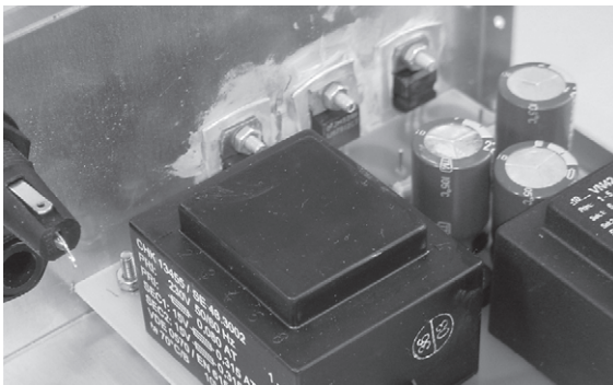
FIGURE 6.29 Showing three components, heatsinked to a metal housing panel.
