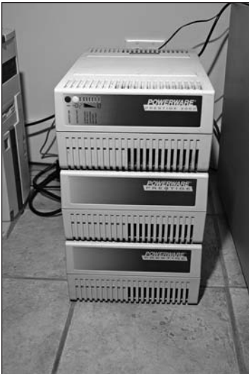
Figure 6-26: Uninterruptible power supply (UPS)
