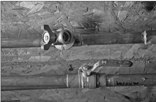
Figure 15-21: Valves at the end of irrigation piping
