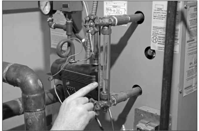
Figure 10-29: Sight glass on a steam boiler
