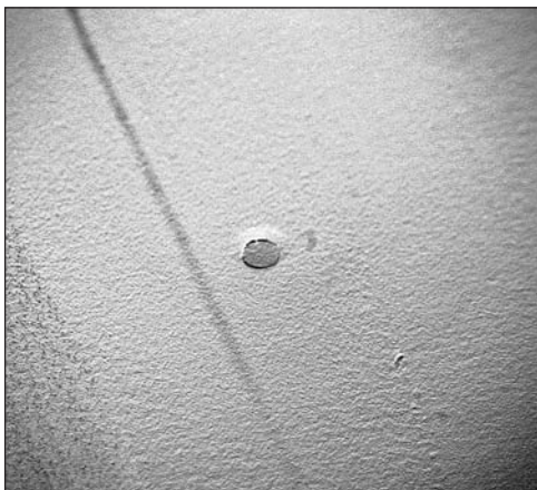
Figure 8-1: Wall with nail holes
