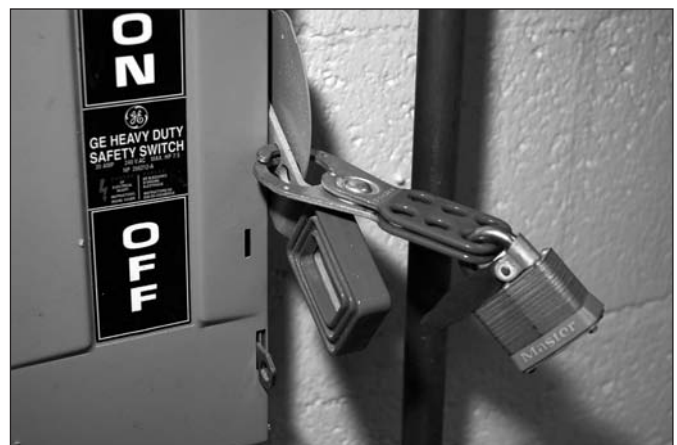
Figure 12-4: After disconnecting the power to the compactor, locking out the distribution panel prevents someone from turning on the power
