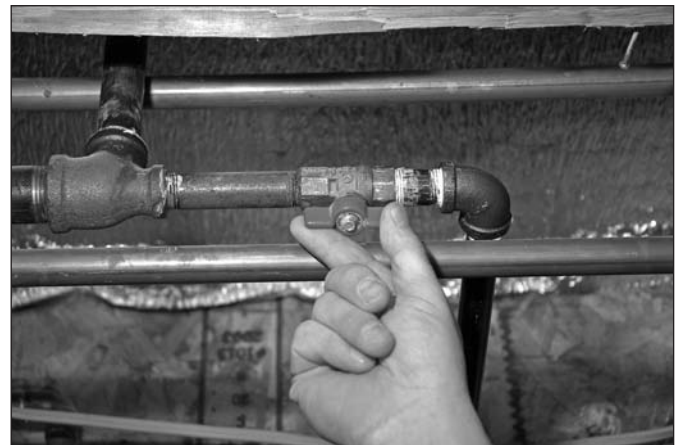
Figure 11-7: Turn off gas line
