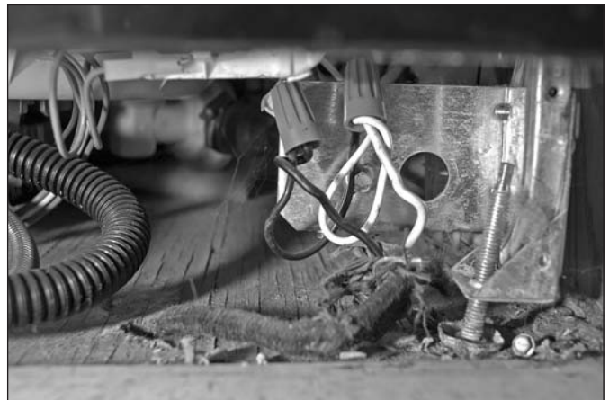
Figure 11-35: Electrical box on dishwasher
