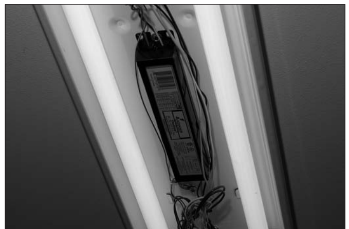
Figure 6-52: Ballast on a fluorescent fixture
