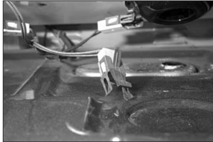
Figure 11-22: Cooktop lifted to access receptacle wiring
