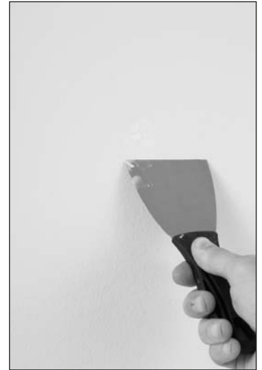
Figure 8-2: Repairing flaws in the wall (Image copyright Mark Stout Photography, 2009. Used under license from Shutterstock.com)
