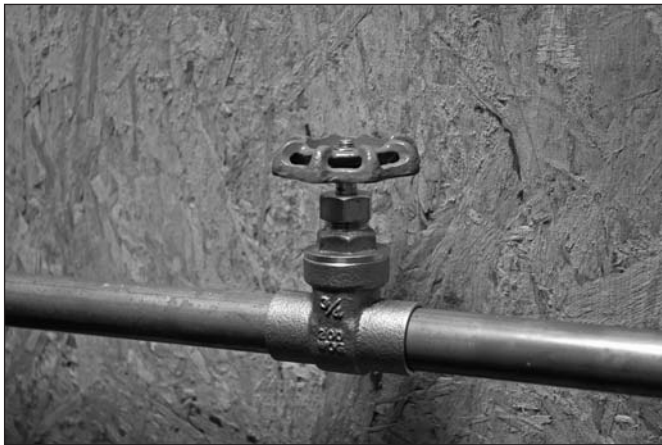
Figure 15-15: Valves on the irrigation piping
