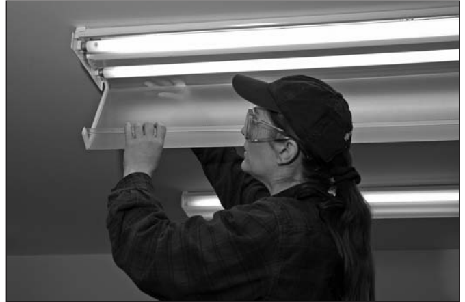
Figure 6.51: Lens/diffuser on a fluorescent fixture
