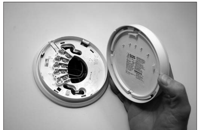
Figure 6-42: Mounting base still attached to box
