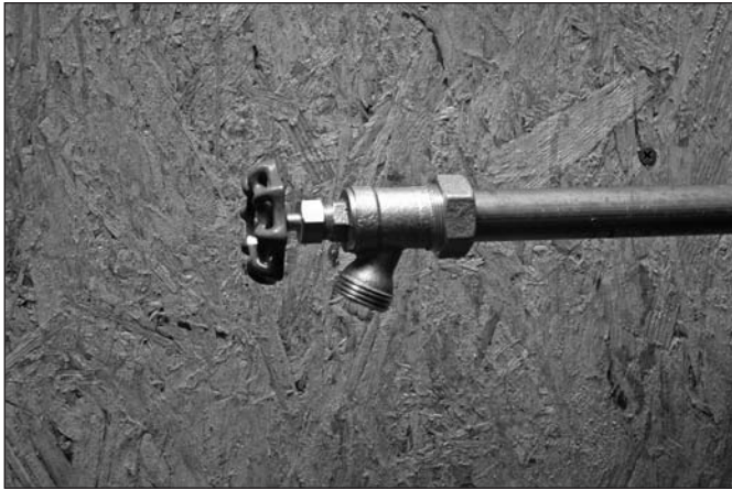
Figure 15-19: Boiler drain valve/drain cap
