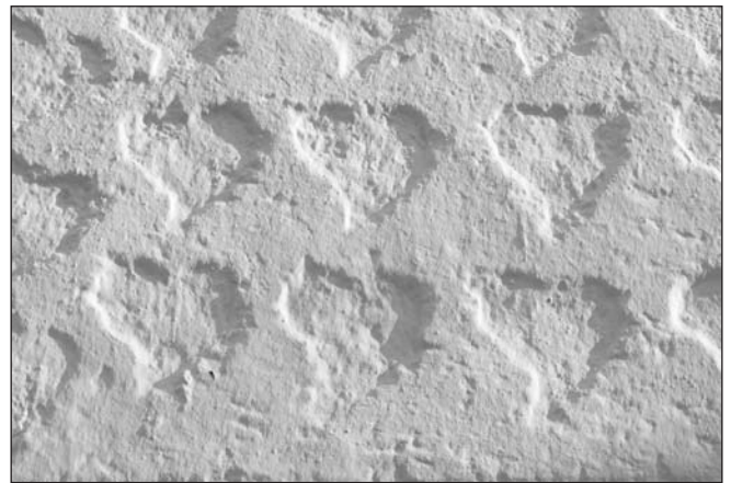
Figure 8-63: Stamp texture on drywall (Image copyright Carsten Medom Madsen, 2009. Used under license from Shutterstock.com)
