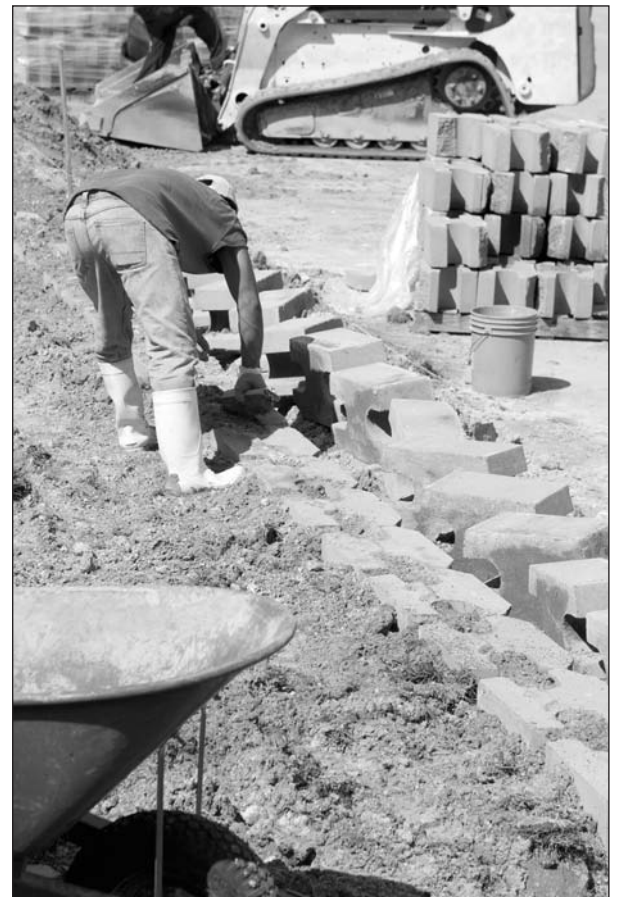
Figure 15-11: Cinder block retain wall (Image copyright Steven Frame, 2009. Used under license from Shutterstock.com)
