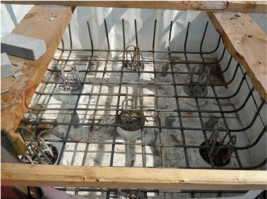
Plate 14.1 Pile cap before concreting (piles are seen at the bottom of the pile cap).
