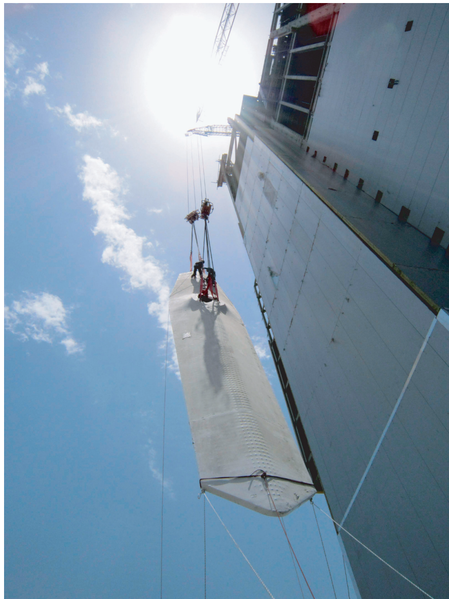
Figure 16.1 Dokaee Clock Tower, Mecca, KSA: clock hand being lifted into position (Courtesy of Premier Composite Technologies)
