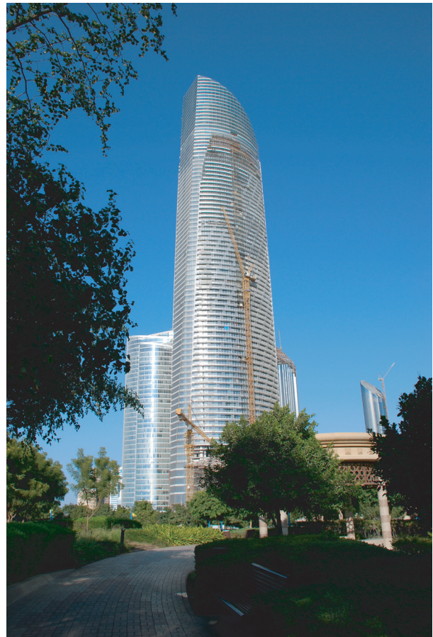
Figure 16.5 The Landmark under construction in Abu Dhabi, UAE (Courtesy of Malcolm White/Buro Happold)
