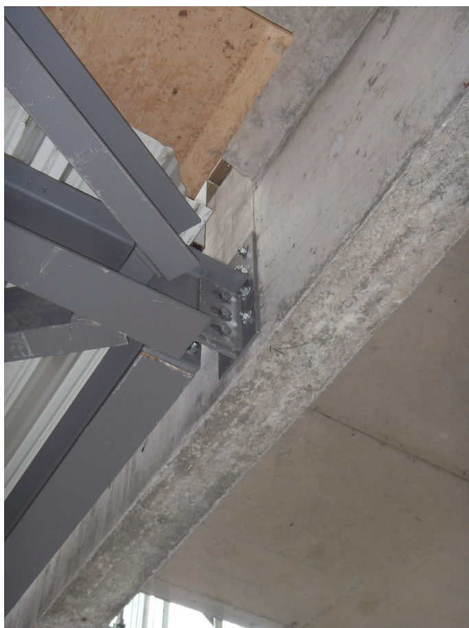
Figure 18.29 Concrete drilled in fixing with slotted steel fin, three steel-to-steel connections with a single steel to concrete connection to simplify tolerance design
