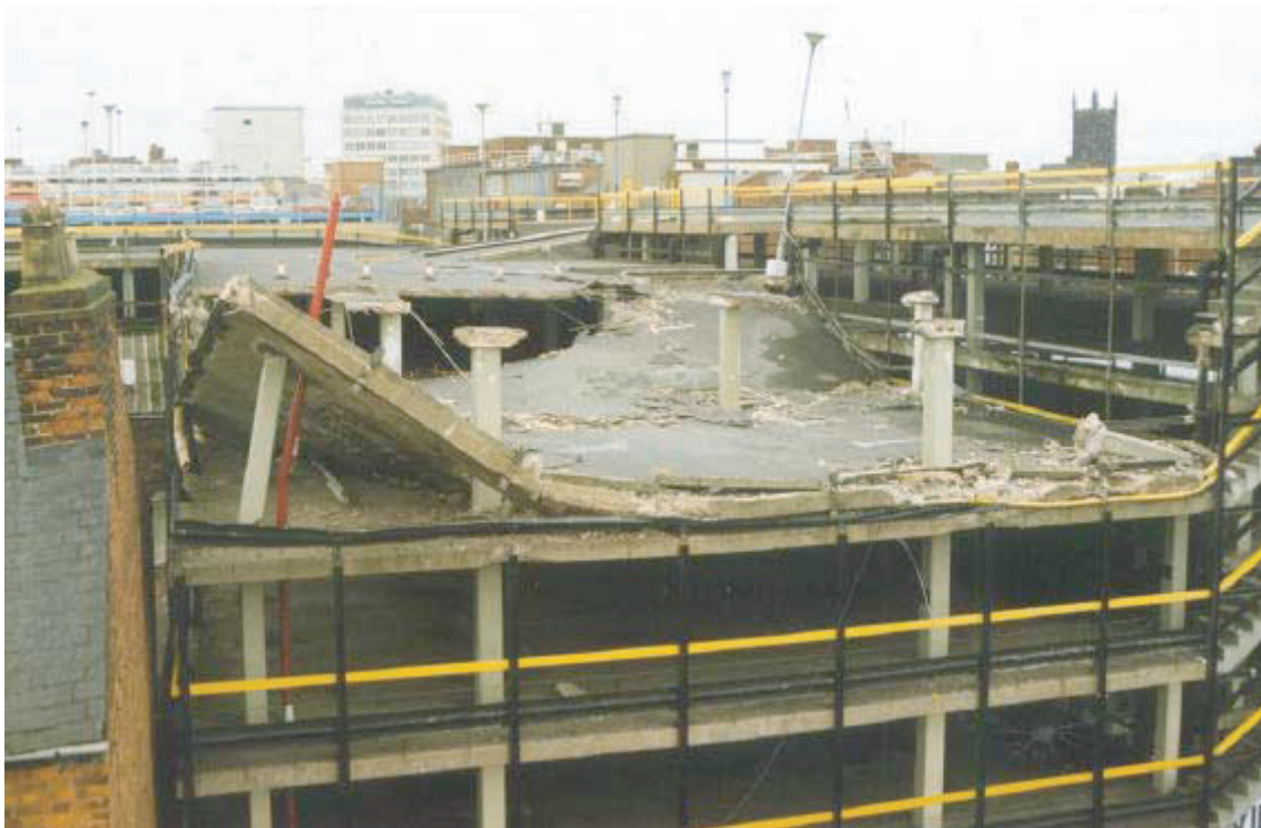
Figure 9.2 Punching shear failure at Pipers Row car park, Wolverhampton © Dr J Wood
