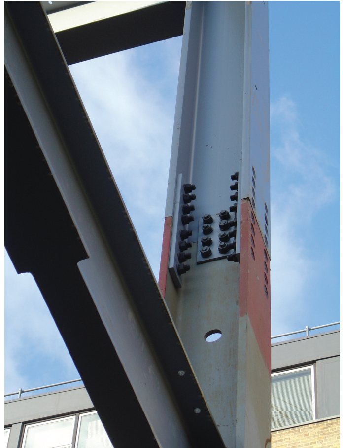
Figure 18.27 Exemplary substructure/steel interaction tolerance control on the verticality of steel plunge pile heads (painted red, note web hole for lifting pin) connected to the superstructure
