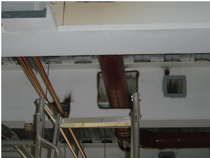
Figure 18.42 This example of site burnt out web holes shows what can happen if coordination is not clearly communicated, leading in this case to costly remedial work
