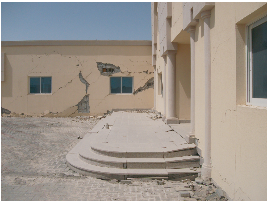
Figure 16.4 Building movement due to limestone cavity collapse, Abu Dhabi, UAE (Courtesy of Buro Happold)
