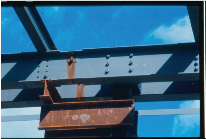
Figure 18.16 Temporary works integrated into the permanent works can be cost effective solutions to high level access – in this case a site weld 15 m above ground level
