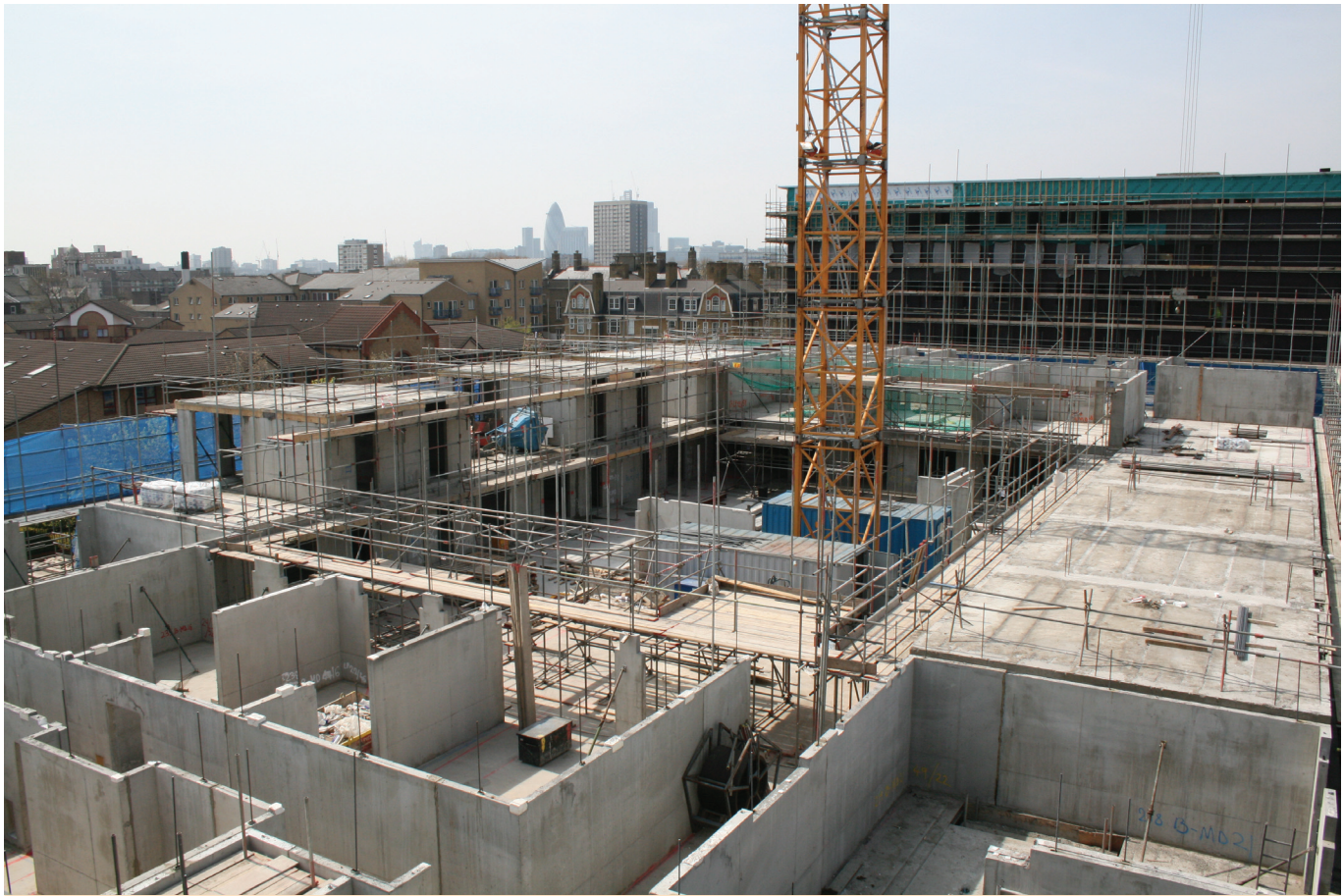
Figure 15.31 Cross walls in precast concrete residential building. Courtesy of GPS Precast Concrete Specialists
