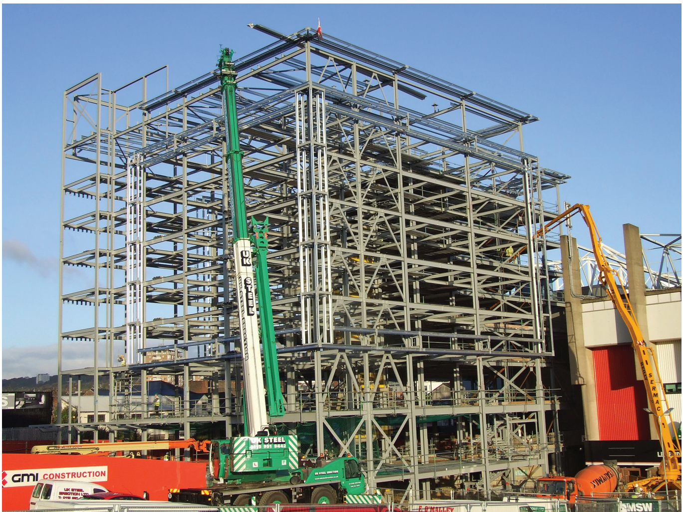
Figure 15.26 Vertical bracing to multi-storey steel framed building. Courtesy of Elland Steel Structures Ltd
