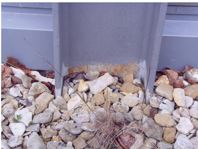
Figure 18.35 Exposed steelwork can become a maintenance problem as this 10-year-old example shows; galvanising should be considered the norm for any external steelwork
