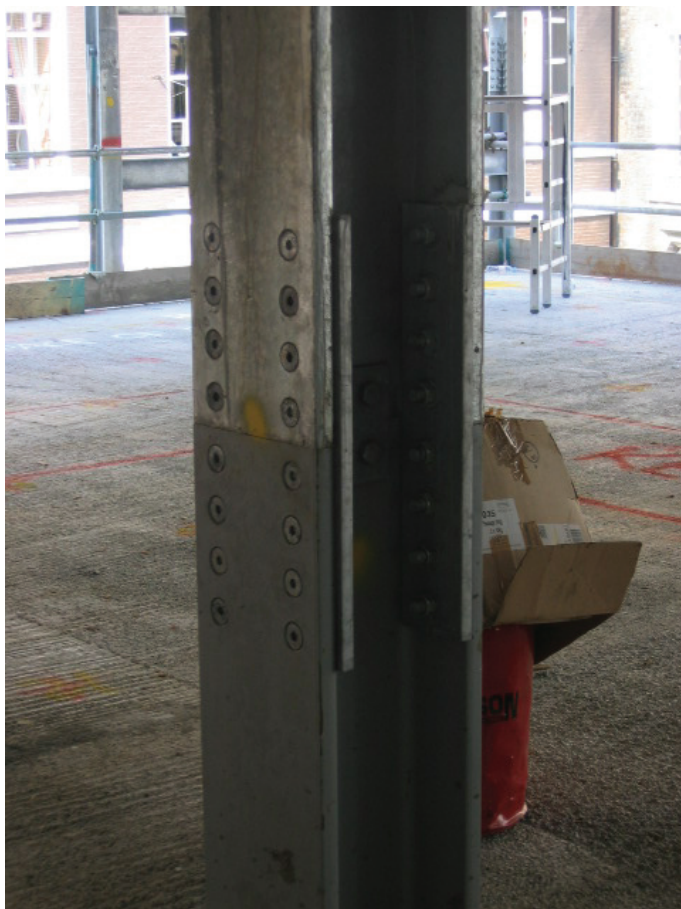
Figure 18.24(a) Compact steel detailing at column splice positions avoids costly change to column casings and ceiling detailing
