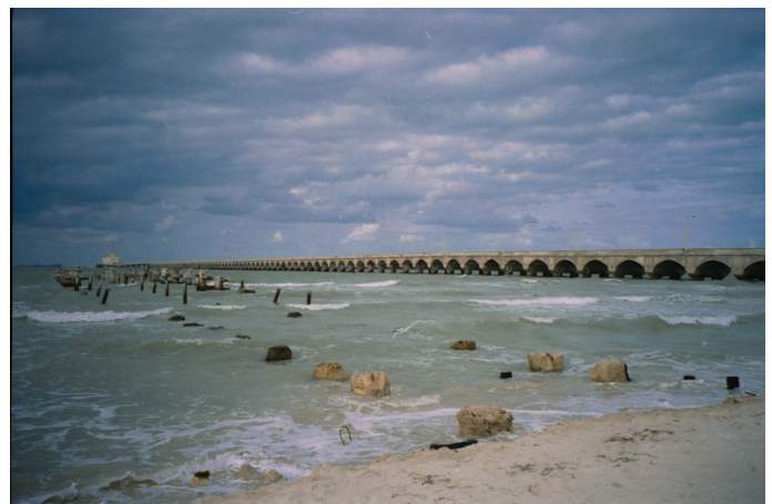
Figure 5.5(c) Progreso piers Original 1940s stainless steel reinforced Progreso pier, with the remnant of the 'modern' carbon steel reinforced 1970s neighbouring pier shown in the foreground (Knudsen et al. , 1999). Courtesy of Arminox A/S, www.arminox.com
