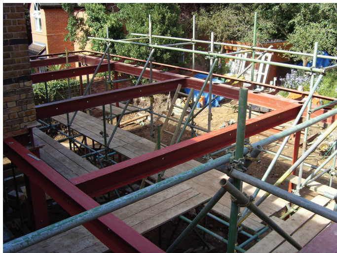
Figure 18.28 Web holes predrilled for through bolting of timber plates to fit timber joists at the same level as the steel
