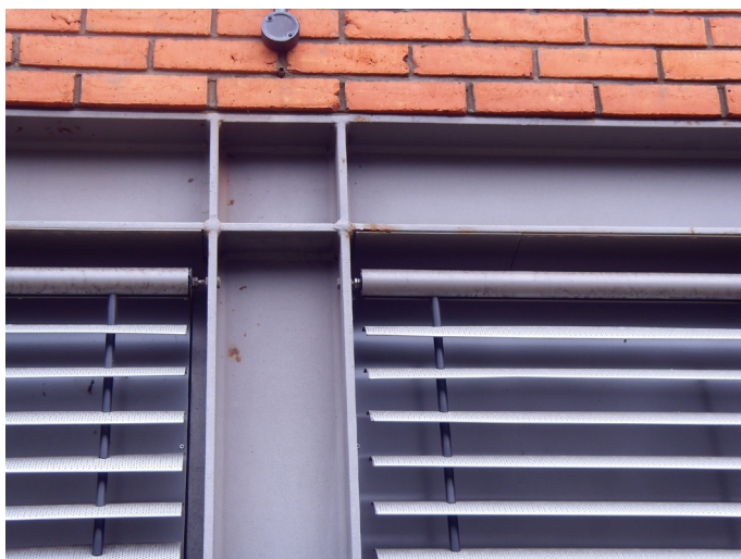
Figure 18.34 Exposed steelwork can become a maintenance problem
