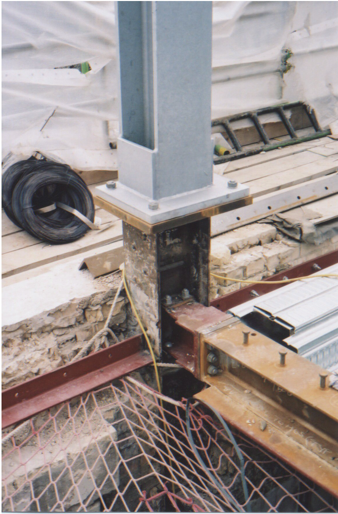
Figure 18.52 Replication of the original angle cleat connections with a stub to aid erection
