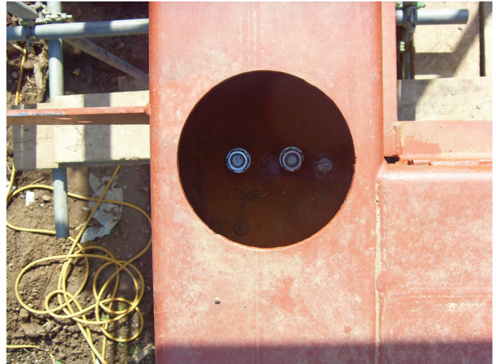
Figure 18.32 Plan on welded corner junction of 200 × 200 SHS, expensive mitred corner detail avoided avoiding problems connecting the 2-bolt post connection from below
