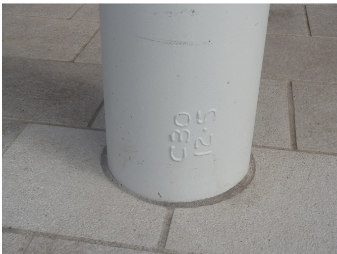
Figure 18.31 Uncontrolled fabrication marks in finished steelwork
