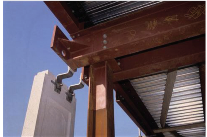
Figure 18.37 This heavy beam end connection provided support to both horizontal and vertical precast concrete cladding, some of the units weighing 8 tonnes, spanning 7.5 m
