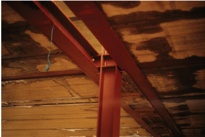
Figure 18.10(a) Parallel continuous UC sections (concrete infill between) used with precast planks
