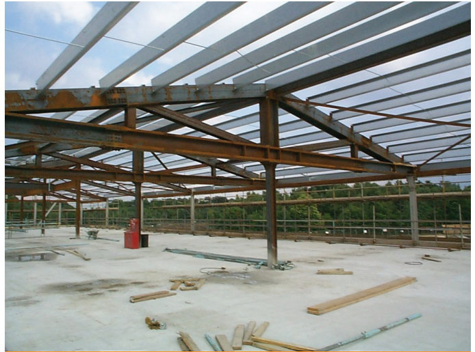
Figure 18.20 This truss was suspended two floors off a centre tie as the ground floor column was omitted. Requiring minimal deflection for compatibility with columns and too heavy for the fabricator to make in one piece, 2 no HSFG splices were used at each end
