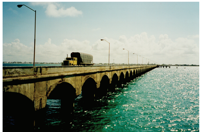
Figure 5.5(b) Original 1940s Progreso pier This is still in service after exposure to the very aggressive marine environment of the Gulf of Mexico for over 60 years
