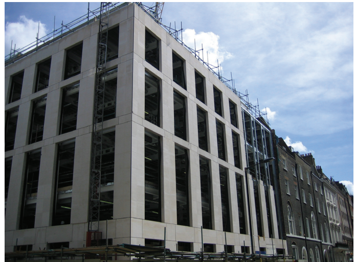
Figure 18.38 Storey height precast cladding units supported off the minus one level restrained by steel frame; avoids need for frame to support heavy edge loading
