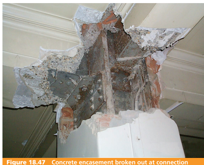
Figure 18.47 Concrete encasement broken out at connection
