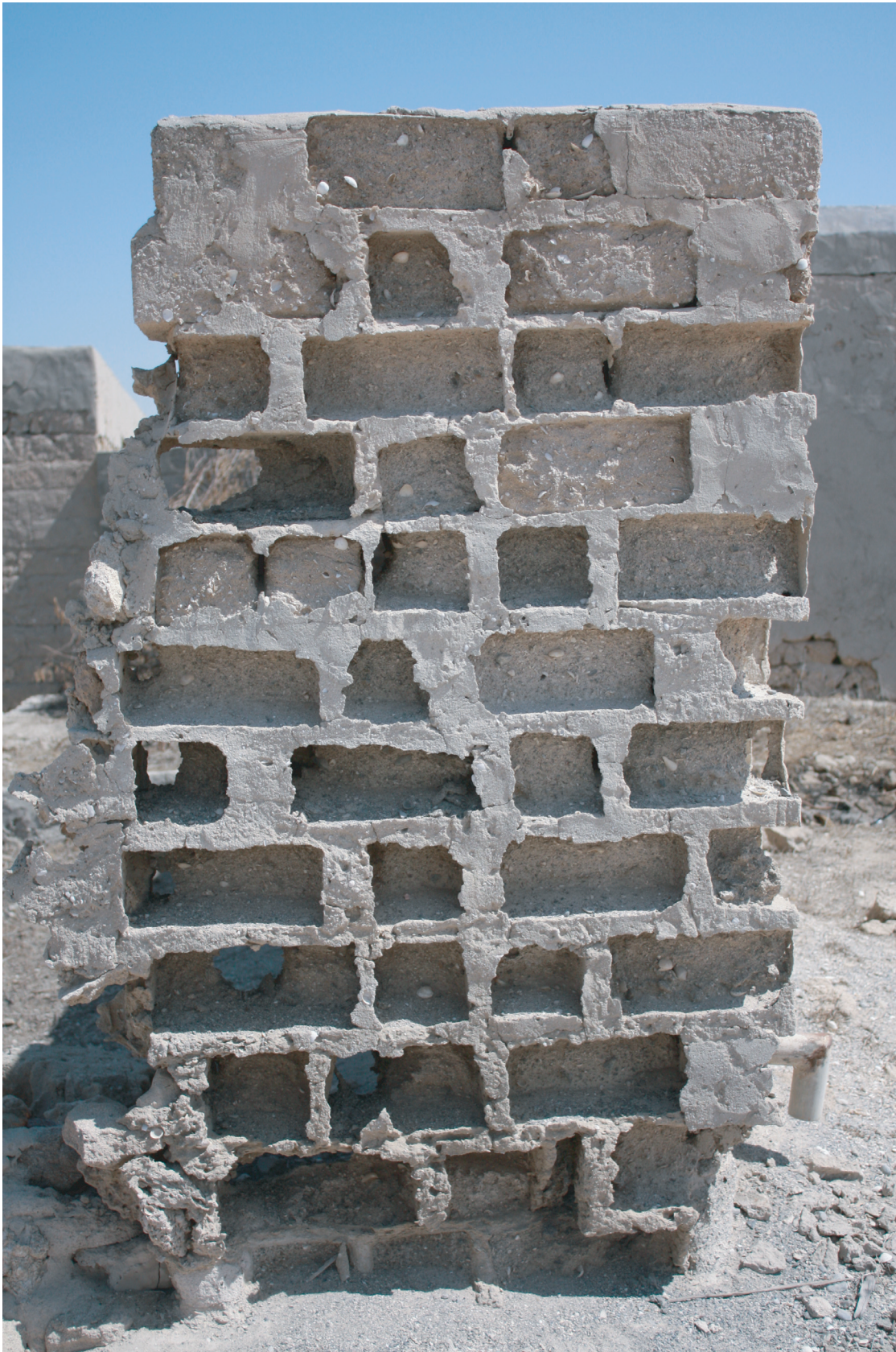
Figure 16.3 Groundwater salt attack on a masonry wall; the stronger mortar is left in situ whilst the blocks have slowly degraded, Ras Al Khaimah, UAE (Courtesy of Buro Happold)
