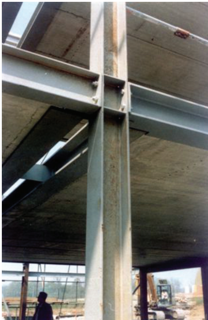
Figure 18.10(b) Parallel continuous UC sections (concrete infill between) used with precast planks
