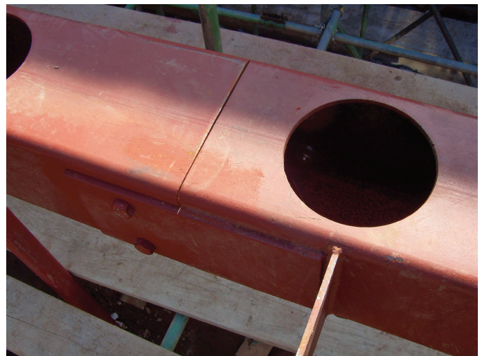
Figure 18.33 Near perfect splice fit achieved because the same piece of SHS has been used for both sides of the splice; note longitudinal seam in this section, good for accuracy but might compromise aesthetics if exposed
