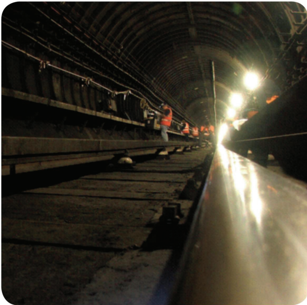
Figure 13.20 Installation of automated monitoring equipment within a London Underground tunnel underlying a new commercial development
