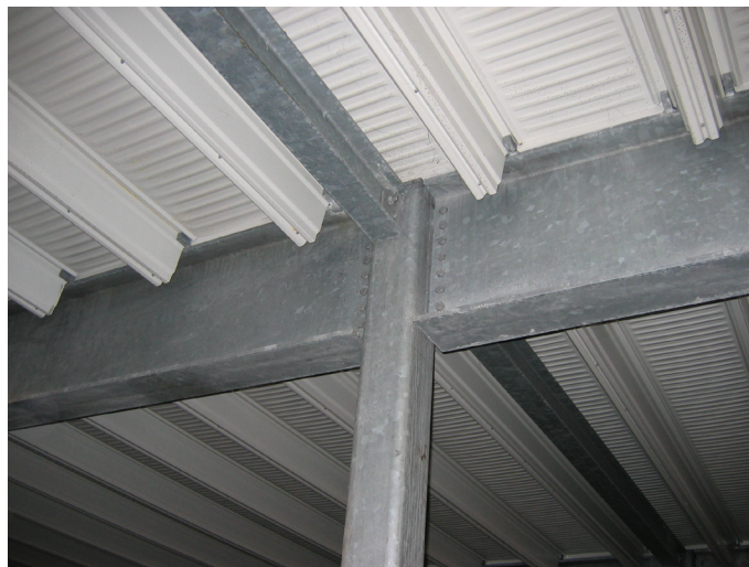
Figure 18.2 Cost-effective detailing exploiting hollow sections, simple joints and corrosion addressed with galvanising
