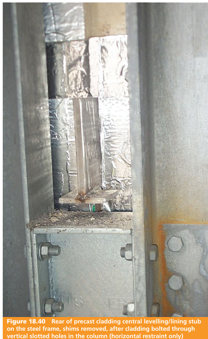
Figure 18.39 Rear of storey height precast cladding before removal of the erection shims; see Figure 18.40
