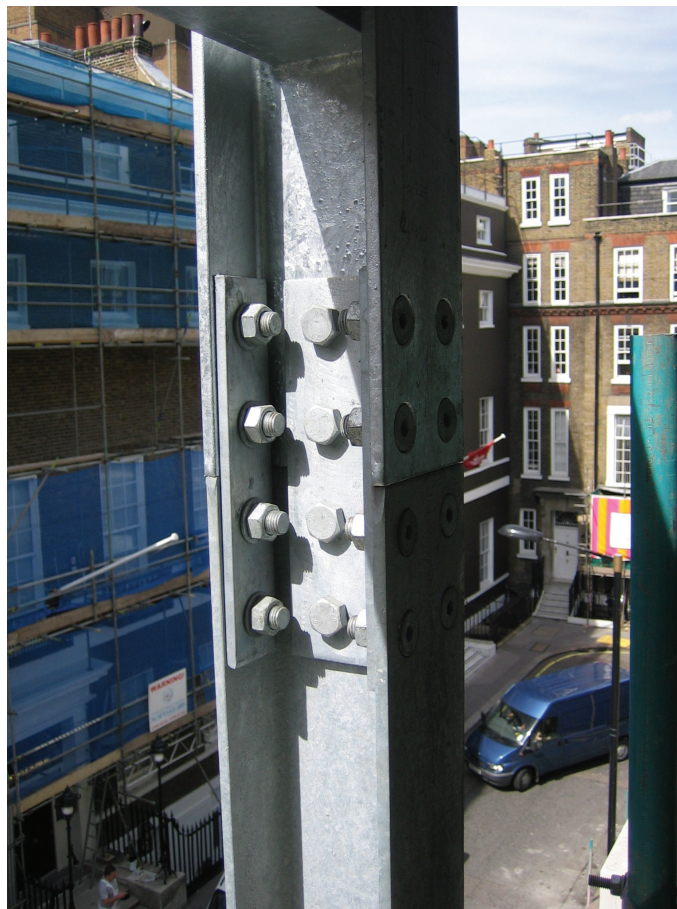
Figure 18.24(b) Compact steel detailing at column splice positions avoids costly change to column casings and ceiling detailing
