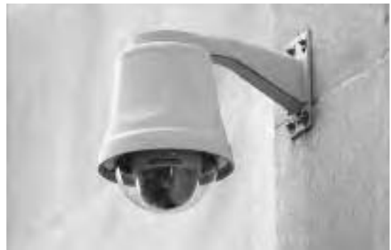
A surveillance camera disguised as a street lamp watches from a street corner in New York City. (SPENCER PLATT/GETTY IMAGES)
