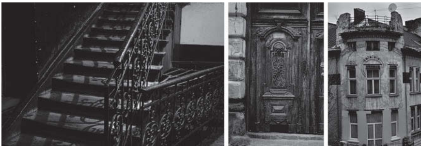
Photo 6.16 Where a lack of cultural significance and of valuation of built heritage persists, original staircases ( left , Majera Balabana St. 29) and ornaments dilapidate, holes may be cut in old wooden doors to let the cats walk in and out ( center , Tomashivs’koho St. 8), and new window frames and satellite dishes are installed ( right , Akademia Bohomol’tsya St. 3)
