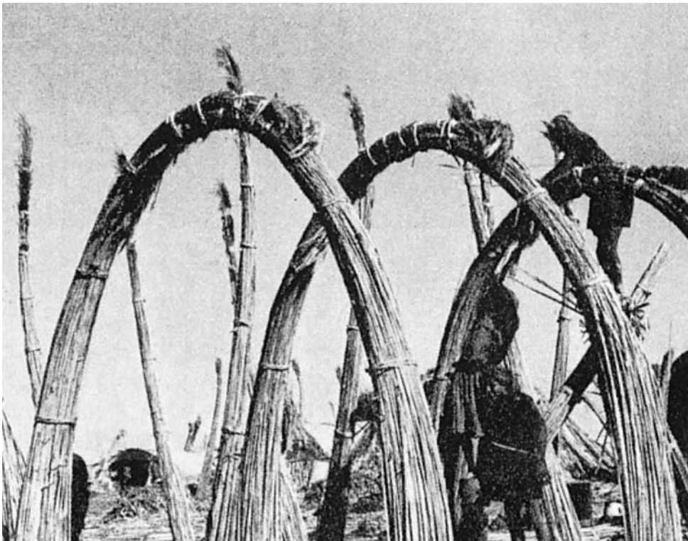
104. The Mudhif. Building Process. Framed construction in bundled reeds of the mudhifs (“guest houses”) of the marsh arabs of Southern Iraq. The cladding is of horizontal “poles” formed from slighter reed bundles which act as ties between the hoop frame, and support sheets of matting. The characteristic (parabolic) curve of the pliant material identifies this type of construction. After Thesiger.
