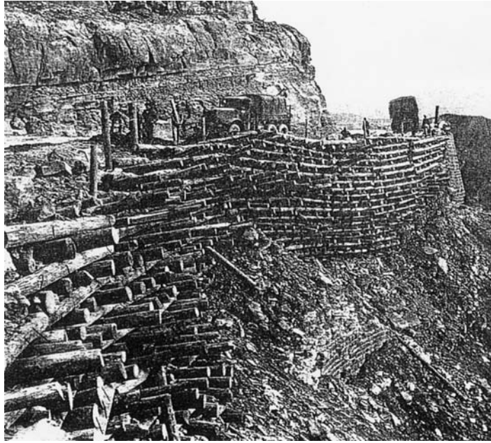
59. Modern Cribbing for Emergency Field Construction Work. To make good a mountain road destroyed by explosives a working platform has been fashioned in the blasted cliff face by laying spaced out logs in courses alternatively set at right angles. This provides a stable and solid support for any building operation, and itself requires nothing beyond human energy to build. After P. Hodges p. 12, fig 12.
